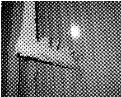
Fig. 6 Deposits on an electrochemical probe in the flue gas path of a CFB boiler after 6 months of co-combustion operation [21]
