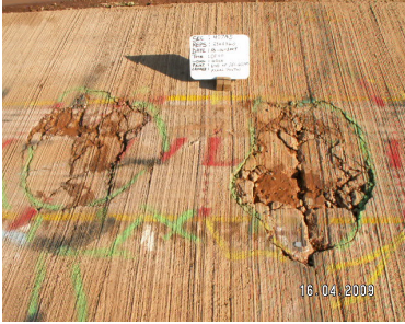
457A5: Failure after 2.235 million reps
