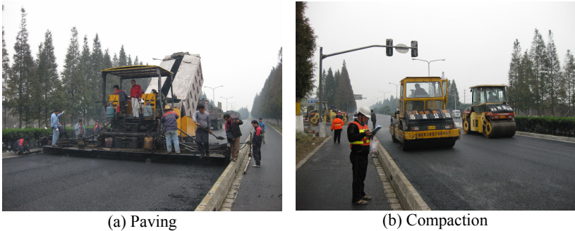
(a) Paving (b) Compaction FIG. 3. Paving and compaction at Huqingping Road project
