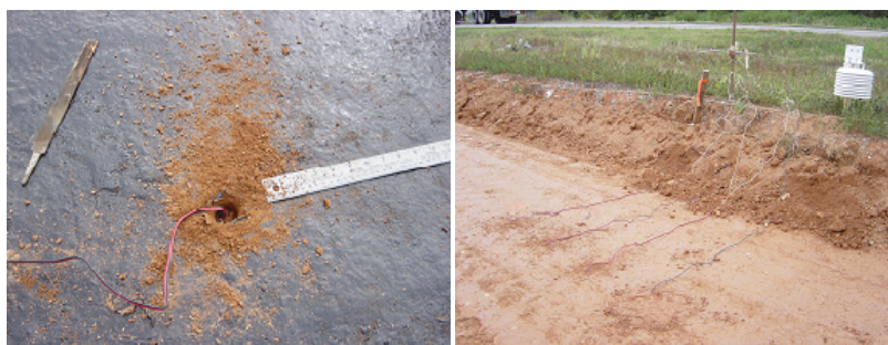
FIG. 1. Individual temperature sensor installation (left) and overall array (right)
