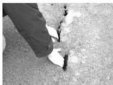
FIG. 11. Longitudinal crack of the surface layer in-situ
