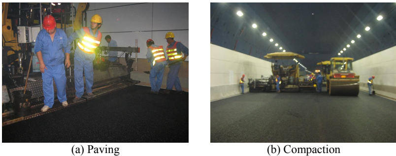
(a) Paving (b) Compaction FIG. 4. Paving and compaction in Yangtze River Tunnel Road project
