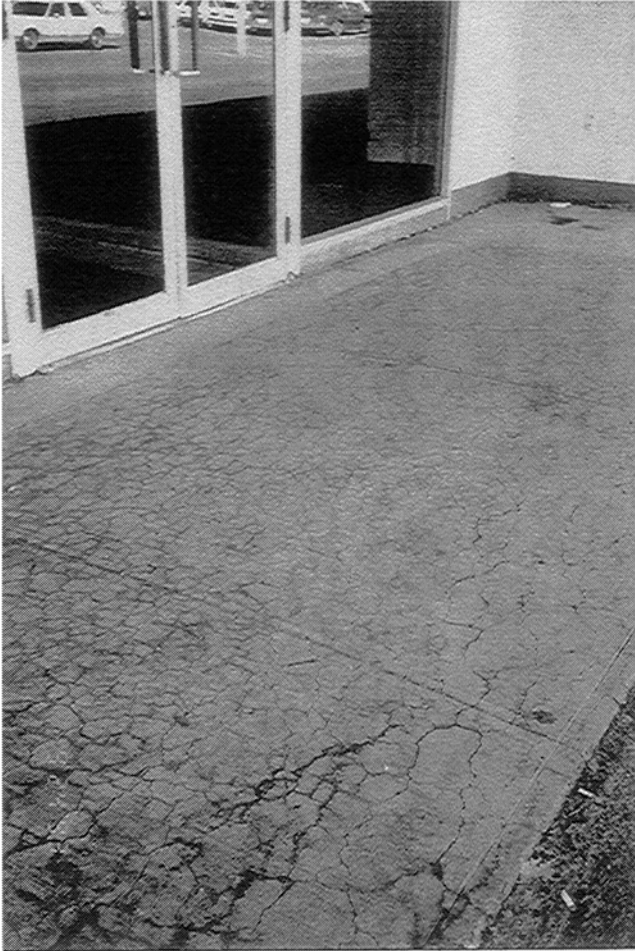
FIGURE 1–14 Cracking in concrete paving caused by an expansive reaction between the aggregate and the alkalis in the cement paste. Source: Hansson, 1995.
