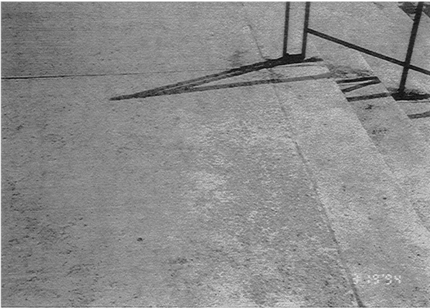
FIGURE 1–13 Salt scaling on concrete steps within six months of being cast caused by the use of deicing salts.
