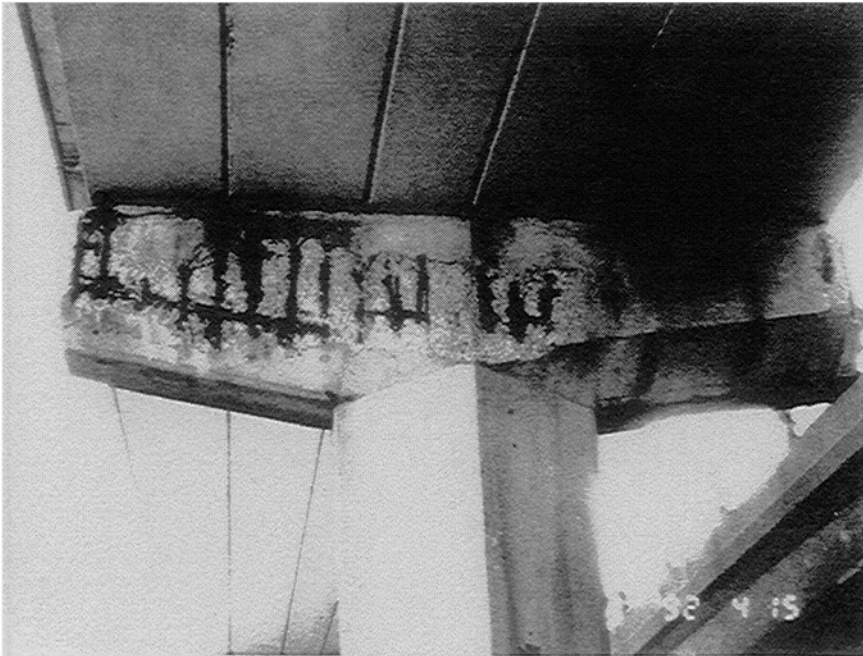
FIGURE 1-11 Corrosion of reinforcing steel in the support structure of an elevated highway caused by deicing salts seeping from the deck. The expansion of the corrosion products has caused spalling of the concrete cover. Source: Hansson, 1995.
