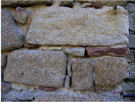
Figure 11.1 Granite ashlars in a building of Giglio island (Tuscany, Italy). Photograph: F. Fratini.
