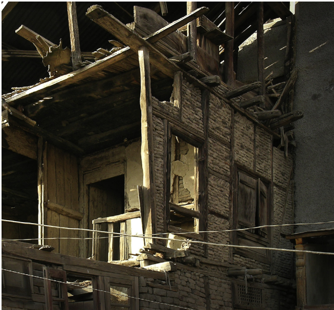
Figure 1.17 Dhajji-dewari building showing the single-leaf construction of the walls. The building was under demolition for a road widening, 2005.
