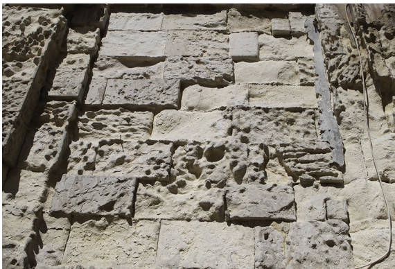
Figure 11.24 Degradation of a calcareous masonry in Ragusa (Italy). Photograph: L. Dipasquale.
