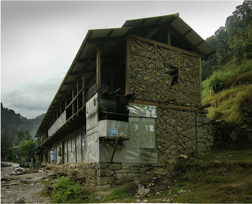
Figure 1.30 Dhajji-dewari building in rural Pakistan, Kashmir, after the 2005 earthquake, showing the few missing wall panels of infill masonry.
