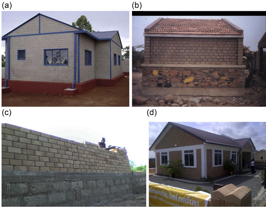
Figure 8.20 CSEB wall and foundation construction. (a) Concrete foundation. (b) Stone masonry foundation. (c) Conventional masonry base with interlocking CSEB superstructure. (d) Foundation and superstructure in CSEBs with higher-strength blocks at base.
