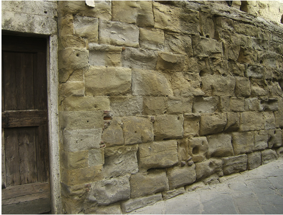
Figure 11.4 “Pietra Bigia” sandstone in a building of Arezzo (Tuscany, Italy). Photograph: F. Fratini.
