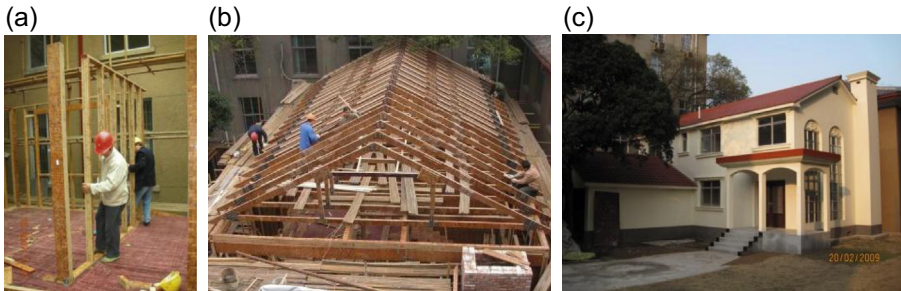
Figure 15.7 Two-story glubam house construction completed in 2008: (a) installing wall frame, (b) roof frame work, and (c) completed glubam house.
