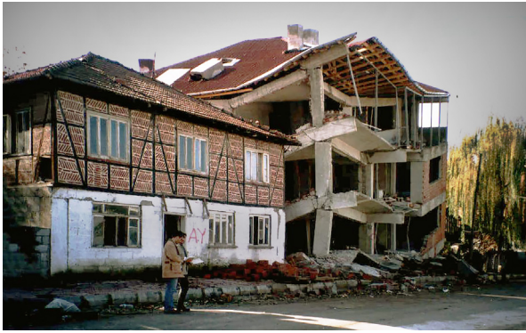
Figure 1.26 View after the 1999 Duzce, Turkey, earthquake showing collapsed reinforced concrete building immediately adjacent to a traditional humuş residence with only one panel of brick infill missing.
