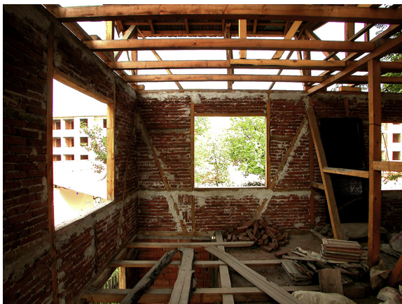
Figure 1.29 The interior of the new house being constructed by this family shown in Figs. 1.27 and 1.28 being built of traditional Turkish humuş construction.
