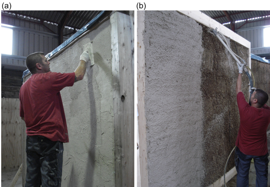
Figure 6.14 Rendering of straw bale wall. (a) Manual finishing off of lime render. (b) Lime render sprayed directly onto surface of the straw bales.
