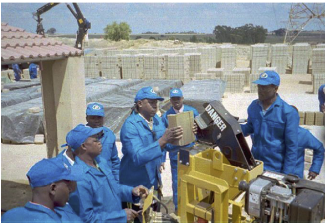
Figure 8.12 Handling and temporary stacking of freshly produced block. African Standards Organisation, 1996. Standards on CEB Construction: Compressed Earth Block Masonry ARS 670: Part 4: Code of Practice for Production and Construction.
