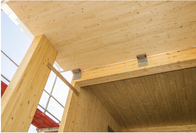
Figure 12.24 CLT construction in Austria similar to that used in the Forté building.
