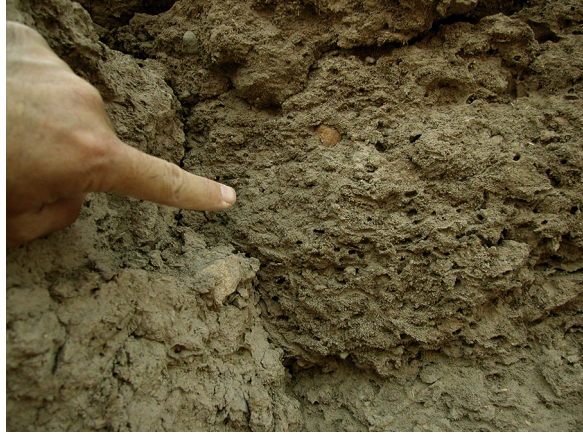
Figure 1.4 Evidence of termites in a wall in the Arg-e-Bam.
