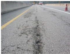
Fig. 6 Distress on bridge deck pavement
