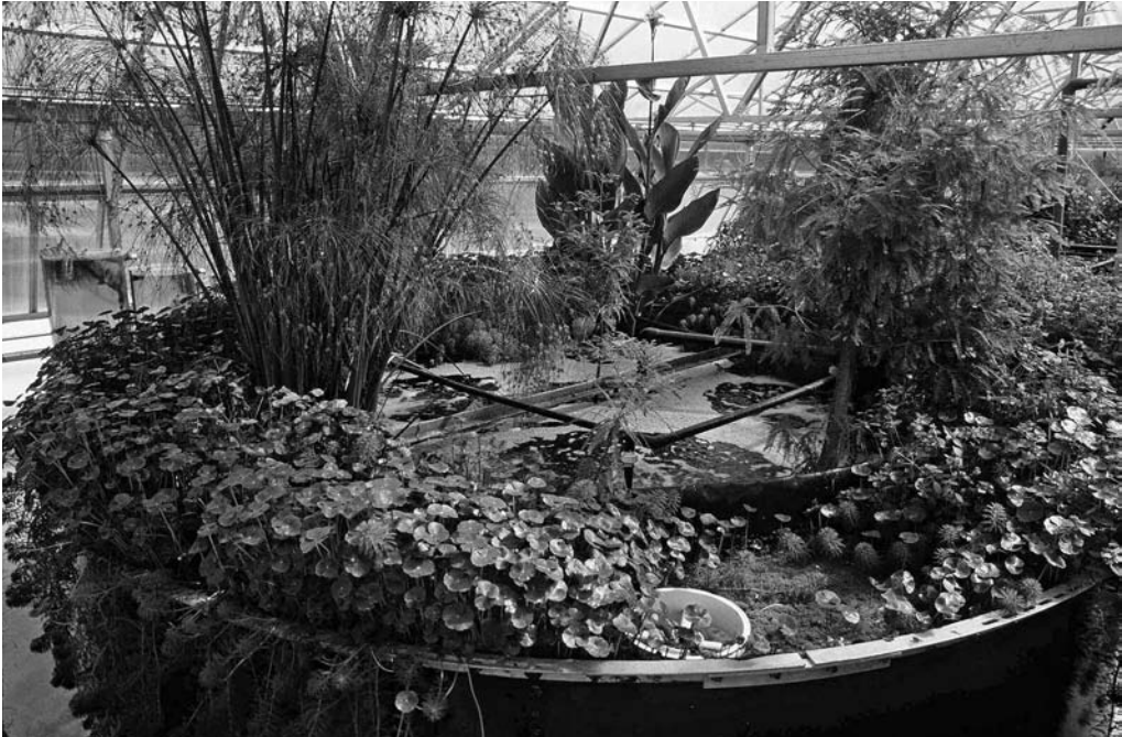
Illustration 18. Known as a “living machine,” this wastewater treatment technology relies on microorganisms and plants to “digest” and “cure” wastewater so that it can be used for other building needs, such as flushing and irrigation.
