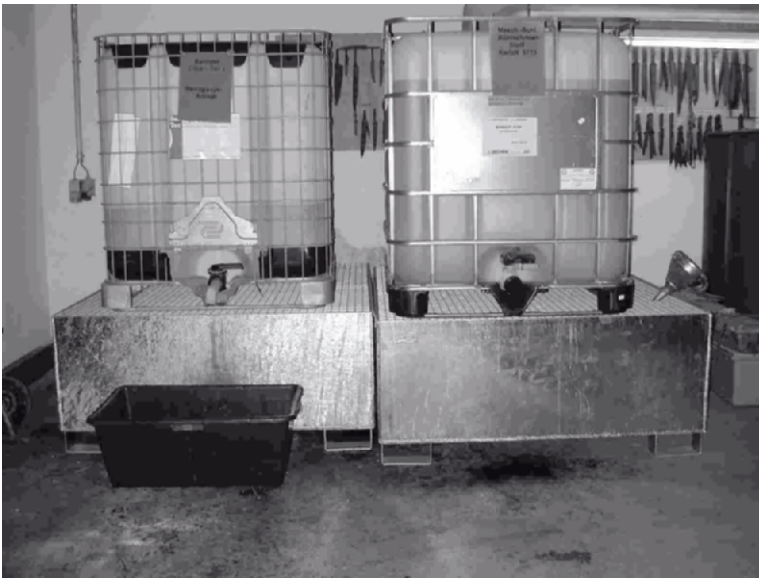
Figure 5. Retention trays for containers with a volume of 1000 l. The tap at the left container is protected by an additional tray to retain small leakages from filling procedures. The whole storage room is constructed as a retention basin and coated with a chemical-proofed coating.
