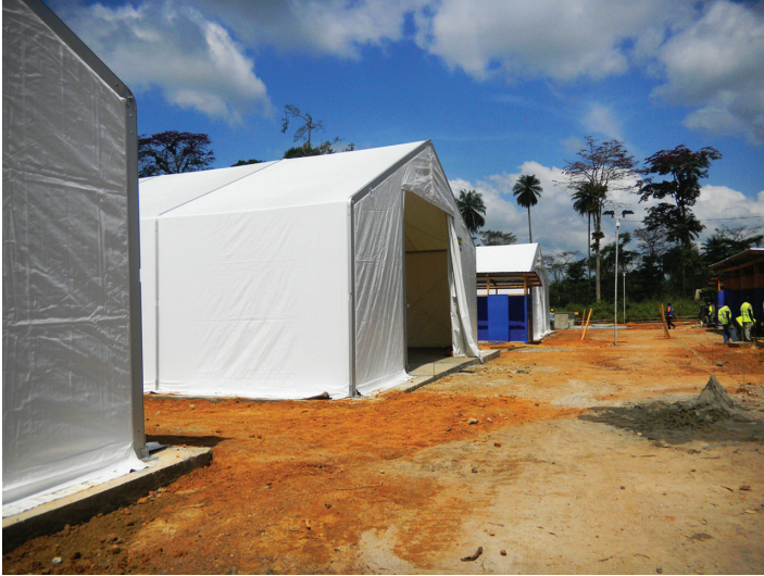
PHOTO 1.2 Treatment center being built in Guinea. (Courtesy of Heidi Soeters, CDC, Atlanta, GA.)
