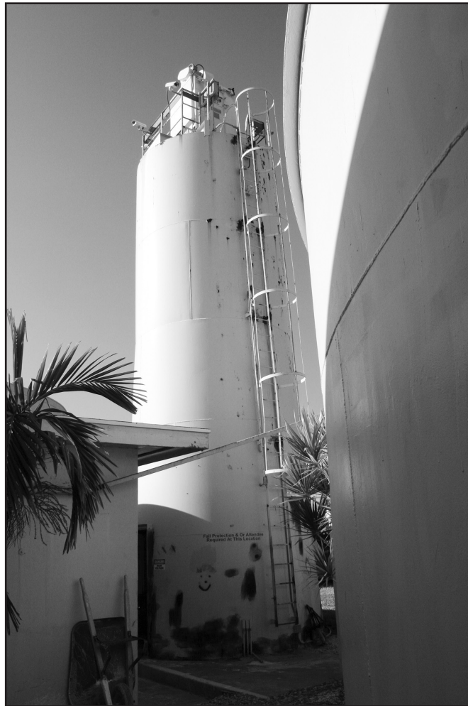
Figure 9-6 Typical silo for dry lime (lime is blown into the silo)
