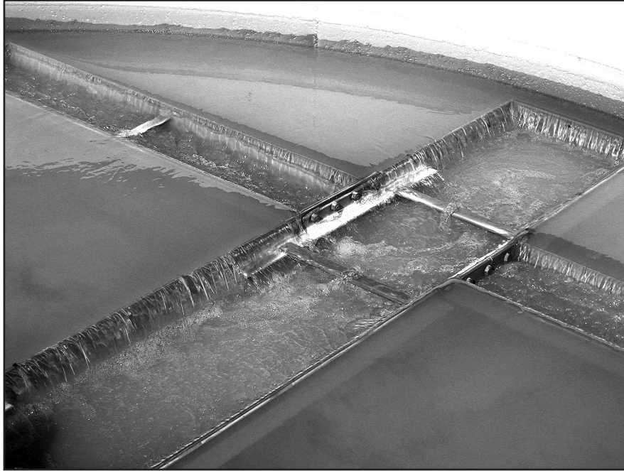
Figure 9-12 Example of filter being backwashed. Backwashing needs to occur regularly but the backwash should be recaptured to improve water use efficiency.
