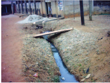
Figure 3.3b. Wastewater in unlined drainage.
