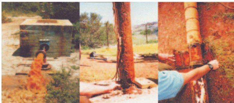
Figure 28.1. Photographs showing the evidence of iron related bacterial clogging at Atlantis in 1991; left, 'red water' is caused by the sloughing of the clogging products inside the borehole; centre, the clogging is encrusted around the submersible pump motor inhibiting effective cooling; right, the pump entry screen is clogged and ultimately the inside of the pump.
