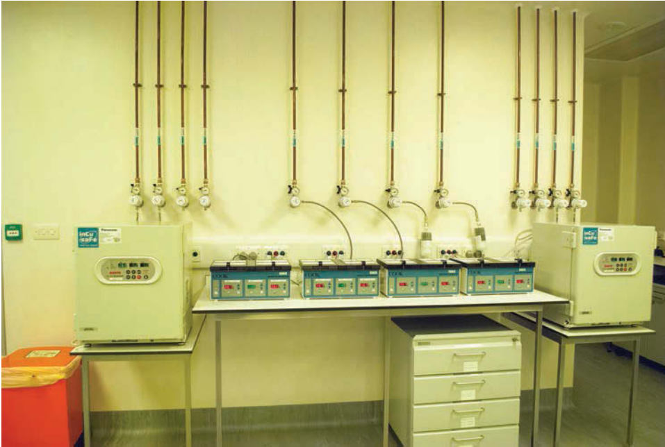
Figure 9.7 Individual gas pipe lines to IVF lab incubators. Each terminal can be connected to an inline filter to remove VOCs from gas bottles. (Courtesy of Magda Carvalho, Cambridge IVF, UK.)
