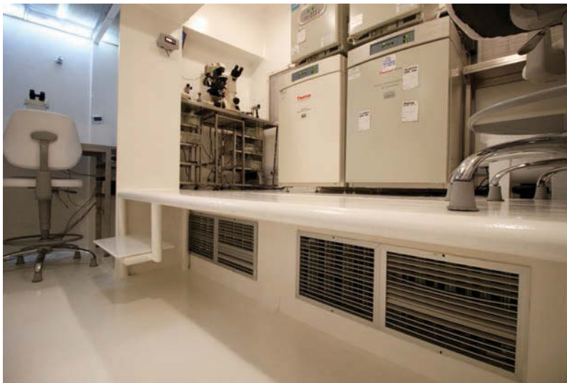
Figure 26.6 Overview of floor level return vents in the embryology laboratory suite.
