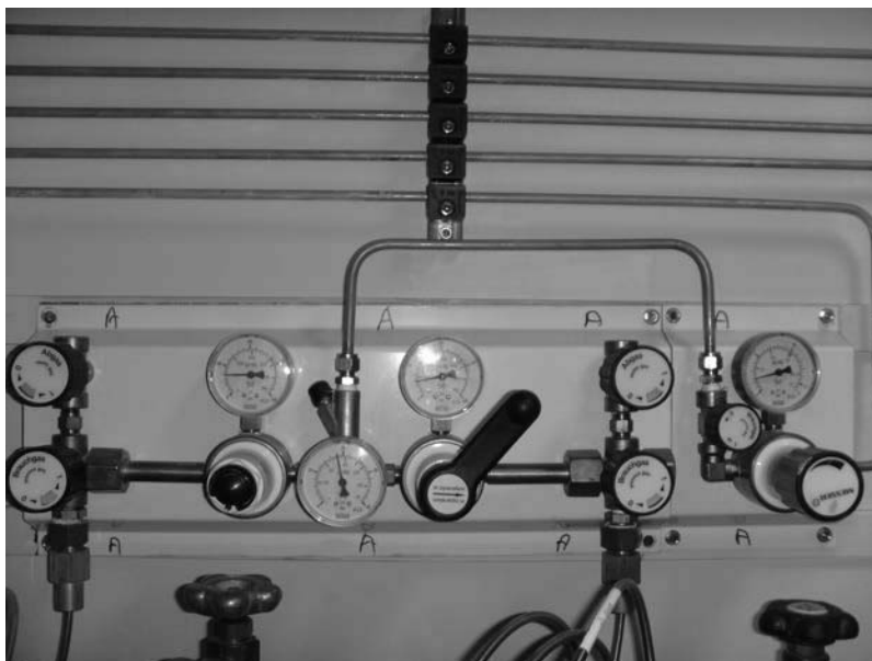
Figure 9.5 Automatic changeover unit connected to a minimum of two cylinders of the same gas. (Courtesy of Giles Palmer, London Womens Clinic, UK.)
