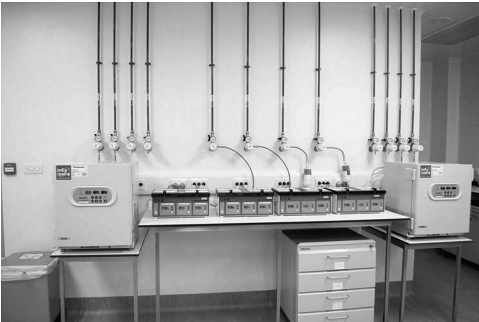
Figure 9.7 (See color insert.) Individual gas pipe lines to IVF lab incubators. Each terminal can be connected to an inline filter to remove VOCs from gas bottles. (Courtesy of Magda Carvalho, Cambridge IVF, UK.)
