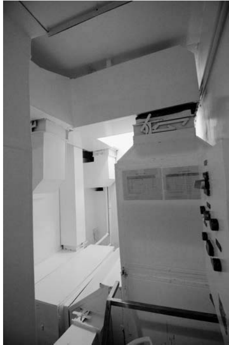
Figure 26.2 Air handling ventilation unit room depicting the free-standing main ventilation unit.
