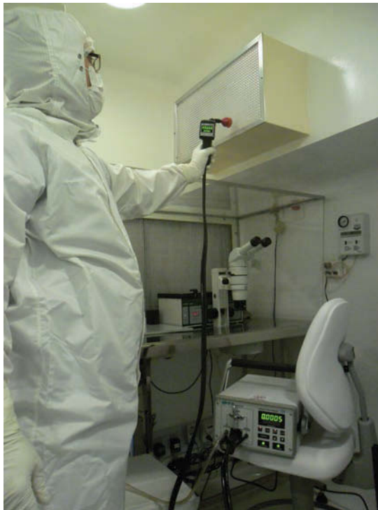
Figure 16.1 In situ testing of HEPA filter installation. Photograph showing an engineer testing a HEPA terminal filter in the clean room IVF laboratory. (Courtesy of Androfert, Campinas, Brazil.)
