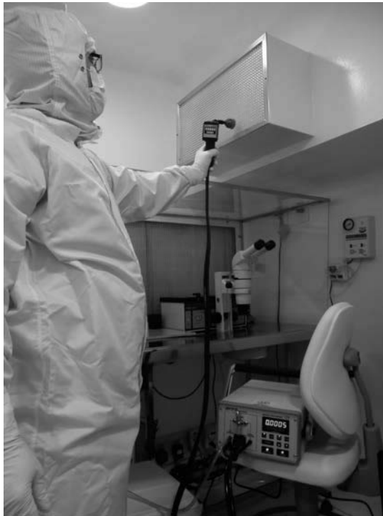
Figure 16.1 (See color insert.) In situ testing of HEPA filter installation. Photograph showing an engineer testing a HEPA terminal filter in the clean room IVF laboratory. (Courtesy of Androfert, Campinas, Brazil.)
