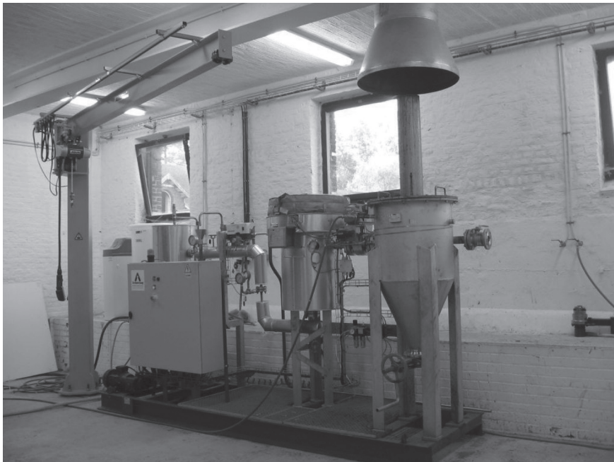
FIGURE 8.15 (a) (see Biorefineries book for redrawing) Steam explosion/vapocracking pretreatment process flow diagram including a steam generator, a reactor, and a burster as developed by Gembloux Agro-Bio Tech, University of Liège. (1) High-pressure pump. (2) Heating collars. (3) Generator pressure and temperature probes. (4) Reactor pressure and temperature probes. (5) Isolation valve. (6) Loading valve. (7) Generator safety valve. (8) Reactor safety valve. (9) Bursting disk. (10) Purge valve. (11) Product recovery valves. (12) Burst manometer. (From Tanahashi, M. et al., Wood Res. , 75, 1, http://ci.nii.ac.jp/els/110000012875.pdf?id=ART0000336908&type=pdf&lang=en&host=cinii&order_no=&ppv_type=0&lang_sw=&no=1310116757&cp= , 1998.) (b) Photograph of the steam explosion/vapocracking equipment at Gembloux Agro-Bio Tech, University of Liège. (Courtesy of Nicolas Jacquet, GxABT, Gembloux, Belgium.)
