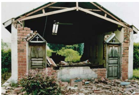
Fig. 233 A church hit by the Fort Portal earthquake of 5 February 1994 in western Uganda.
