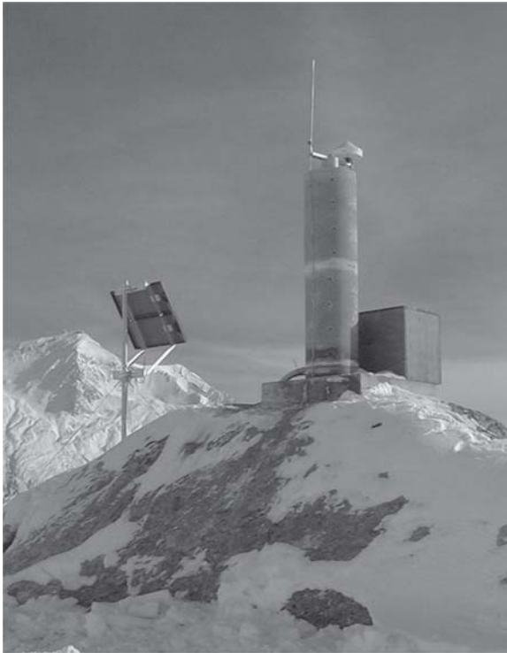
Fig. 7 GPS-receiver on pillar with solar panel energy supply as part of the GOCA array for the monitoring of the Gotthard railway tunnel construction (2002-2014).
