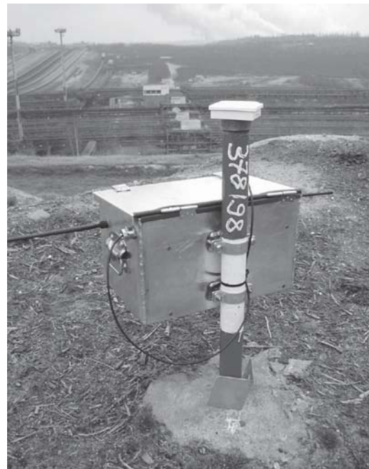
Fig. 2 Example of a GPS receiver and telemetric equipment within a GOCA sensor array in case a slope monitoring in open cast mining at RWE Power AG, Garzweiler using the GOCA system.
