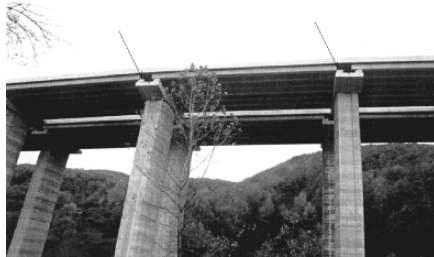
Fig. 14.3. The 1999 Sea of Marmara earthquake. Effects of surface faulting (see the arrows) on the viaduct, near Düzce, part of TEM (Trans-European Motorway). Courtesy of Prof. Polat Gulkan
