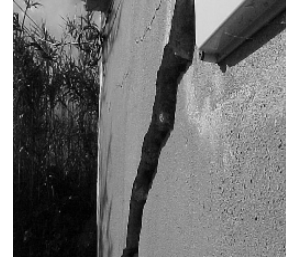
Fig. 19.14. 45° crack in the main façade caused by the displacements of the end wall
