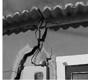
Fig. 19.13. Cracks where the electricity wiretap frame is mounted on the wall
