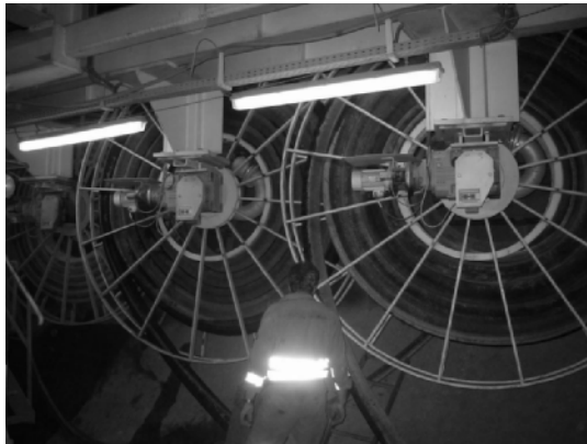
Fig. 12.3. Rolled cables for TBM power supply
