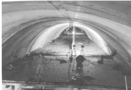
Fig. 2.6. Supply and extract channels above the carriageway. The separating vertical wall has not yet been mounted. 14
