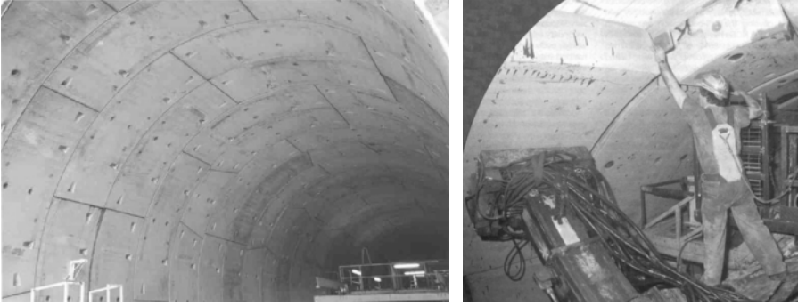
Fig. 4.32. Segmental tunnel lining 30 ; Placing of small discs of wood in the joint
