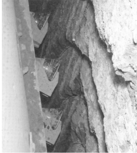
Fig. 4.63. Undercutting at the Uetliberg tunnel 58
