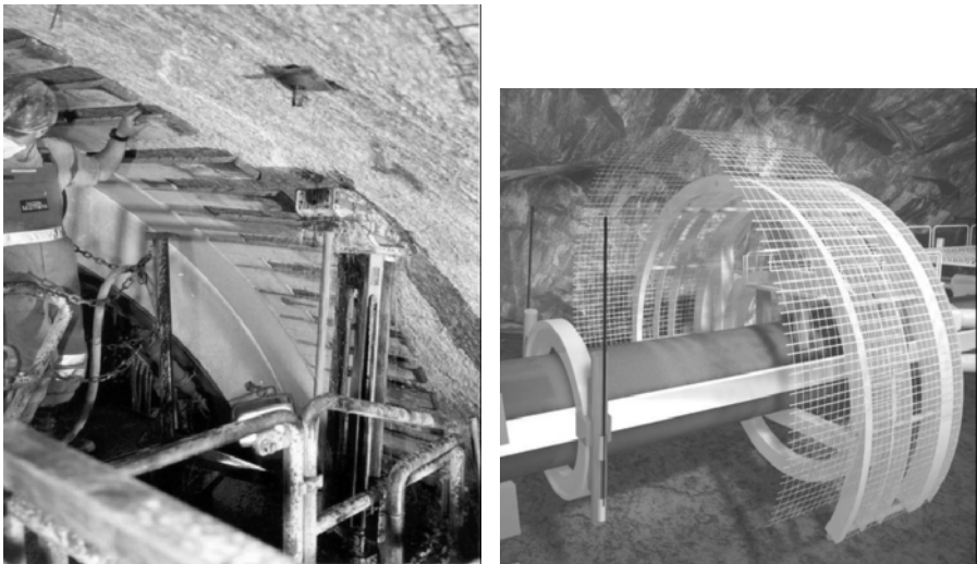
Fig. 4.13. left: Anchoring behind the cutterhead; right: Installation of wire mesh behind the cutterhead 10
