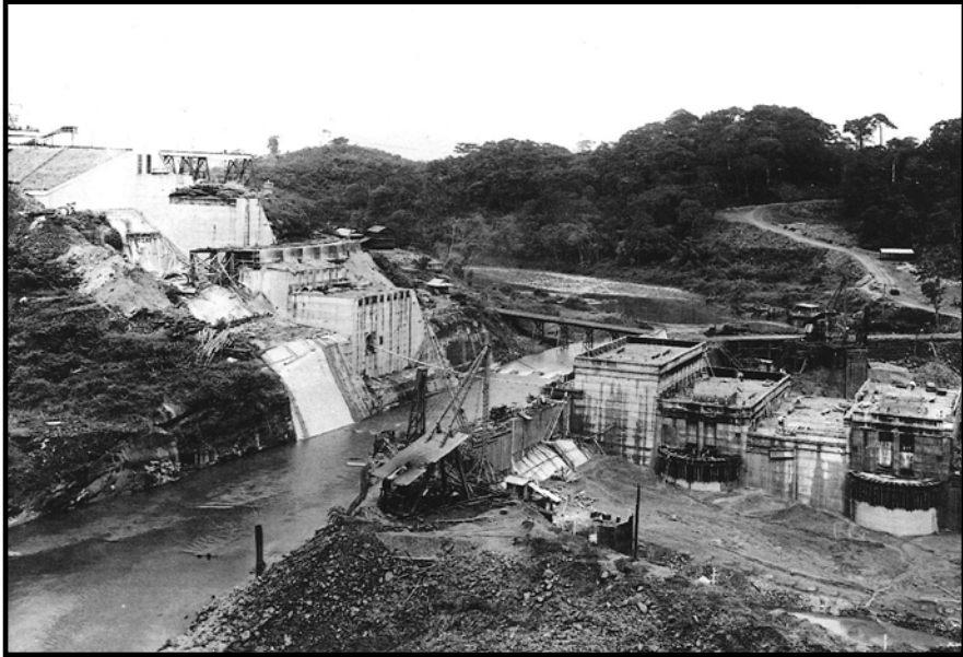
Figure 5. The construction of Madden Dam (1930-1935) across the Río Chagres gave birth to Lago Alhajuela. The dam had three purposes: flood control, storage of water for canal operations during the dry season, and the eneration of electricity for the Canal Zone and canal operations (Panama. Source: Archives, Panama Canal Commission).
