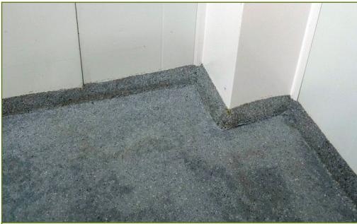
Coated concrete is the correct material for the floors. The design of the join of the floor and wall must be waterproof. It must be easy to keep clean.
