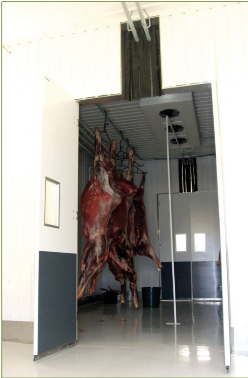
An excellent, airy refrigeration area for carcasses. Condensation from refrigeration machines is collected hygienically into the drain to prevent it from dripping on the carcasses. Note the moisture protection at the bottom of doors.
