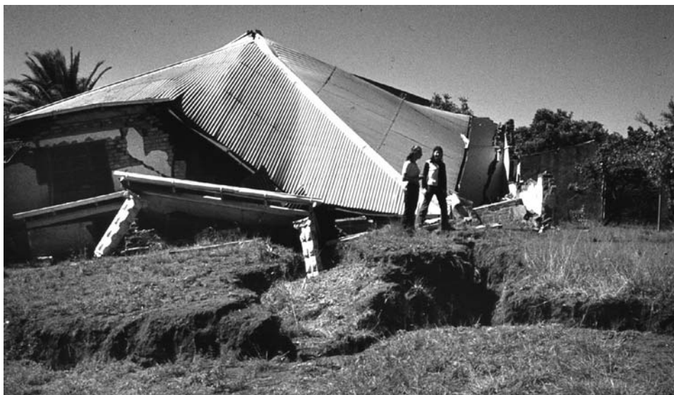
Figure 5.12. A destroyed house within a large compaction sinkhole induced by de-watering the fill in a large and deep buried sinkhole; in the abandoned Bank township in South Africa's Rand karst.
