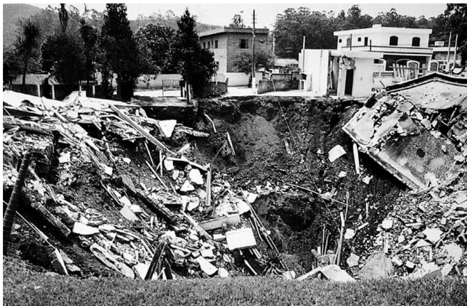
Figure 8.7. Collapse of a house in Cajamar, Brazil, in 1986 over a sinkhole induced in a thick soil cover by excessive groundwater abstraction at a nearby industrial site.
