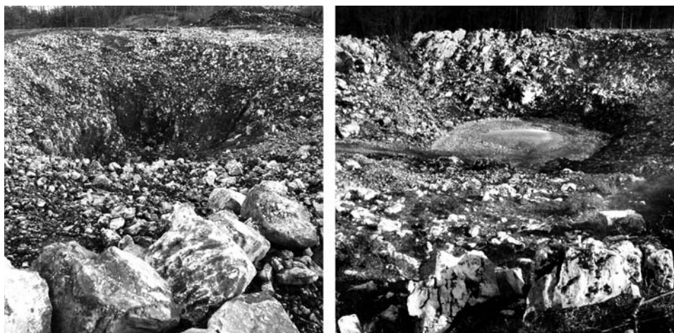
Figure 12.5. Solution sinkholes exposed during construction along a highway footprint in Slovenia, one cleaned out ready for filling, the other with a concrete plug forming its floor. Photos: John Gunn.
