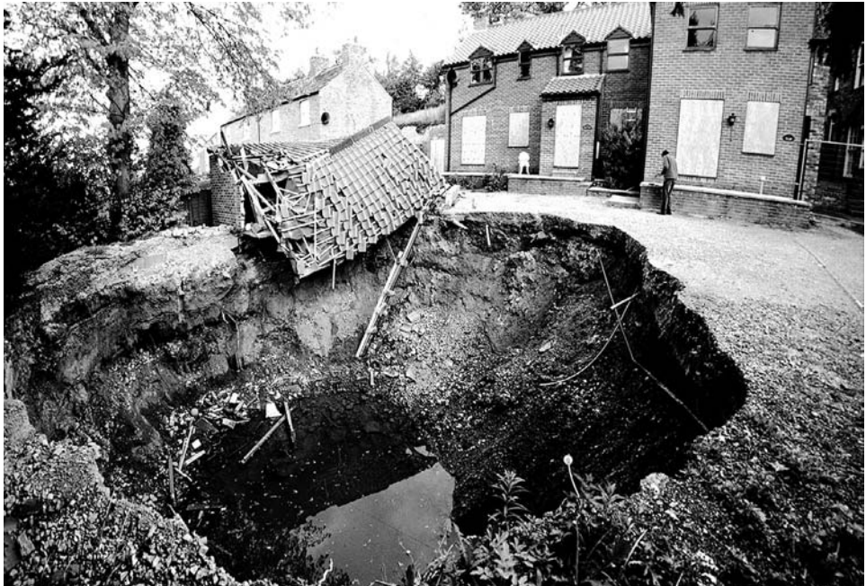
Figure 13.1.1. The open sinkhole that collapsed in front of the house on Ure Bank Terrace, Ripon. TW.
