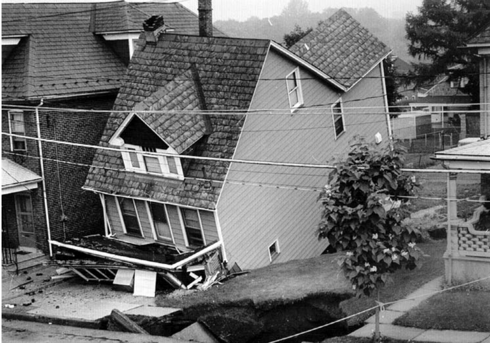
Figure 8.3. Terminal damage to a timber-frame house in Phillipsburg, New Jersey, caused when sinkholes developed underneath it and under the sidewalk after a water main burst beneath the street.
