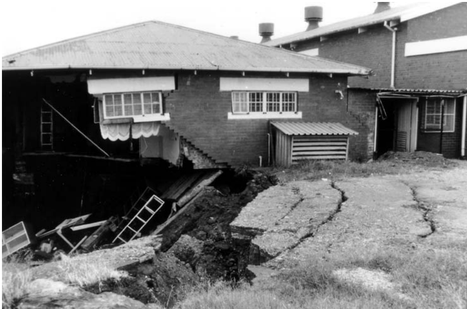
Figure 2.11. A house in Centurion, South Africa, destroyed by development of a large subsidence sinkhole when the soil beneath its foundations was washed into the dewatered underlying limestone.
