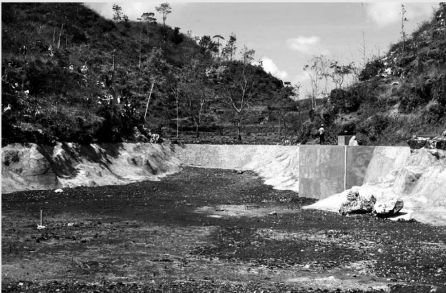
Figure 2.1.2. The Puleirang doline as modified in 1982, with its mortar-sealed slopes, graded clay floor and the concrete dam around the open sink. TW.
