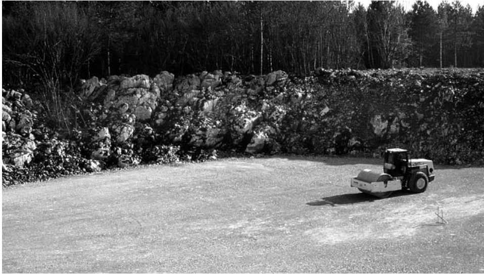
Figure 13.3.3. Compacting a graded fill placed inside a large sinkhole that had previously been filled with loose soil, near Divača.
