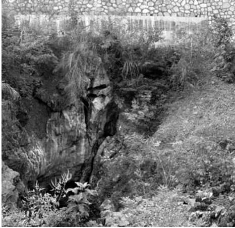
Figure 13.5.6. A concrete slab spanning wide and deep fissures in exposed limestone, with hand-placed stone facing on the road embankment above. Photo: Mingtang Lei.
