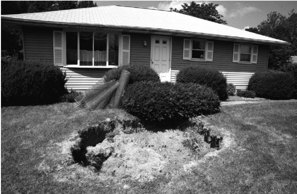
Figure 4.8. A dropout sinkhole in the front lawn of a house in Pennsylvania; the hole was originally 5 m deep but was filled with soil to prevent the sides flaring out, and the soil fill had compacted and settled by 0.7 m by the time this photo was taken. TW.
