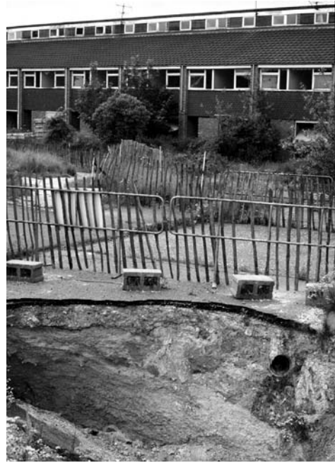
Figure 3.17. One of the collapse sinkholes formed by liquefaction failure of the chalk over old mines in Bury St. Edmunds, U.K., seven years after their failure destroyed the road. TW.
