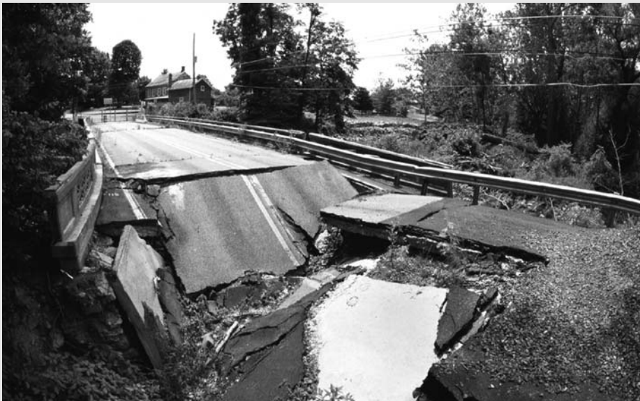
Figure 8.2.2. The bridge that carried Tatamy Road over Bushkill Creek, destroyed by an expanding and ever-changing cluster of sinkholes. TW.
