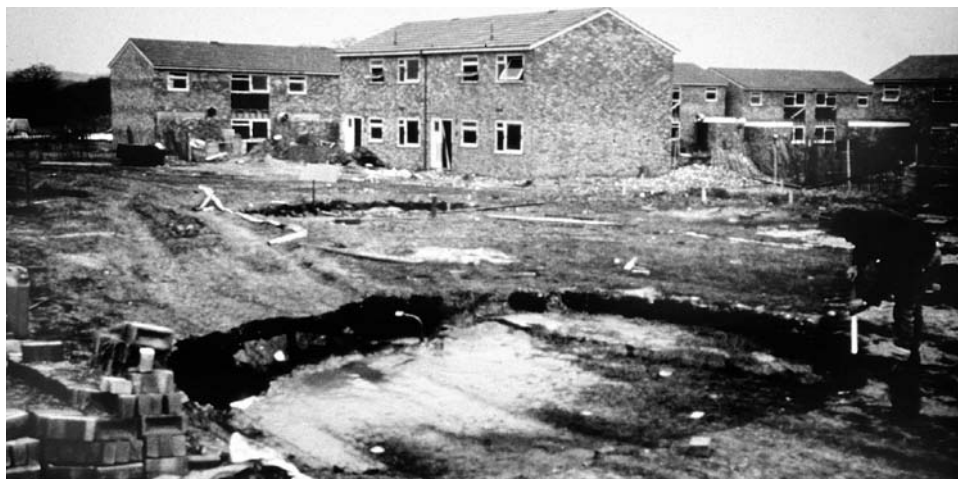
Figure 5.15. Subsidence of about 300 mm over a chalk pipe whose fill was disturbed by construction activity on a site in the English Chiltern Hills.
