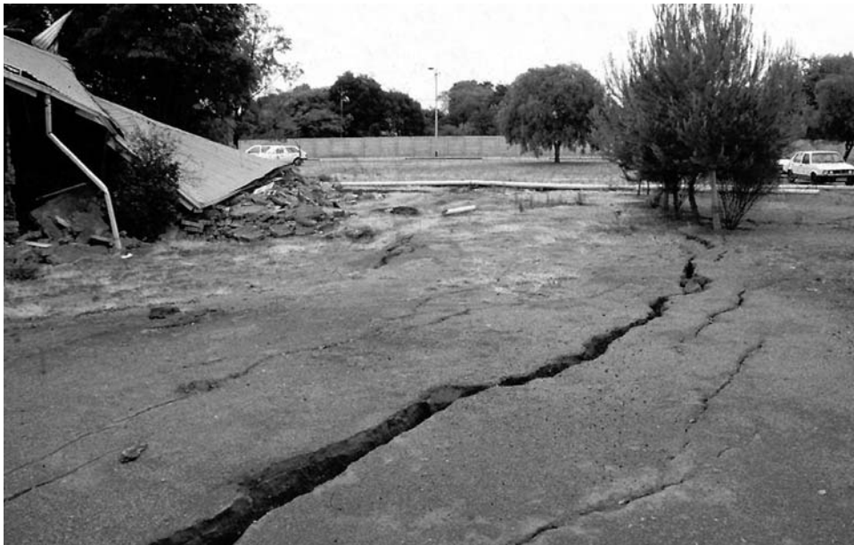
Figure 13.12.2. Ground fissures around the subsidence feature adjacent to the northern end of the Centurion warehouse after it finally collapsed in November 1994.
