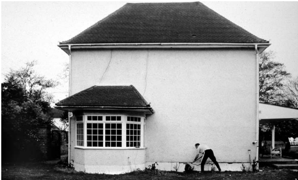
Figure 13.8.2. The west end of the house extension, showing the new open break where the floor has dropped away from the wall, and also cracks in the higher part of the wall where it is failing in cantilever.
