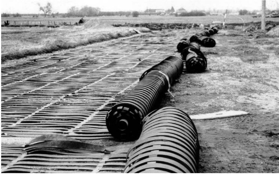
Figure 12.7. Heavy paralink geogrid being rolled out onto a road sub-base as a protection measure against sinkhole development in the underlying soil. TW.
