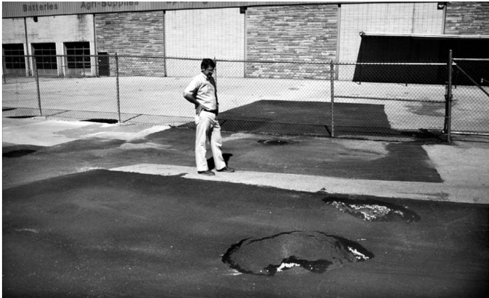
Figure 11.4. A small sinkhole that has been repeatedly filled, without proper treatment, under a much-patched parking lot in Bowling Green, Kentucky. TW.
