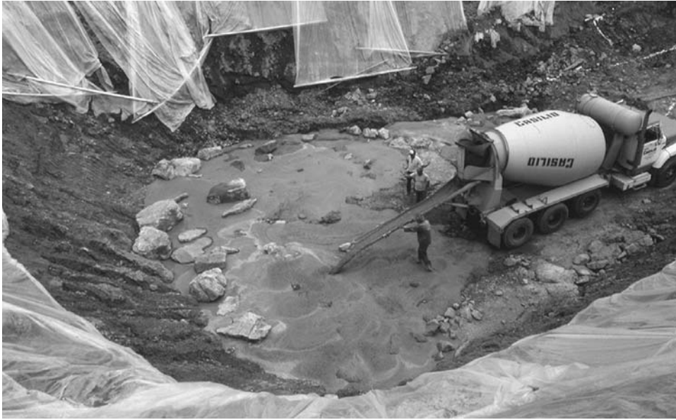
Figure 11.10. Pouring the last of the concrete into the plug of chunk rock in the Macungie sinkhole, before rebar was laid as reinforcement to a cast concrete cap.
