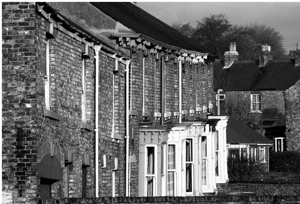
Figure 2.9. A terrace of houses in Ripon, U.K., subsided due to a combination of rockhead dissolution of gypsum and compaction of soft sediments filling an old buried solution doline. TW.
