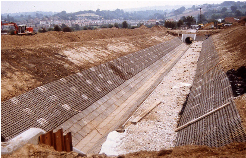
Figure 7.20 Lined vee ditches.
