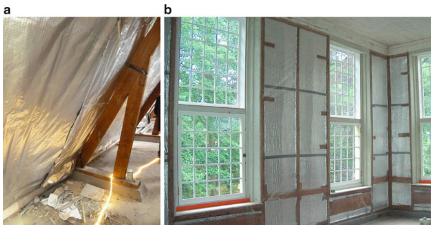
Fig. 7.34 The application of vapor barriers is an import but sometimes difficult job: (a) a vapor barrier with very small overlap and weakly glued seams, this can become problematic in future and needs adjustment (Photo: Van der Wal, Cultural Heritage Agency of the Netherlands), (b) a properly executed vapor barrier with a sufficient overlap and properly glued seams as part of a wall closing protocol
