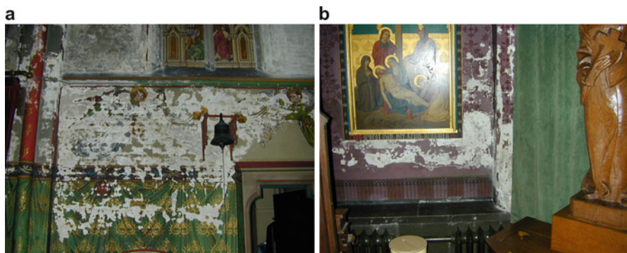
Fig. 5.3 Salt efflorescence near the surface of a catholic church in the Netherlands severely damaging the wall painting (a) and a common cause the heating system (b) near the surface causing high temperatures and low relative humidity
