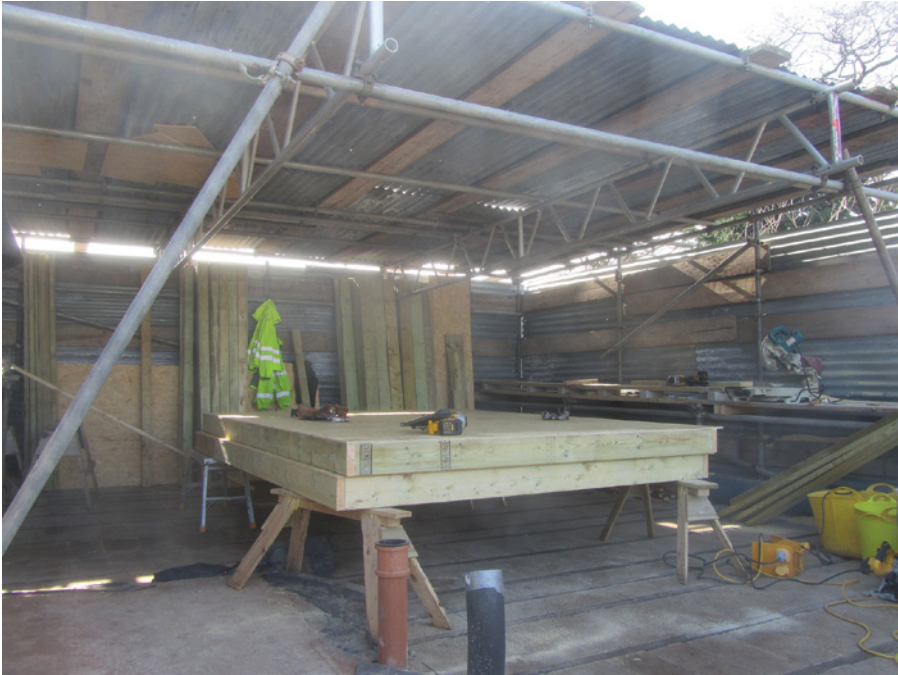
On site panel fabrication area- scaffold framed temporary building with open front
