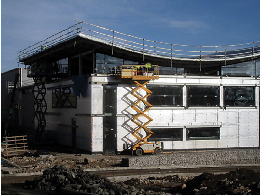
Cladding to office block elevation in progress, stone gabions to form wall feature to front face of office block and returns
