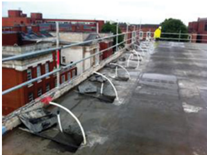
Anchorage points on surface slab. Anchorage consists of iron casting and wedge system which grips the wire strand
