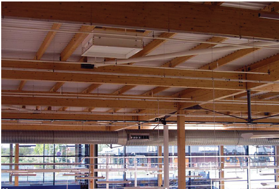
General view of laminated timber roof supported on 250 x 250 mm timber columns
