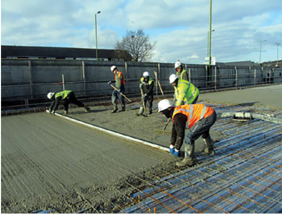
Screeding surface of slab with metal screed board. Tolerances +/- or - 10 mm. Tarmac surface to be laid over finished concrete
