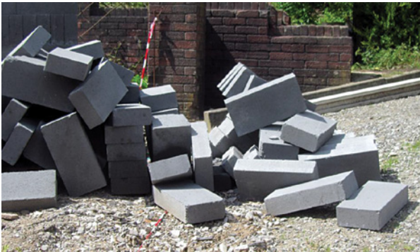
Block stacks inadequately banded – as the bands are removed the blocks are allowed to fall over
