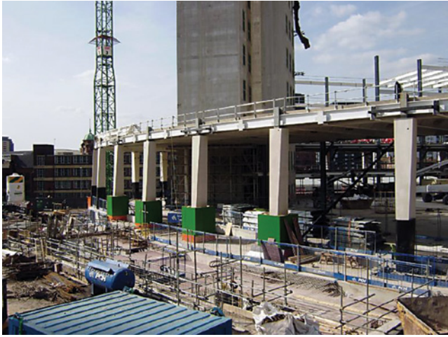
Pre-cast columns on building façade and 2 nd floor steelwork and floors completed
