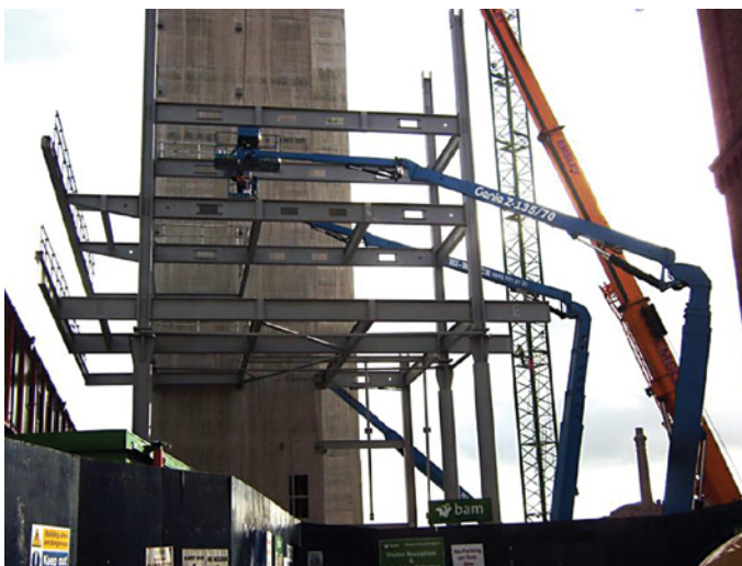
Telescopic mobile crane and hydraulic lifters(Genia Z type) in action, Erecting the steel frame around the staircase cores
