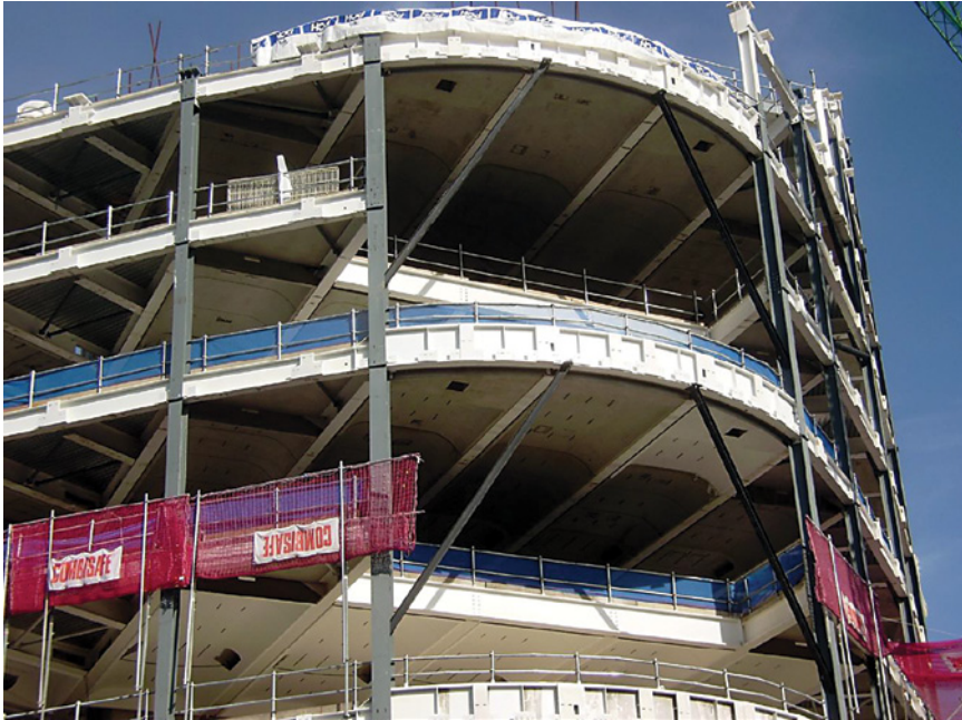
Precast coffered floors at levels 6 to 8. Steelwork in progress to elevated level at rear of building (floors 9 & 10)
