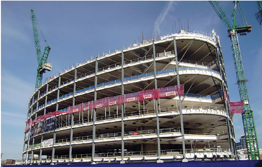
The steelwork and precast coffered floors were erected over a 6 week period (June/July 2011). Work commenced to the services fit out to the lower ground floors
