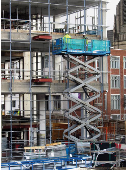
Handling and fixing of support frame and glazed wall panels from hydraulic scissor lift
