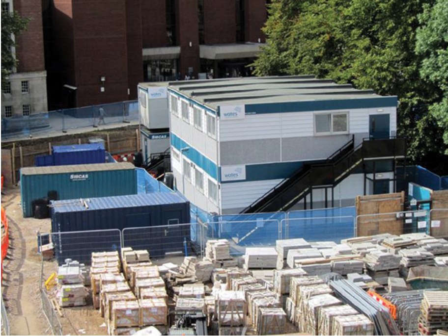
Site office compound area – initial storage area for paving products in front of rear building extension
