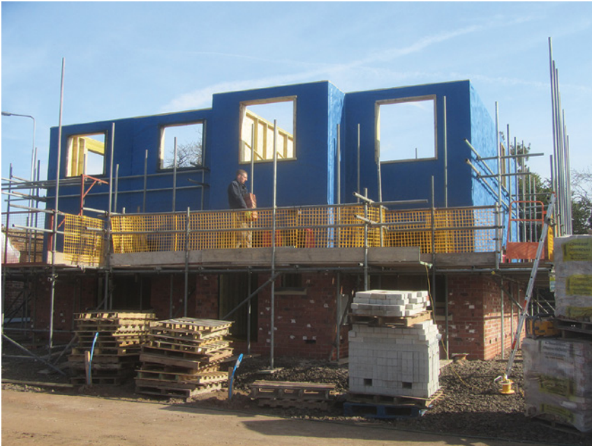
Front and side elevation panels to upper floor in position. Upper floor panels to house units 1 and 2 erected within a one day period (two joiners and one labourer)
