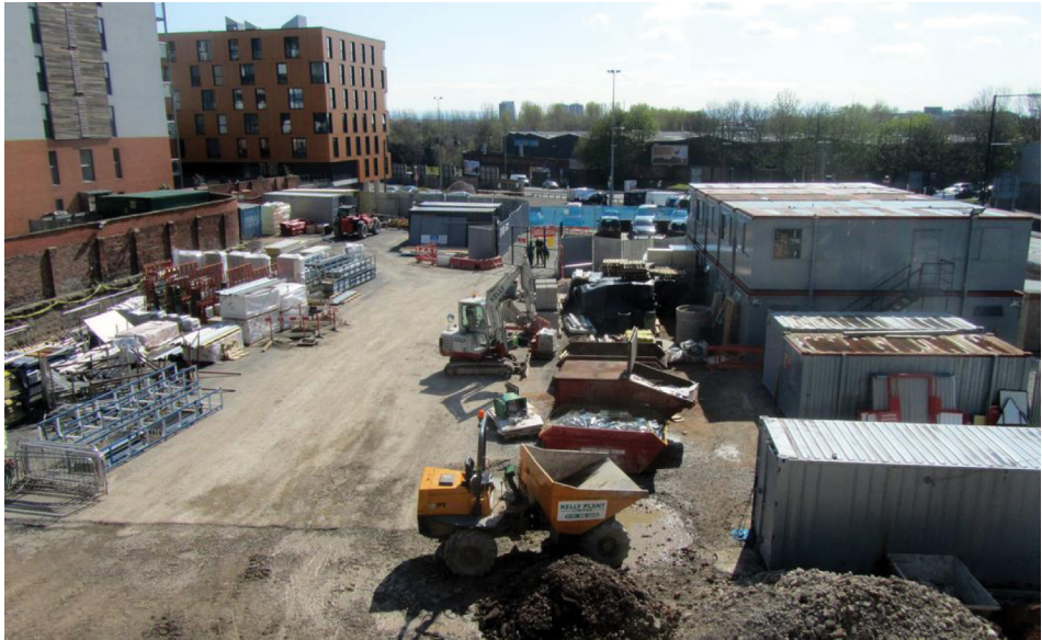
Extensive site compound and storage areas – central areas for vehicles moving materials to the building area
