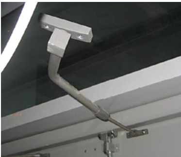
Snagging item: door stay requires refixing to frame
