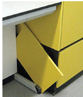
Incomplete work: refix panel at side of unit
