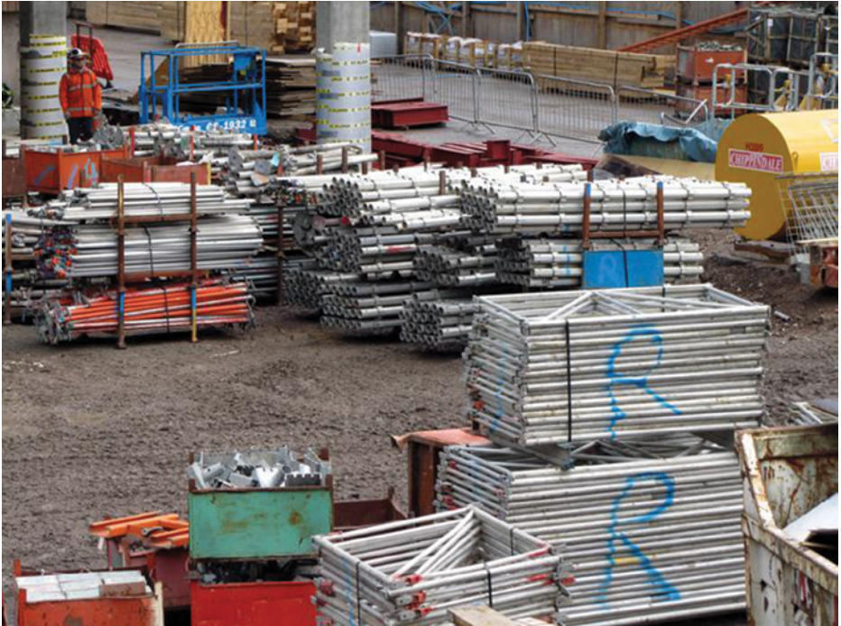
Disbanded formwork support being banded and placed on storage racks prior to removal from site
