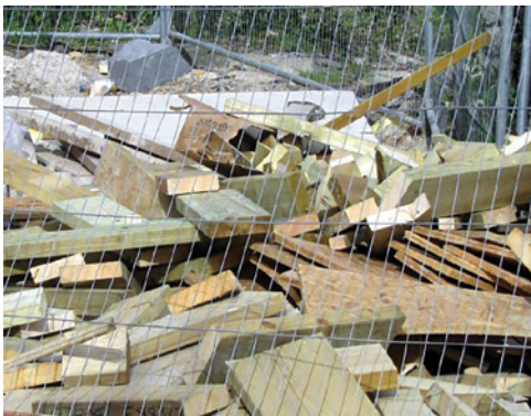
Timber off-cuts from roof purlins and rafters – mass waste of treated timber (this could have been easily deposited in large bags for disposal)
