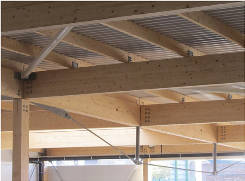
Metal base plates and column connections to all laminated columns and roof beams. This enables the speedy erection of the main timber frame
