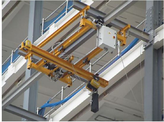
Single track mono-rail in position for handling glazed storey height panels to rear of building
