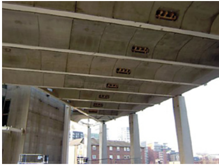
Services provision along underside of floor units
