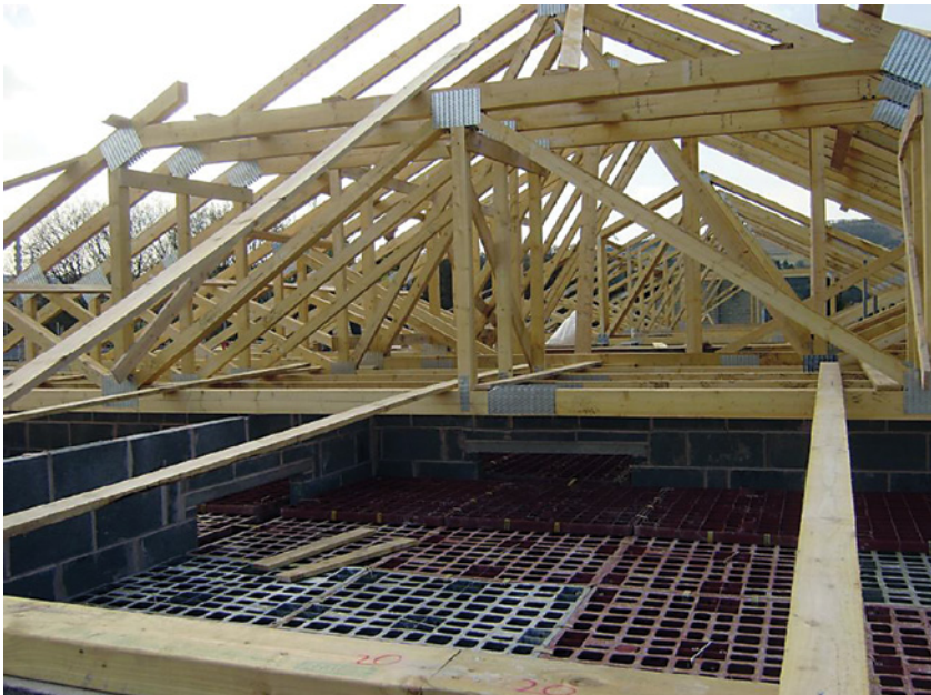
Internal bracing to 10 m span roof trusses. Safety Deck shown for access to underside of trusses
