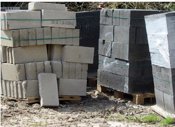
The subcontractor cannot be held fully responsible as a prepared area for storage of materials was not provided by the speculative contractor.
