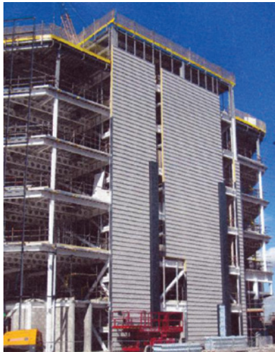
Rear view with external cladding in progress – plant room completed at roof level
