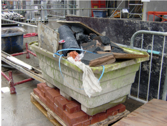
Use of waste containers for handling mixed materials – in this case a mortar skip
