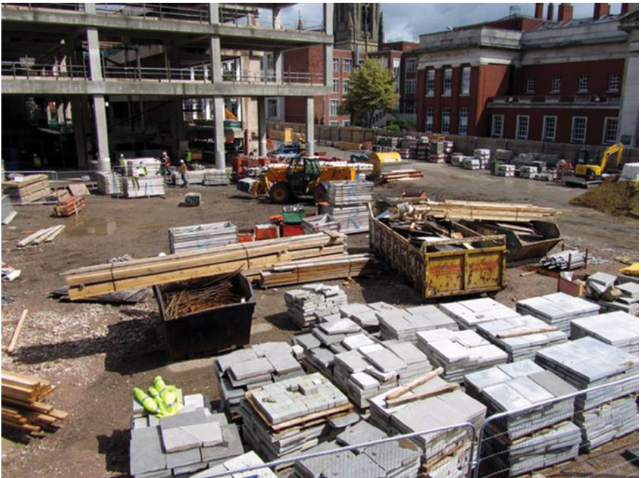
Soffit timber being de-nailed and re-banded for transfer to another site. Loose timber skips for waste material
