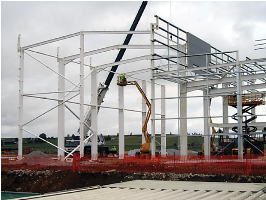
Commencement of the erection of the nine bay high level portal frame
