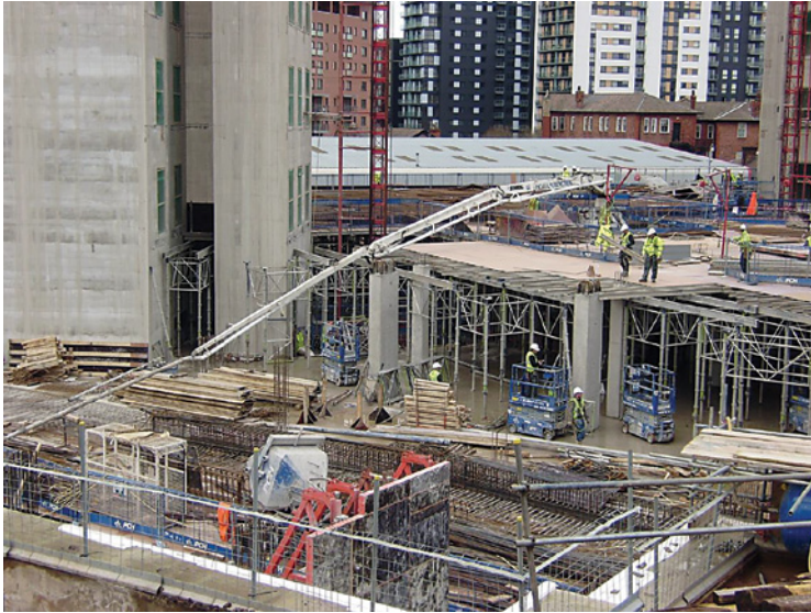
Mast pump located at ground floor level (placing concrete in the basement area)
