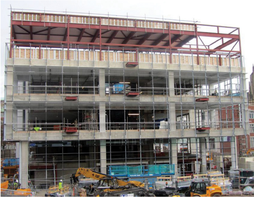
Rear elevation of building with aluminium curtain walling support in position to receive glazed panels
