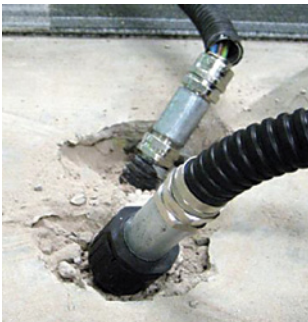
Snagging item: make good around connections, prior to tiling
