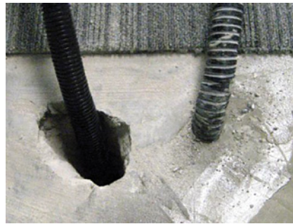
Snagging item: wrong position of service holes in floor – sleeve and make good around opening
