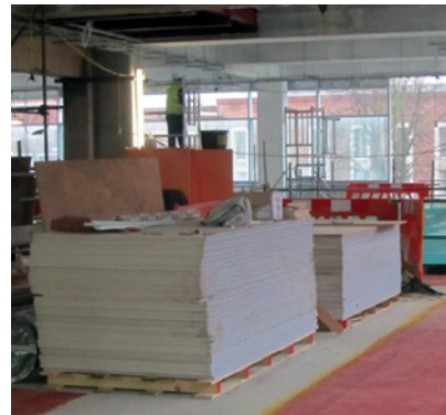
Cleared areas at each floor level for storage of internal wall lining materials
