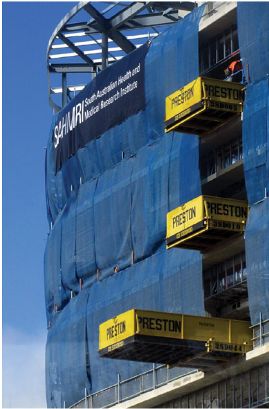
Extensive use of projecting storage skips (conti boxes) on the facade of a building – the conti boxes can be used for storage of components positioned by tower crane or other mobile cranes
