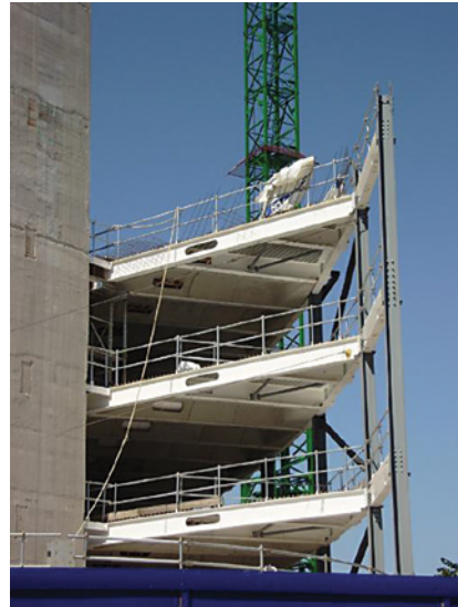
Precast coffered floor units positioned with tower crane working up from floor 3 to 5
