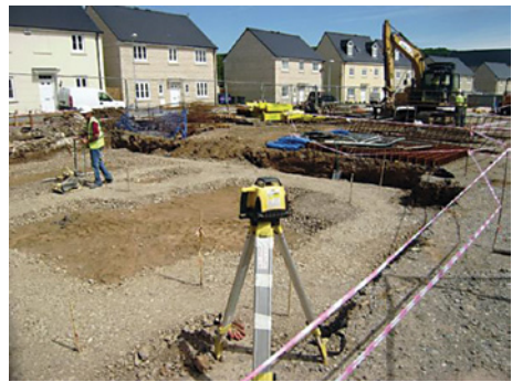
Foreman checking level of foundation concrete/ checking compact stone fill levels using the laser level
