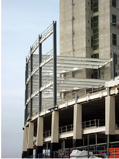
As the precast floors are completed work can commence to internal walls and service installation on the lower floors
