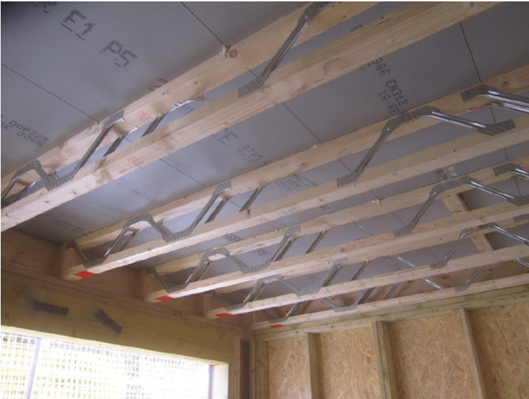
Underside of floor panels to first floor – IJ beams at centres incorporated in floor construction
