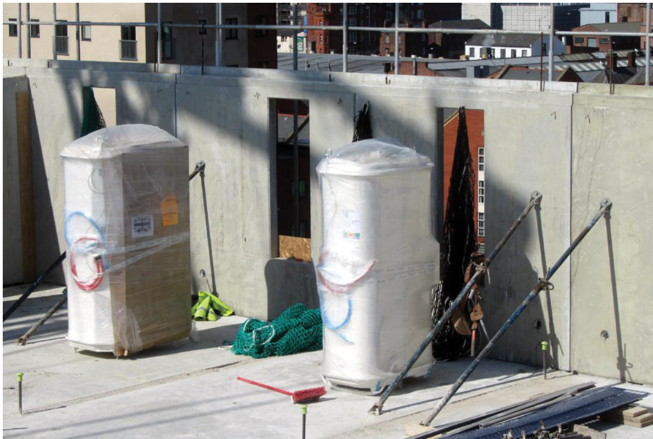
Bathroom shower cassettes lifted into rooms as work progresses – temporary propping support shown to external wall panels
