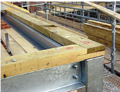
225 mm x 75mm Softwood timber wall plates bolted to steelwork or fixed to top of brickwork
