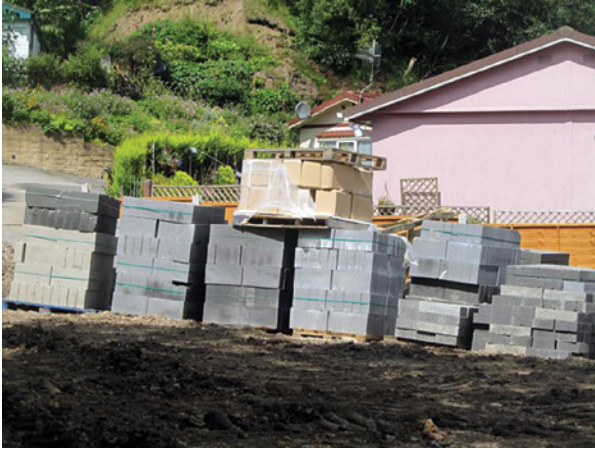
Complete lack of site preparation prior to the delivery of site materials – blocks delivered and placed on uneven ground (on pallets)
