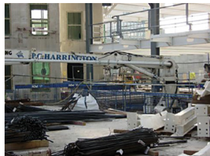
Position of mast pump in centre of project
