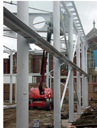
Single-storey castilated roof beams – erected by mobile crane and hydraulic lifters (cherry pickers)
