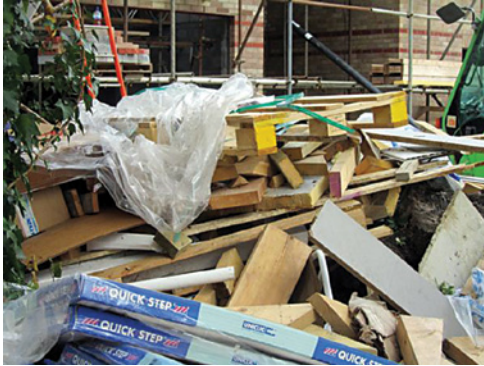
Mixed materials stockpile – packaging, pallets, timber off-cuts, plasterboard, insulation – why not put it in a skip?
