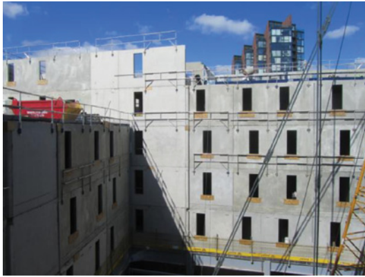
Progress at fifth floor of crosswall frame – note the handrail fitted to the top edge of the external wall units
