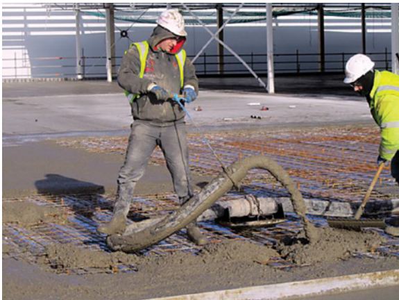
Flexible delivery hose at discharge end of pipe line. 10 labourers engaged on placing reinforcement and laying concrete slab
