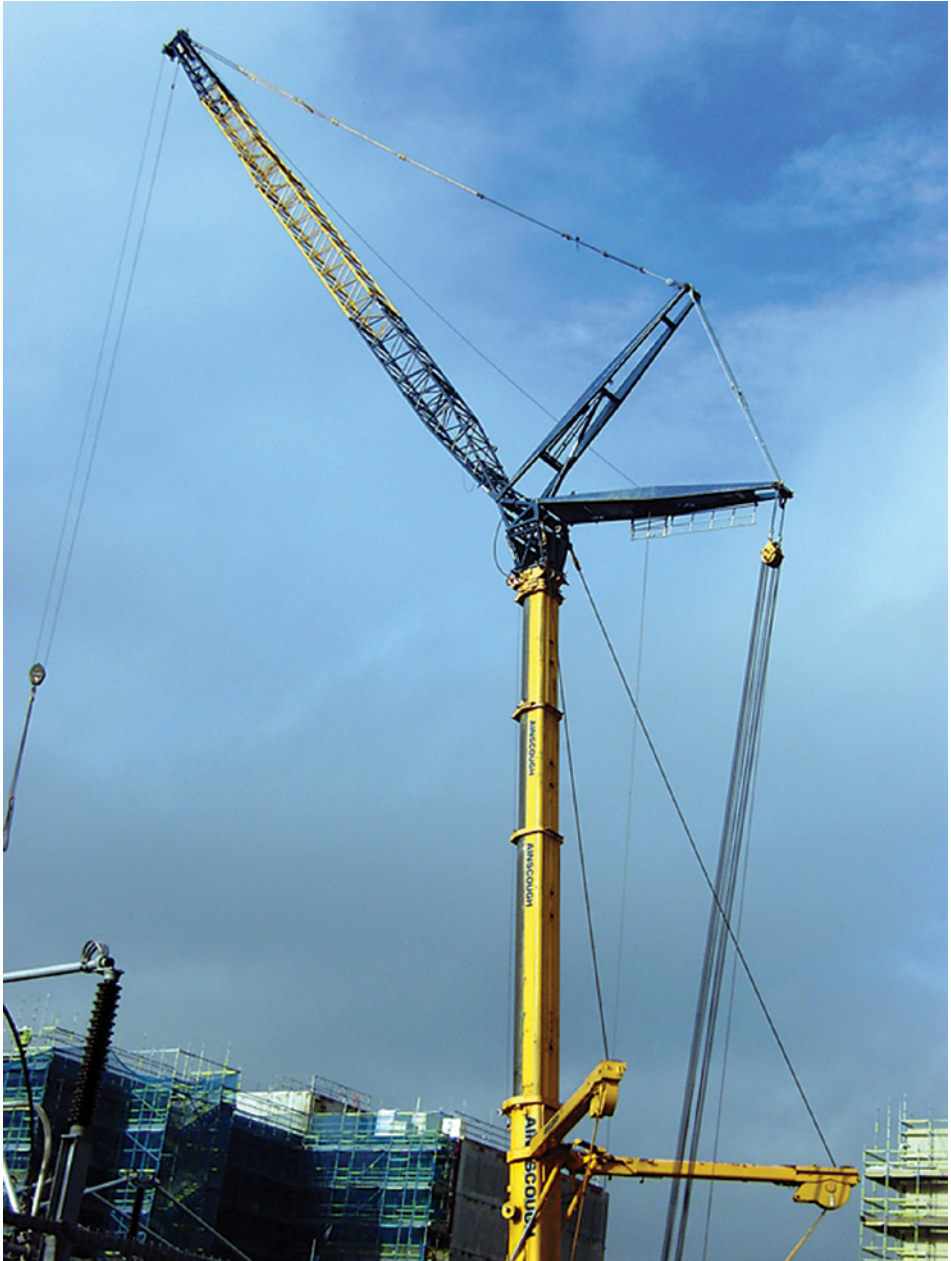
A self erecting tower crane with a telescopic tower (luffing jib tower crane for use on a restricted access site)
