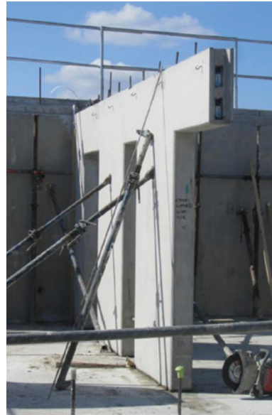
200 mm thick precast crosswall held in vertical position with extendable metal props
