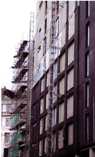
Example of an external skin of blue brick supported on metal angles fixed to the precast flank walls
