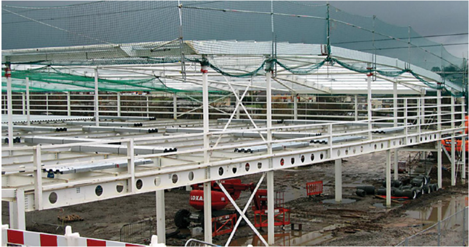
Image of two storey steel frame to the first floor car park. Metal Deck formed of heavy duty HOLORIB metal deck supporting a 150 mm insitu concrete slab
