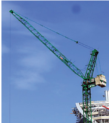
Luffing jib tower crane (to prevent crane moving over adjacent properties and roads etc.)
