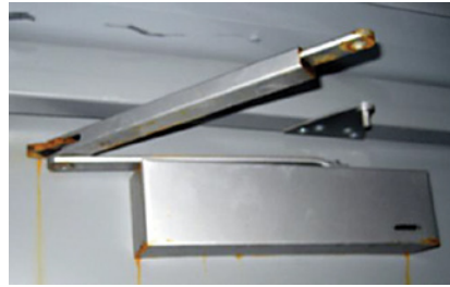
Defect item: broken door closure – replace complete fitting
