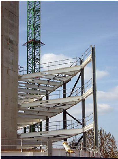
Main steelwork fixed to staircase and lift cores to provide rigidity to building frame
