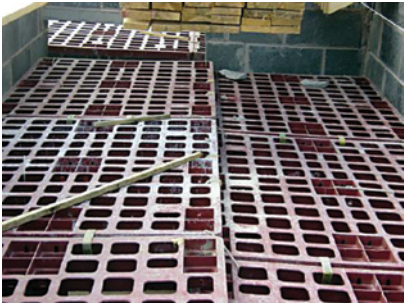
Safety Deck system in position 900 mm below the underside of the trusses
