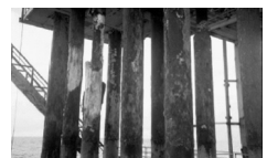
d) Corrosion damage
