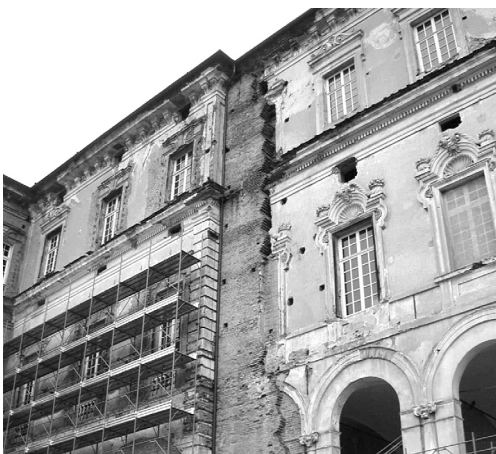
Figure 1. Facade of the Royal Residence of Venaria Reale (Turin, Italy) during its restoration works.
