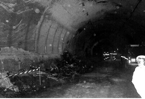
Figure 4. Vault and top slab damages.
