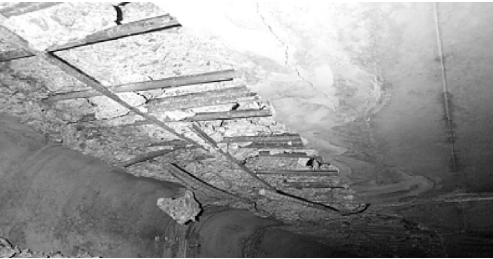
Figure 5. Concrete spalling of the carriageway slab intrados.
