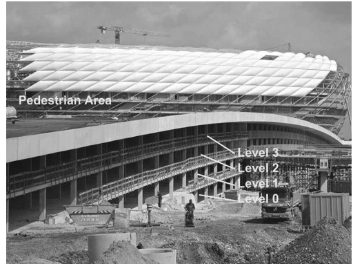
Figure 3. View of the Allianz Arena and the adjacent parking garage during construction.
