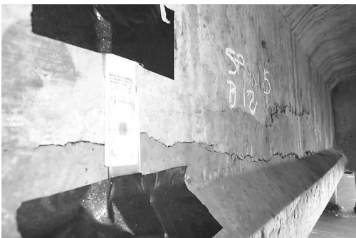
Figure 3. Typical longitudinal web crack along a beam.
