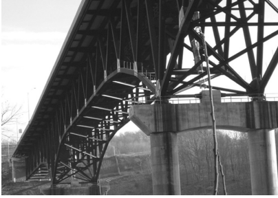
Figure 1. Photograph of the main span of the SR33 Lehigh River Bridge (photo taken by Sunyong Kim on 8 January 2008).
