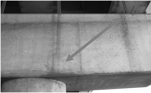
Figure 8. Diagonal cracks announcing a compressed strut.
