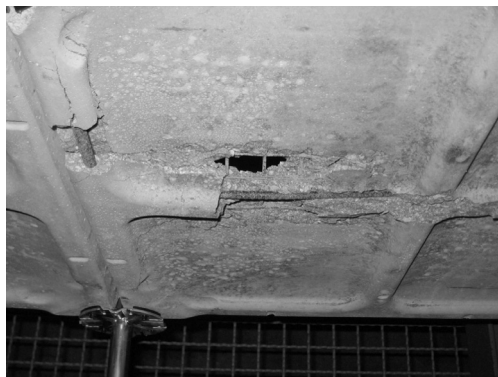
Figure 9. Example of panel collapse.
