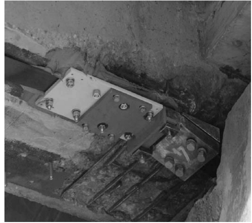
Figure 8. Fixed end anchorage plate of the CFRP strip with lock wedge.
