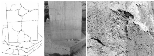
Figure 13. The coincidence of symptoms with different origins calls the attention specifically of well trained inspectors.
