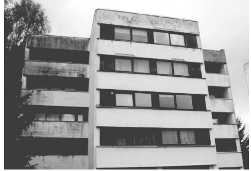
Figure 3. Degradation of concrete facade may cause aesthetic problems before the technical service life of the facade comes to end.
