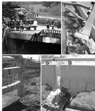
Figure 18. Railings: a topic that relates user's safety and structural aspects.
