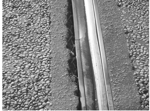
Figure 3. Failure of metal runner fixing in nosing.
