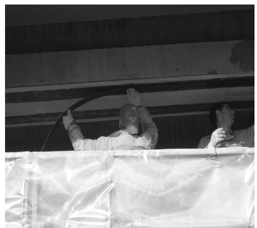
Figure 6. Application of the CFRP strip to be pre-stressed at the beam intrados.
