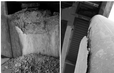
Figure 1. Left: concrete scaling, threatening the stability of a bearing device. Right: chloride induced corrosion attack.
