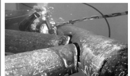
b) Fracture of a tubular joint
