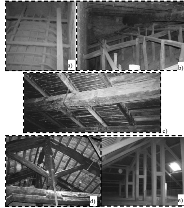
Figure 4. Horizontal structures: a) Wooden self-bearing vaults; b) Complex wooden structure; c) Wooden beam floor. Roofing structures: d) Wooden truss; e) R. c. trusses.
