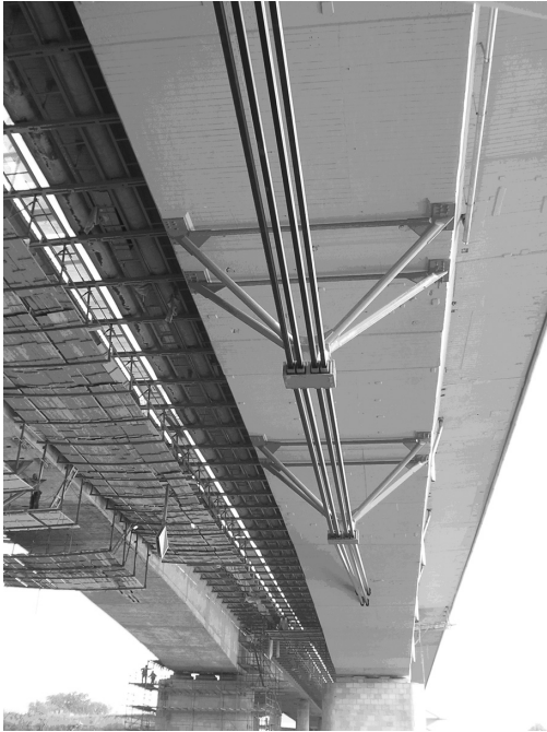
Figure 2. External tendons for structure relieving.
