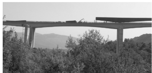
Figure 1. Longitudinal view of the central span of the viaduct (110 meter in length). At midspan the thickness of the box girder is 2200 mm while in correspondence of the piers is about 5500 mm. Overall this dimensions provide the bridge with a pleasant slenderness.
