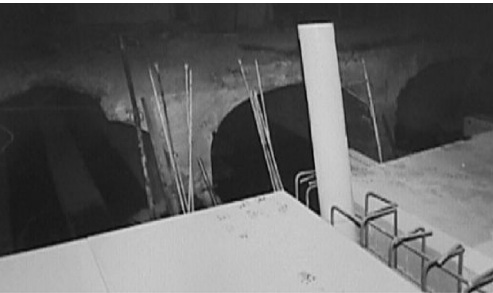
Figure 10. Replacement of abutment 3 – transition between box structure and arch structure at chainage 5.800.00.
