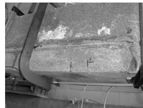
Figure 3. Detail of a fibre optic extensometer mounted to include the crack.
