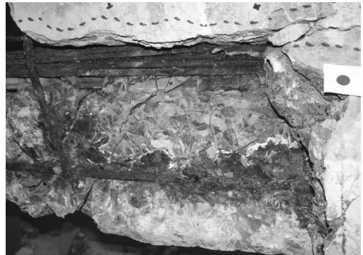
Figure 9. Extent of rust staining.
