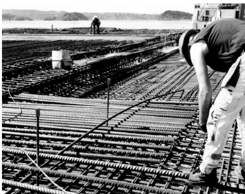
Figure 3. The concrete deck had very congested reinforcement.
