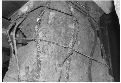
Figure 11. Collapsed column of a building with durability problems as well as poor design of details and construction.
