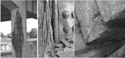
Figure 3. Degradation processes affect a great variety of structures and condition, always increasing with age.
