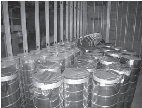
Ssealed Ducts – before installation
