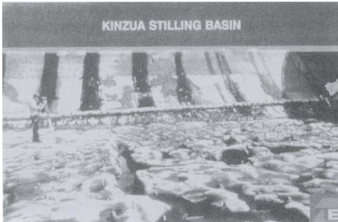
Fig. 12.10 Kinzu Dam, showing damage to high-strength fibre-reinforced concrete.
