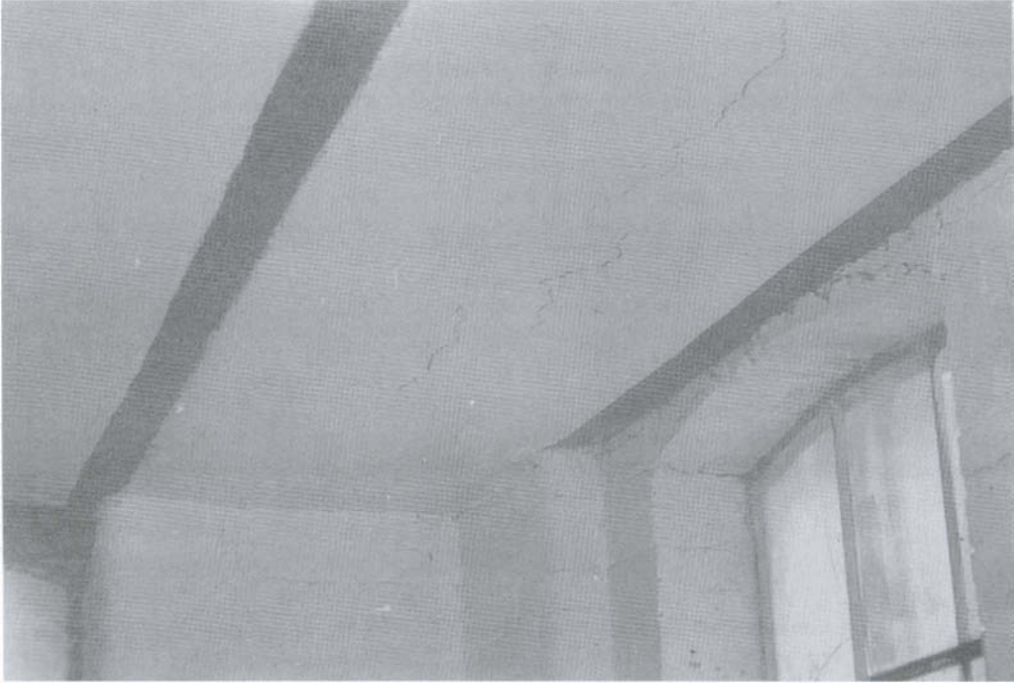
Fig. 16.33 Expansion and cracking of a flat concrete roof slab caused by unsound clinker aggregate. The view shows the ceiling on the underside of the recently water-penetrated roof slab in an early 20th century warehouse building in London, UK.
