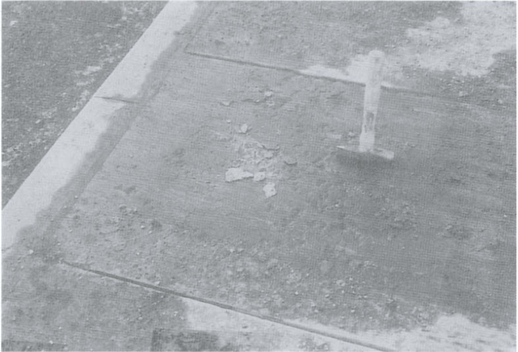
Fig. 16.29 Scaling of a concrete surface in the central reservation between two road carriageways in the English West Midlands caused by freeze-thaw damage involving a weak and porous oolitic limestone aggregate. The freeze-thaw damage had been greatly worsened in those areas most subjected to the wheel-splashed accumulation of water and de-icing salt.
