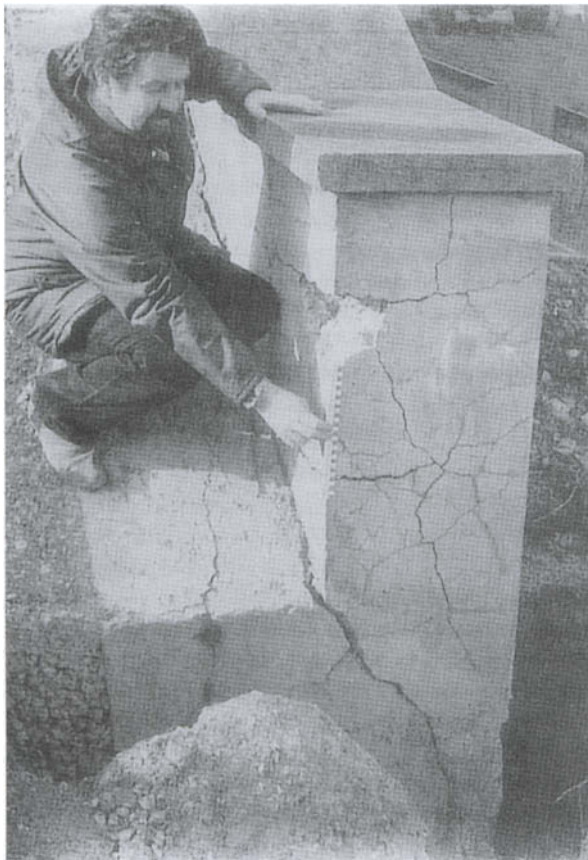
Fig. 16.22 Expansion, cracking and displacement of concrete caused by alkali-silica reactivity (ASR), affecting part of a bridge abutment in south-west England, UK. The reactive constituent was chert in the coarser fractions of the sand.
