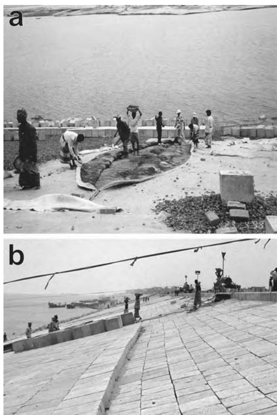
Figure 19.27 Construction of the B2 hardpoint at Sirajganj showing (a) dredged river silt covered with geotextile membrane filter, then covered by broken brick and concrete cubes (photograph courtesy of Mr Bob Courtier, W.S. Atkins Ltd) and (b) 0.45 \text{ m}^3 concrete blocks in place, view looking downstream from the hardpoint 'nose'
