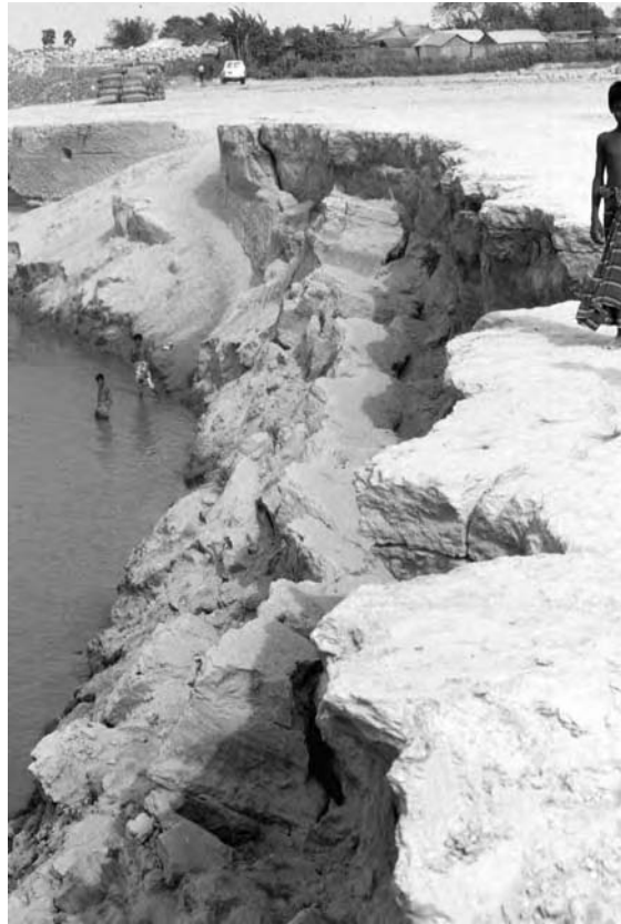
Figure 19.25 Large-scale slab failure by bank undercutting near Shailabari (~4 km upstream of Sirajganj). Photograph taken at low flow. During seasonal floods the water level would be up to bankfull
