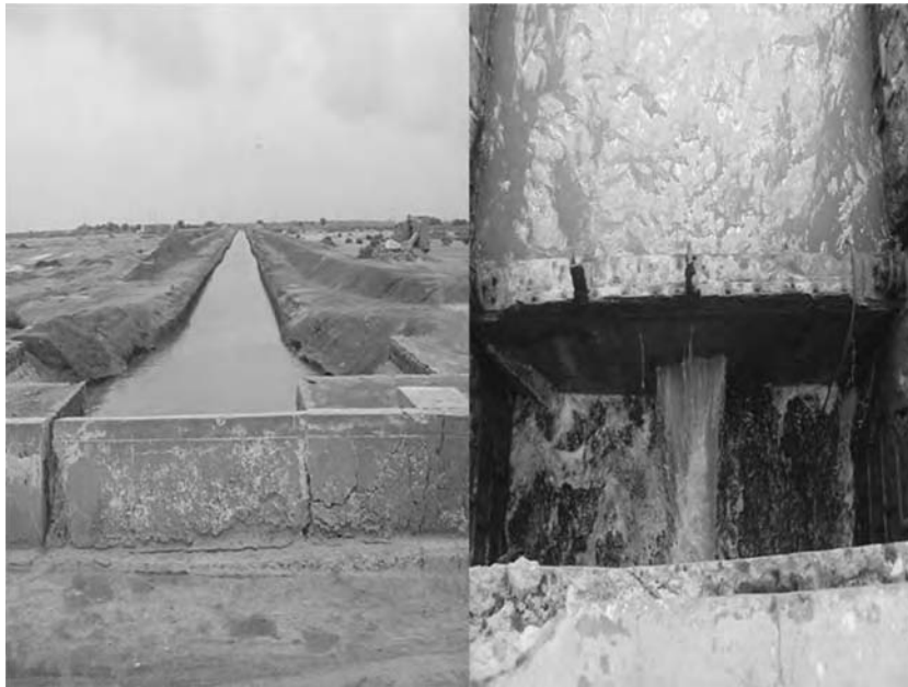
Figure 16.5 One of the drainage canals in the Indus deltaic area of Keti Bandar where the sea water is entering irrigated land through a defective gate
