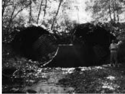
Figure 2 - Failing Culverts (NCD)
