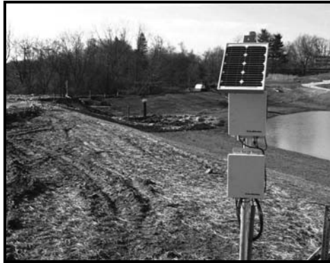
Figure 5. Remote automated electronic monitoring equipment setup
