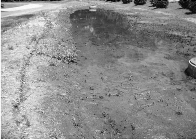
Figure 2. Ponded water on the biofilter surface observed after rainfall event (the vegetation cover is very poor indicating likely serious compaction).
