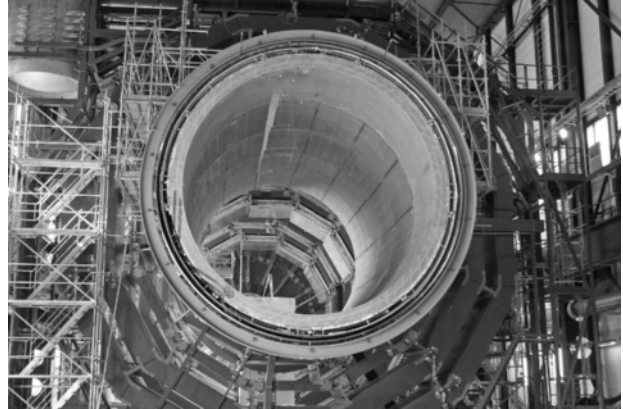
Fig. 2. Assembly of the yoke of the CMS magnet. The outer vacuum tank and the coil can be seen.
