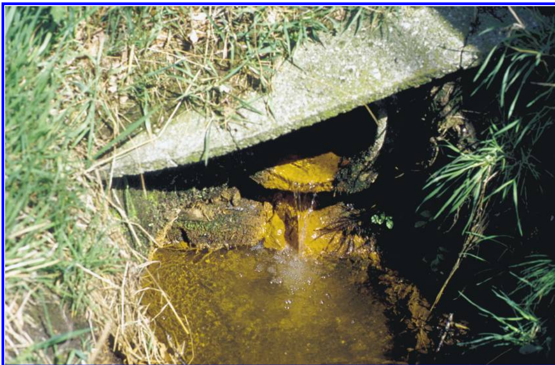
Figure 5.6. Top view of brownish iron hydroxide precipitate at a small stream emerging from a culvert, Uden, The Netherlands.
