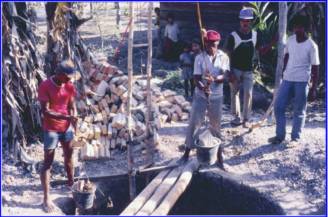
Figure 1.27. Constructing a large diameter well by hoisting loosened material from the excavated hole. Sulawesi, Indonesia.
