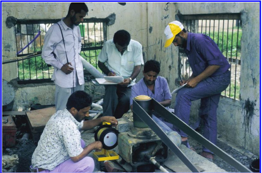
Figure 6.9. Pumping test carried out at an agricultural well in the Tihama Plain, Yemen.
