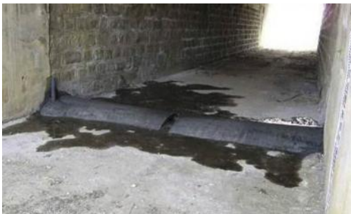
FIGURE 5.11 Culvert B (control subcatchment) weir designed for adequate gauging of flow with minimum impact on users.
