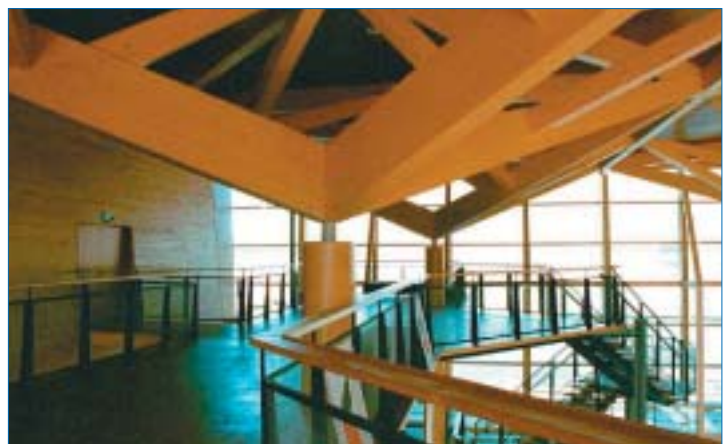
Fig 6.7 Sibelius Hall, Lahti Finland – junction detail of roof parasol beams to column tops in balcony area of atrium – connection steel work is entirely embedded within glulam to provide fire protection. © C.J.Mettem, TRADA Technology
