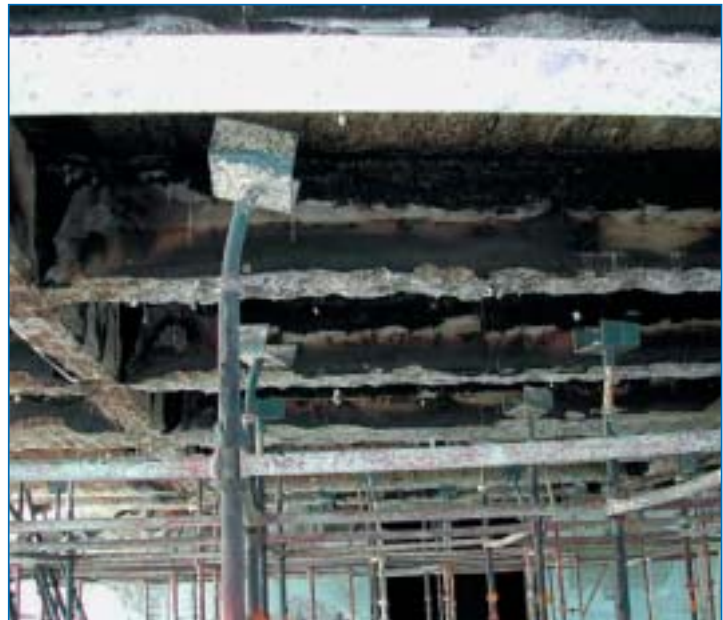
Fig 4.1 Fire in office building in Kuwait during construction. Post fire photograph showing damage to green concrete prior to carrying out repairs, and the distorted props that were used to support the timber formwork. © Buro Happold
