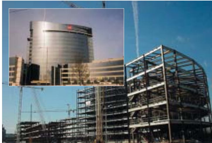
Fig 1.2 Glaxo Smith Kline building London – The GSK building involved repetitive large scale construction and fire safety engineering was used to design the edge beams to address constructability and improve safety. Offsite intumescent was more practical as a construction solution but the prescriptive fire resistance rating could not be economically achieved. An engineering approach looking at the natural fire effects on edge beams and considering the 3D behaviour of the structure enabled the use of offsite intumescent to achieve the required standard. © Hillier RHWL (view under construction), © Buro Happold (inset)
