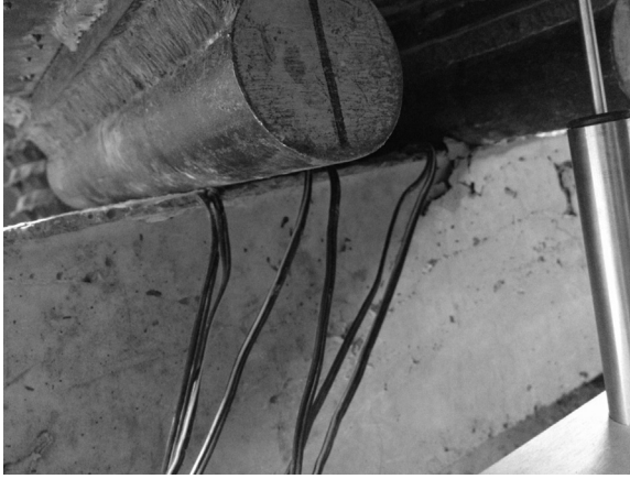
Figure 2.32 Crack at loading point with loading equipment in place.
