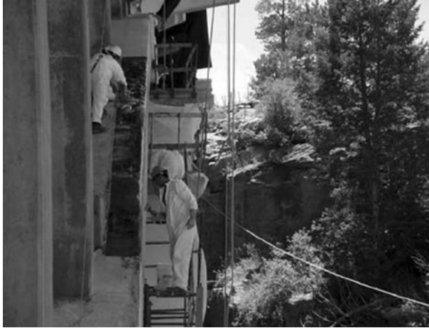
FIGURE 7.42 Applying FRP-wrapping laminates. (Courtesy of Colorado Department of Transportation: Fafach et al., 2005.)
