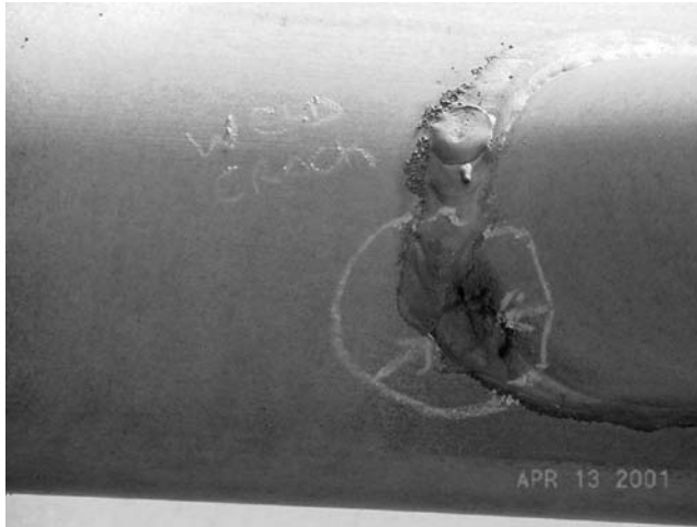
FIGURE 7.54 Details of a cracked welds in a road sign structure. (Courtesy of New York State Department of Transportation.)
