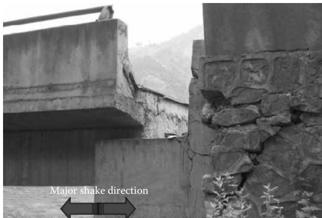
FIGURE 2.10 Excessive seismic abutment motion. (Courtesy of MCEER, University of Buffalo.)
