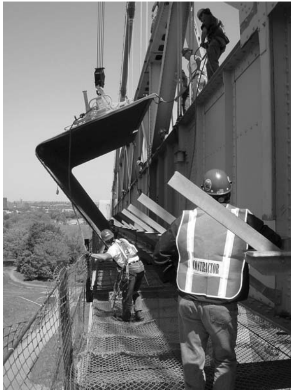
FIGURE 7.45 Installation of wind fairings at the side of the Bronx-Whitestone Bridge. (Courtesy Weidlinger Associates, New York City, NY.)
