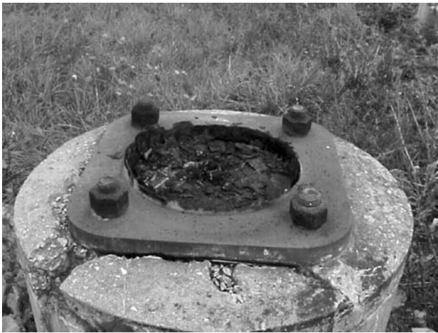
FIGURE 7.53 Deteriorated base of a road sign structure. (Courtesy of New York State Department of Transportation.)
