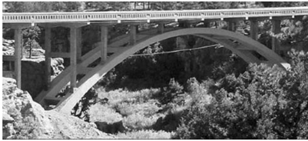
FIGURE 7.43 Bridge after rehabilitation. (Courtesy of Colorado Department of Transportation: Fafach et al., 2005.)
