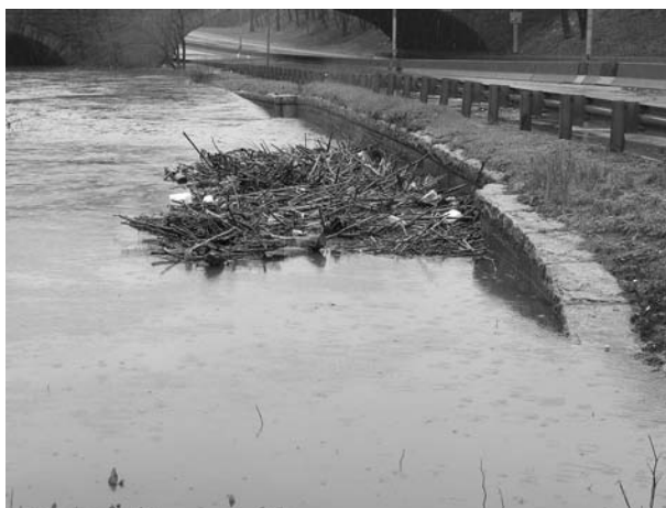
FIGURE 1.3 Debris damage during flooding. (Courtesy of New York State Department of Transportation.)
