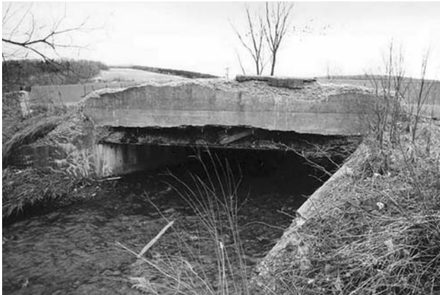
FIGURE 6.43 Old superstructure over Bennetts Creek. (Courtesy of New York State Department of Transportation.)
