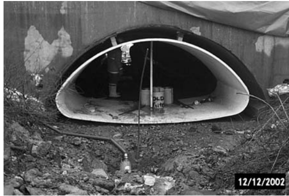
FIGURE 7.61 FRP culvert liners in place. (Courtesy of Erie County DPW of New York State.)
