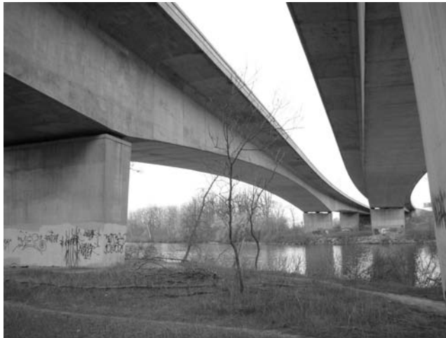
FIGURE 4.23 I-390 Bridge over the Genesee River, Rochester, NY. (Courtesy of Olson Engineering, Inc.)
