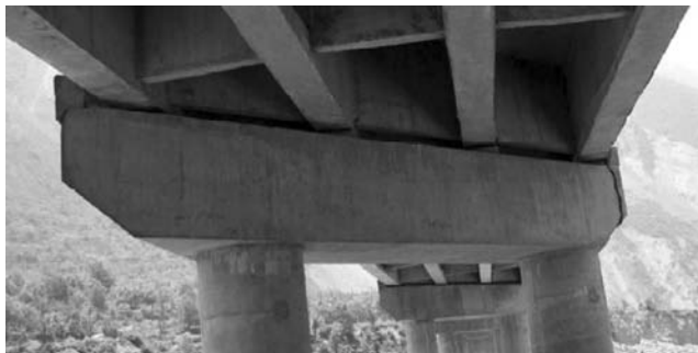
FIGURE 2.3 Seismic damage of skew bridge. (Courtesy of MCEER, University of Buffalo.)
