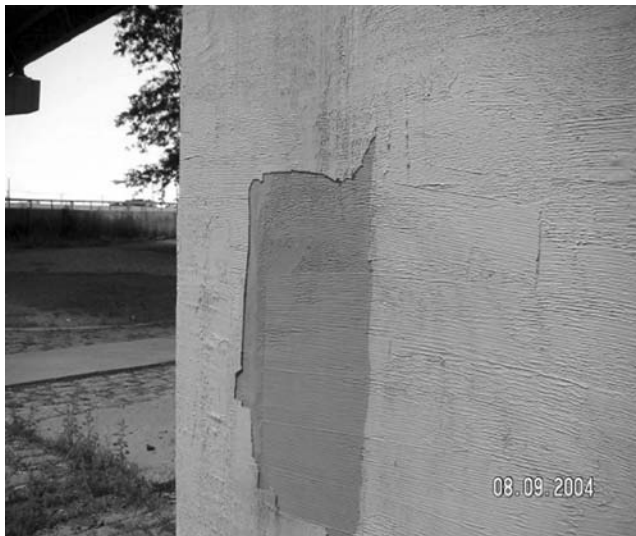
FIGURE 7.85 Surface peeling after 2 years. (Courtesy of New York State Department of Transportation.)
