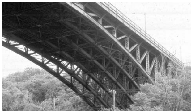
FIGURE 8.32 Potential ductile behavior during a load test of a steel bridge. With permission from National Highway Institute.
