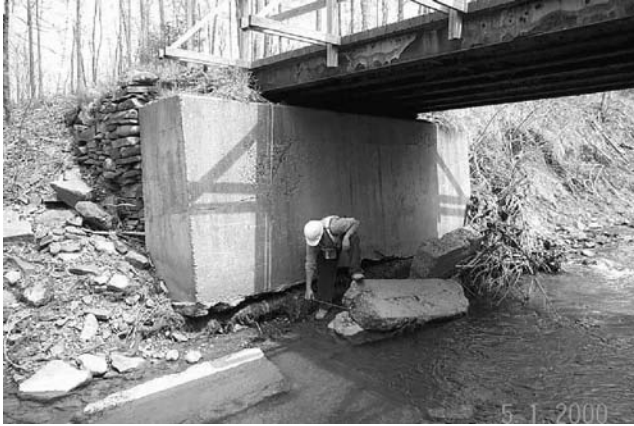
FIGURE 1.10 Local scour at abutment. (Courtesy of New York State Department of Transportation.)
