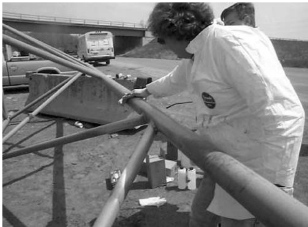
FIGURE 7.55 Preparations for FRP retrofits. (Courtesy of New York State Department of Transportation.)
