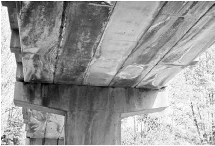
FIGURE 4.13 Leaking between adjacent box girders. (From Hartle, R. et al., Bridge inspector's reference manual, Federal Highway Administration, FHWA, Report No, FHWA NHI 03-001, McLean, VA, 2002, with permission from National Highway Institute.)
