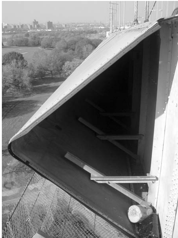
FIGURE 7.47 Longitudinal view of the installation of the wind fairings at the side of the Bronx-Whitestone Bridge. (Courtesy Weidlinger Associates, New York City, NY.)
