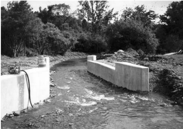
FIGURE 6.46 Abutments ready for new superstructure. (Courtesy of New York State Department of Transportation.)
