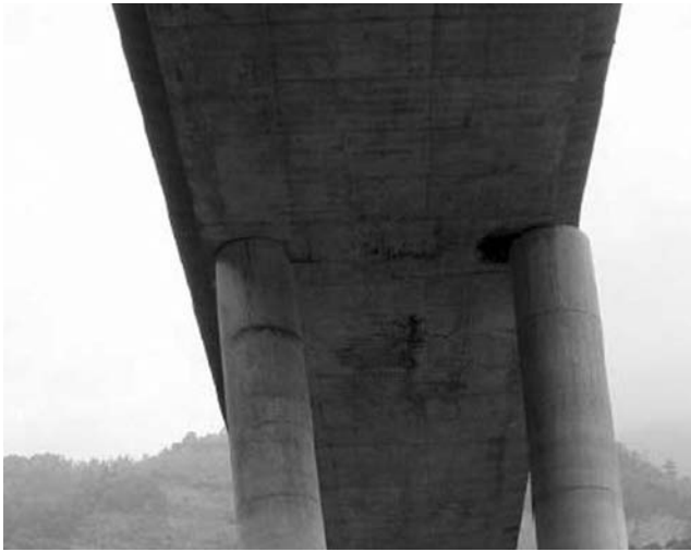
FIGURE 2.9 Failure of column-superstructure connection. (Courtesy of MCEER, University of Buffalo.)
