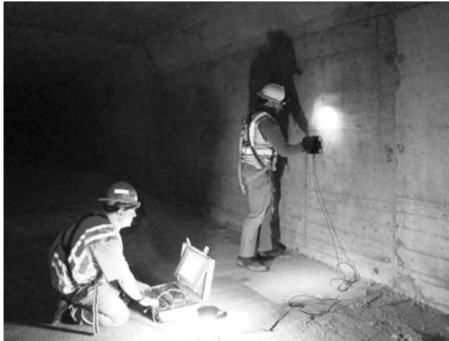
FIGURE 4.27 Typical impact-echo scan on box girder with duct voids. Courtesy of Olson Engineering, Inc.
