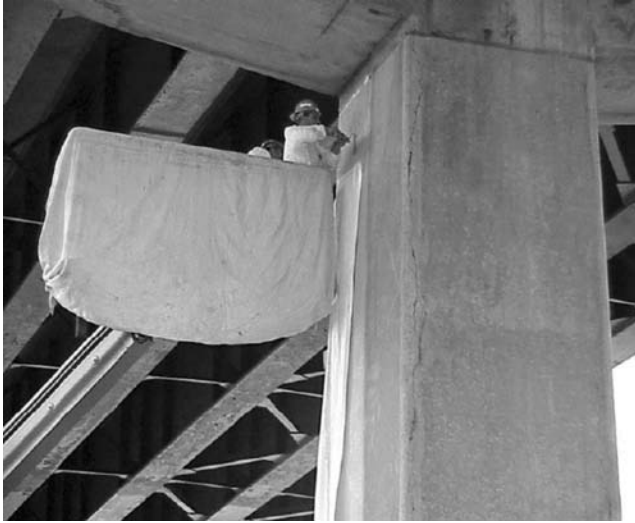
FIGURE 7.78 Application of retrofitting FRP laminates. (Courtesy of New York State Department of Transportation.)
