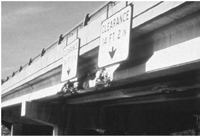
FIGURE 4.15 Traffic impact damage. (From Hartle, R. et al., Bridge inspector's reference manual, Federal Highway Administration, FHWA, Report No, FHWA NHI 03-001, McLean, VA, 2002, with permission from National Highway Institute.)
