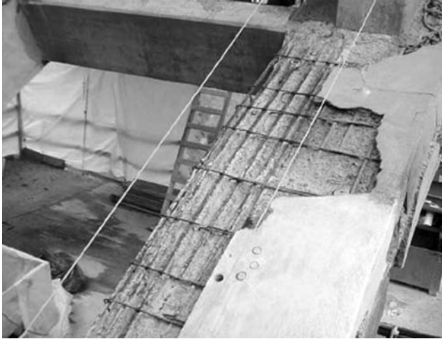
FIGURE 7.40 Exposed steel during construction. (Courtesy of Colorado Department of Transportation: Fafach et al., 2005.)
