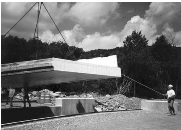
FIGURE 6.49 Moving new FRP superstructure into position. (Courtesy of New York State Department of Transportation.)
