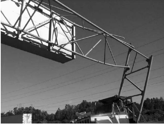
FIGURE 7.50 Damaged road sign structure. (Courtesy of New York State Department of Transportation.)
