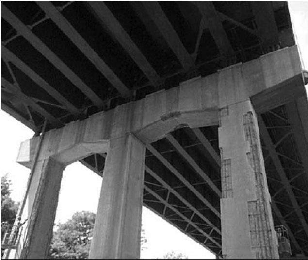
FIGURE 7.77 Removed delaminated and damaged concrete. (Courtesy of New York State Department of Transportation.)
