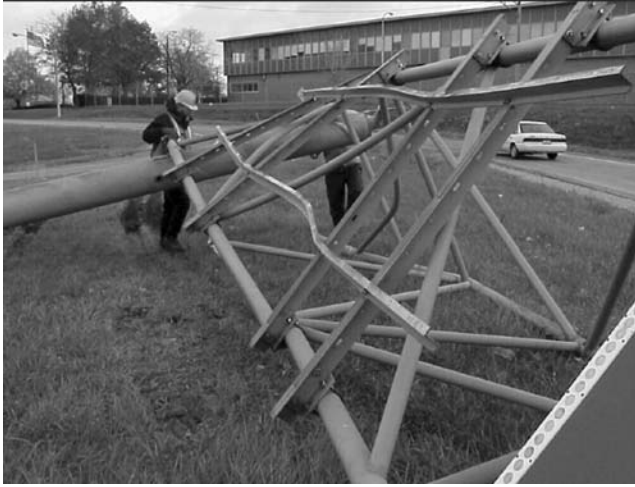
FIGURE 7.52 Inspection of a damaged road sign structure. (Courtesy of New York State Department of Transportation.)
