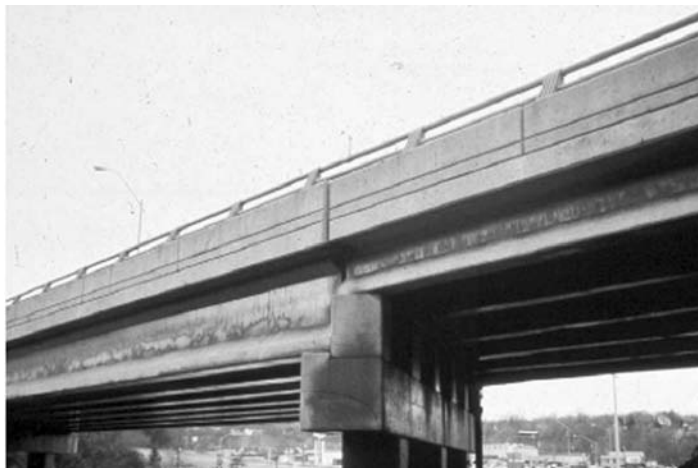
FIGURE 4.14 Leaking at end of beam. (From Hartle, R. et al., Bridge inspector's reference manual, Federal Highway Administration, FHWA, Report No, FHWA NHI 03-001, McLean, VA, 2002, with permission from National Highway Institute.)
