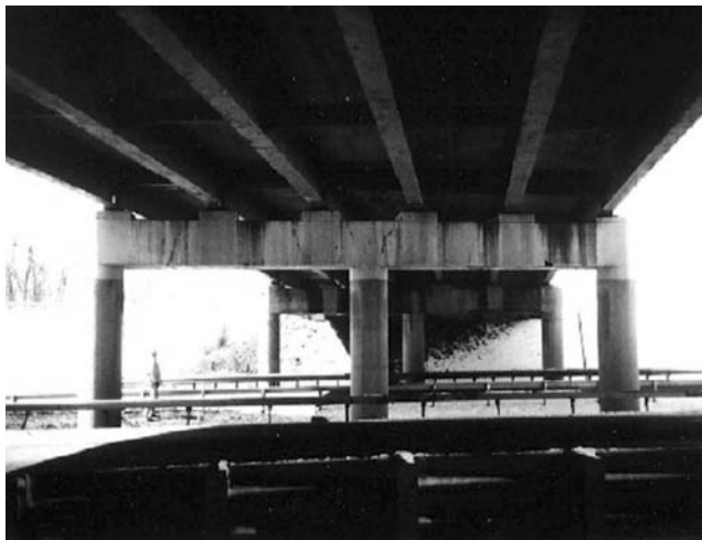
FIGURE 7.62 Deficient capbeams. (Courtesy of New York State Department of Transportation.)
