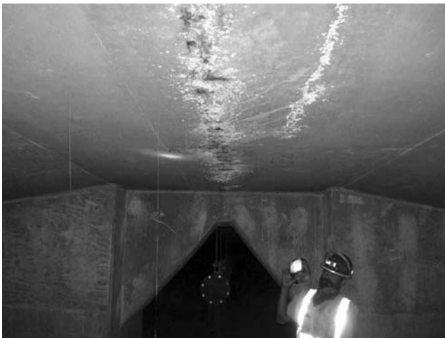
FIGURE 4.34 Signs of damage. (Courtesy of Siva Venugopalan.)
