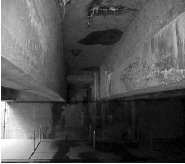
FIGURE 7.69 Deteriorated beams before retrofitting. (Courtesy of New York State Department of Transportation.)
