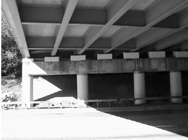
FIGURE 7.1 FRP wrapping to reduce exposure to road salt and inhibit corrosion. (Courtesy of New York State Department of Transportation.)
