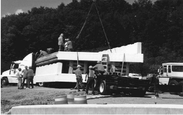
FIGURE 6.25 FRP superstructure delivered to site before installation. (Courtesy of New York State Department of Transportation.)
