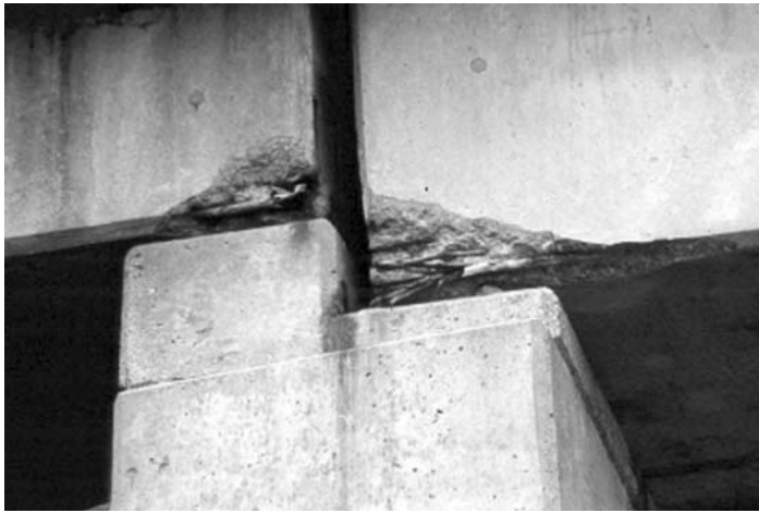
FIGURE 4.11 Damage near supports. (From Hartle, R. et al., Bridge inspector's reference manual, Federal Highway Administration, FHWA, Report No, FHWA NHI 03-001, McLean, VA, 2002, with permission from National Highway Institute.)
