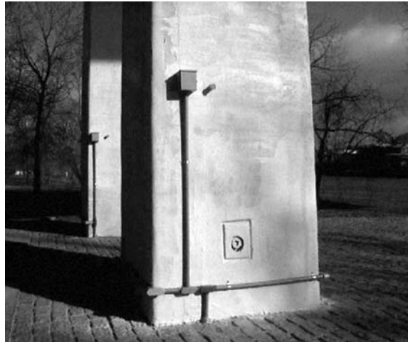
FIGURE 7.80 Placements of corrosion probe. (Courtesy of New York State Department of Transportation.)
