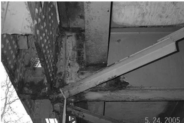
FIGURE 8.35 Potential brittle behavior during a load test steel beam problem. (Courtesy of New York State Department of Transportation.)
