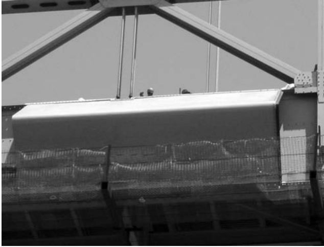
FIGURE 7.46 Lateral view of the installation of the wind fairings at the side of the Bronx-Whitestone Bridge. (Courtesy Weidlinger Associates, New York City, NY.)
