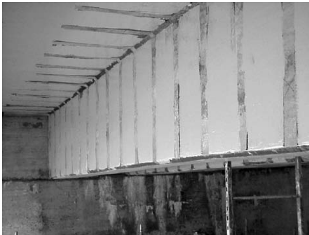
FIGURE 7.2 FRP wrapping of beams to increase flexural strength of bridge T-beams. (Courtesy of New York State Department of Transportation.)
