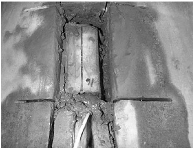
FIGURE 7.79 Installation of corrosion probe. (Courtesy of New York State Department of Transportation.)
