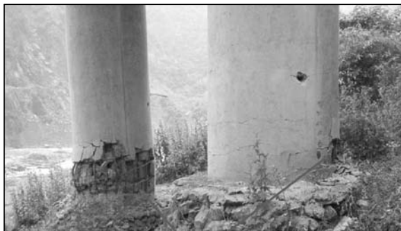
Damaged column of pier 1 perpendicular to the direction of fault
