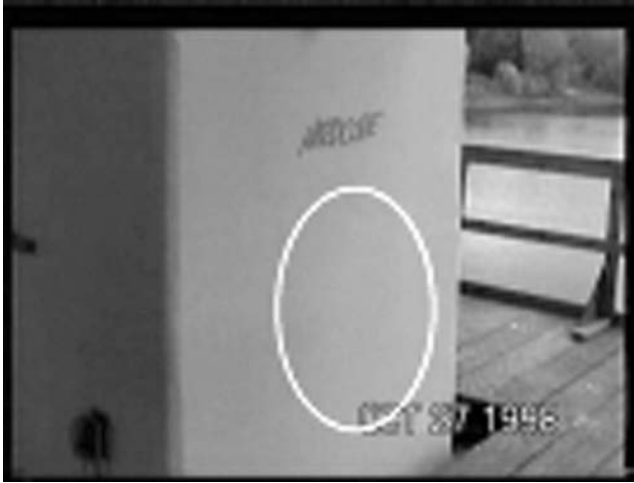
FIGURE 7.28 Photograph of an area—circled in white—on one of the FRP-wrapped columns that had disbondment and voids. (Courtesy of CRC Press.)
