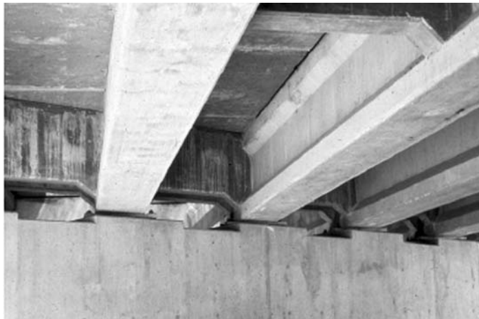
FIGURE 4.12 End diaphragm in an I-beam PSC system. (From Hartle, R. et al., Bridge inspector's reference manual, Federal Highway Administration, FHWA, Report No, FHWA NHI 03-001, McLean, VA, 2002, with permission from National Highway Institute.)
