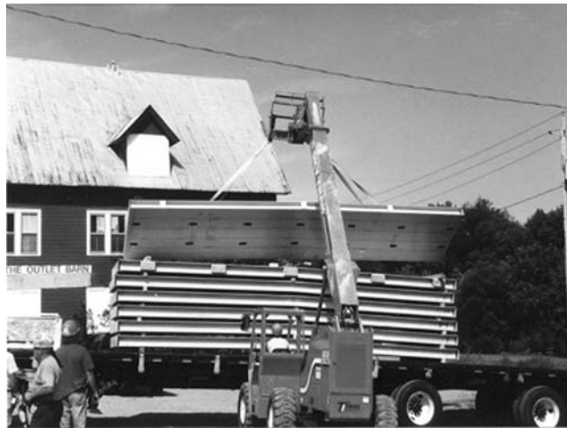
FIGURE 6.24 Sections of FRP deck delivered to construction site on a truck. (Courtesy of New York State Department of Transportation.)
