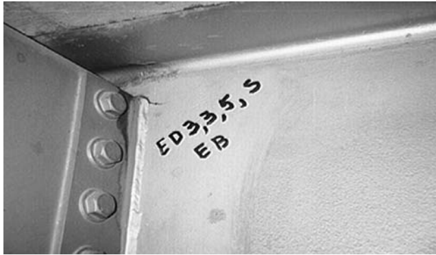
FIGURE 5.9 Fatigue crack—I-40, Edith Street Bridge. (Courtesy of CRC Press.)
