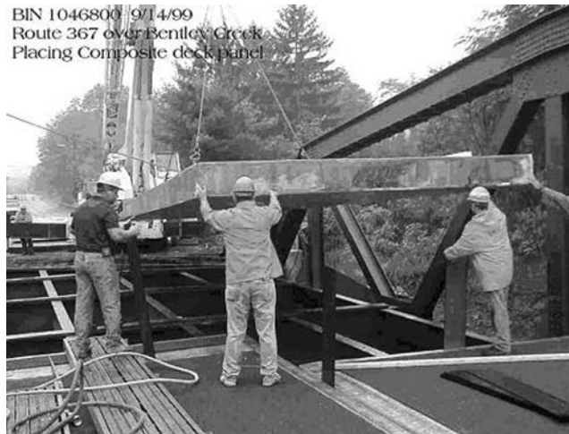
FIGURE 6.56 FRP bridge deck during erection. (Courtesy of New York State Department of Transportation.)
