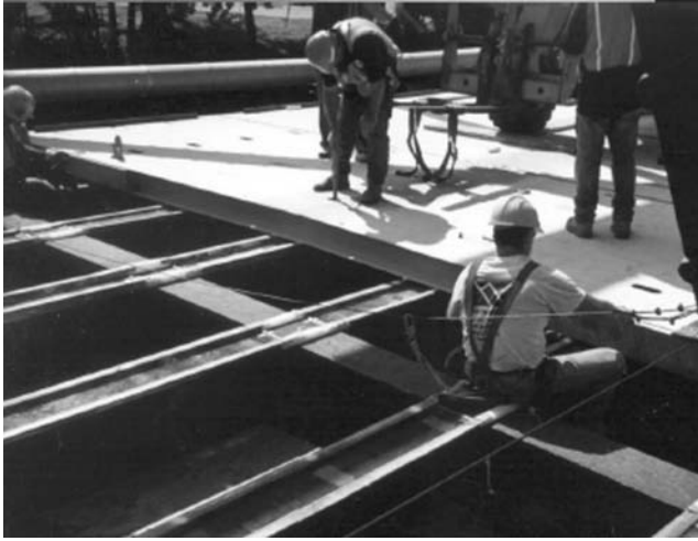
FIGURE 6.10 Connecting FRP bridge deck to steel supports. (Courtesy of New York State Department of Transportation.)
