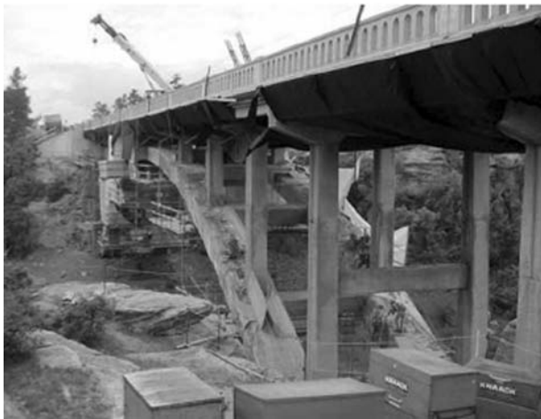
FIGURE 7.41 Arches during construction. (Courtesy of Colorado Department of Transportation: Fafach et al., 2005.)
