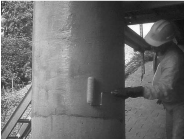
FIGURE 7.33 Finishing FRP wraps around bridge column. (Courtesy of New York State Department of Transportation.)
