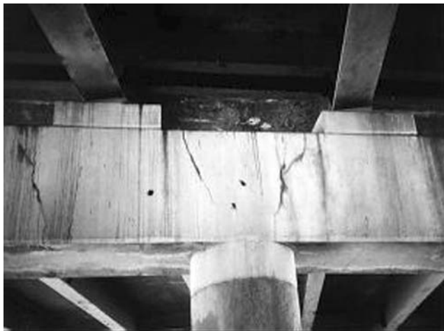
FIGURE 7.63 Detail of deficient capbeam. (Courtesy of New York State Department of Transportation.)
