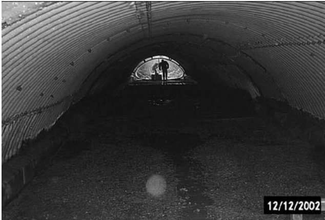
FIGURE 7.58 Longitudinal view of the culvert. (Courtesy of Erie County DPW of New York State.)
