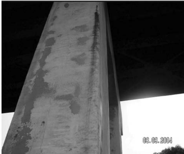
FIGURE 7.84 Rust spots after 2 years of retrofit. (Courtesy of New York State Department of Transportation.)
