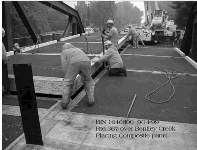
FIGURE 6.23 FRP bridge deck in New York during installation. (Courtesy of New York State Department of Transportation.)
