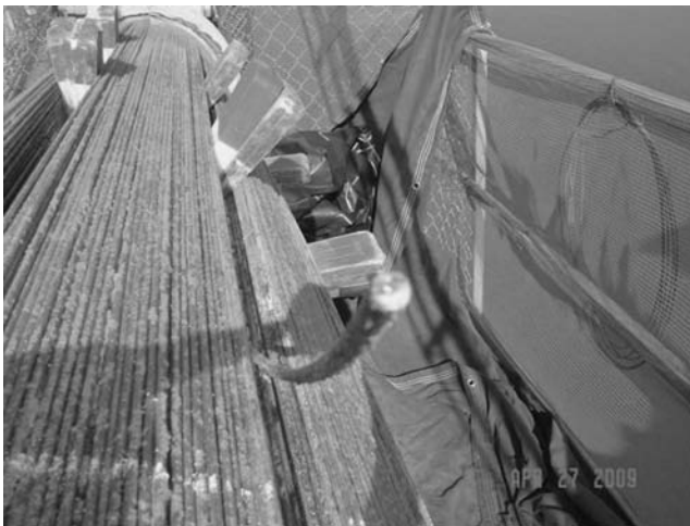
FIGURE 5.25 Damages in high-strength wires. (Courtesy of William Moreau.)
