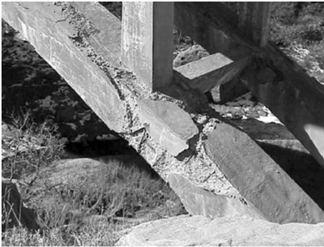
FIGURE 7.39 Damage in arch before rehabilitation. (Courtesy of Colorado Department of Transportation: Fafach et al., 2005.)
