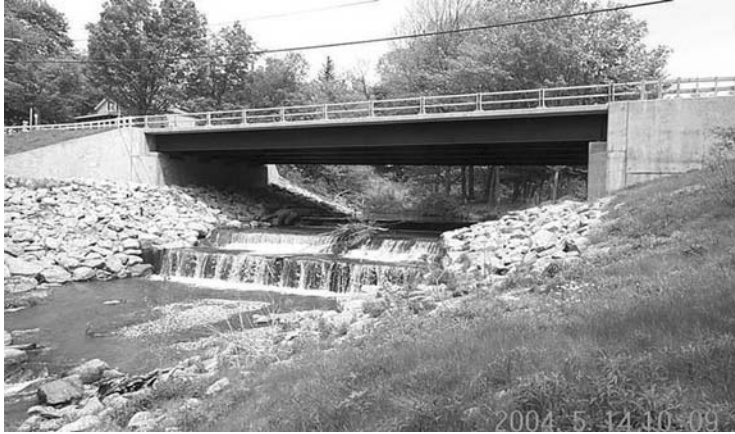
FIGURE 1.24 Check dam (under bridge). (Courtesy of New York State Department of Transportation.)
