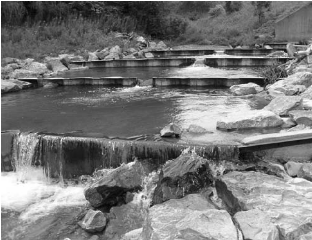
FIGURE 1.25 Check dam on the bridge approach. (Courtesy of New York State Department of Transportation.)
