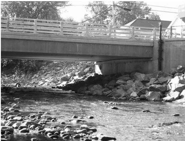
FIGURE 1.17 Riprap mitigation for scour. (Courtesy of New York State Department of Transportation.)
