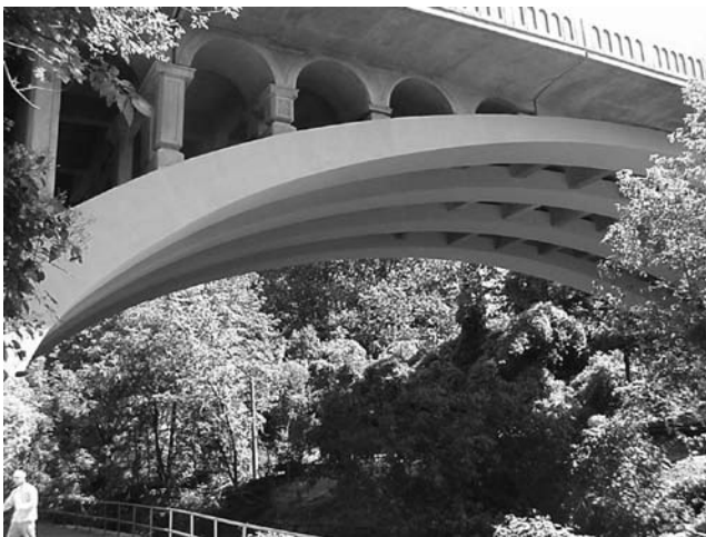
FIGURE 7.37 Woodlawn viaduct after strengthening with FRP wraps. (Courtesy of New York State Department of Transportation.)
