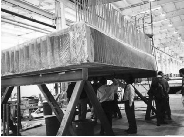
FIGURE 6.47 New FRP deck at manufacturing plant. (Courtesy of New York State Department of Transportation.)
