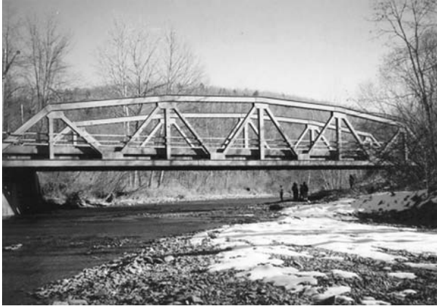
FIGURE 6.55 State Route 367, NY: Bentley Creek Bridge. (Courtesy of New York State Department of Transportation.)
