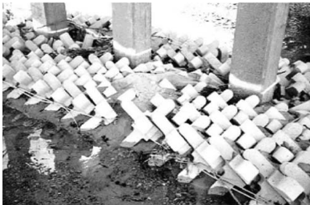
FIGURE 1.22 Concrete armor units over the I-33 bridge in Graves County, KY (HEC-23, with permission from National Highway Institute).
