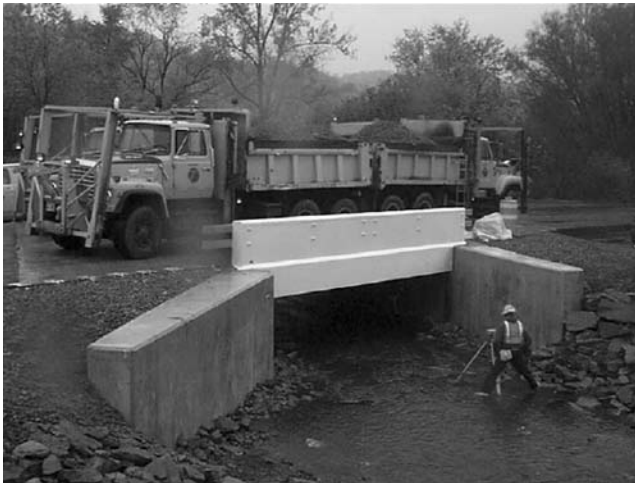
FIGURE 6.51 Load testing of new FRP superstructure/deck. (Courtesy of New York State Department of Transportation.)
