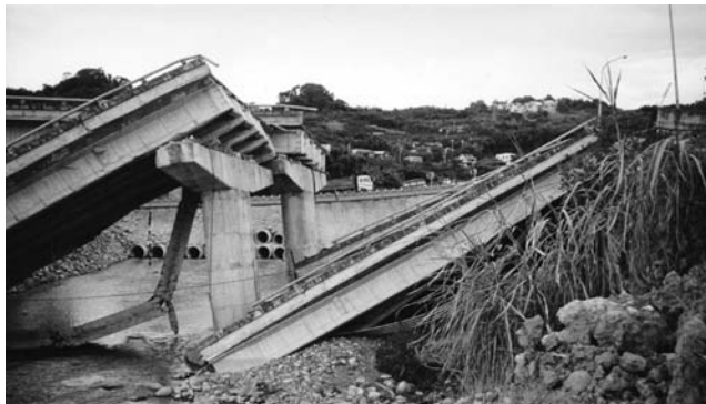
FIGURE 2.6 Unseating of joints during seismic events. (Courtesy of MCEER, University of Buffalo.)
