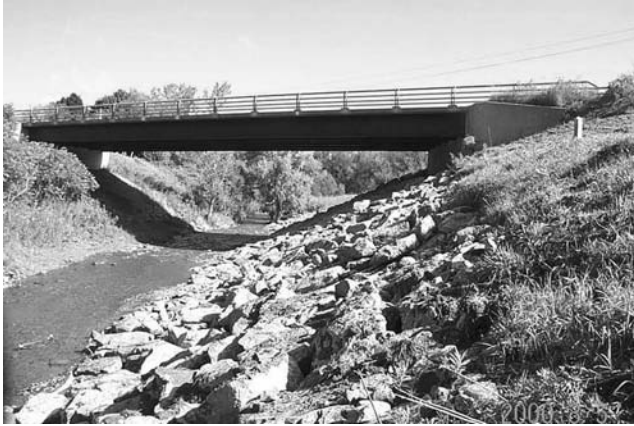
FIGURE 1.18 Riprap mitigation for scour. (Courtesy of New York State Department of Transportation.)
