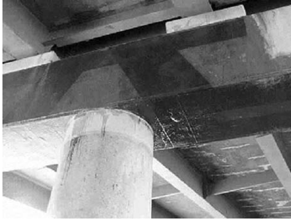
FIGURE 7.3 FRP Laminates to increase stiffness of capbeams. (Courtesy of New York State Department of Transportation.)
