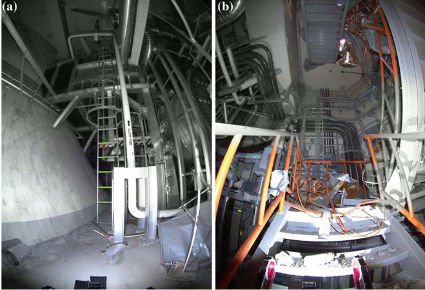
Fig. 1 High-resolution photos captured in the reactor building of unit 3. The left shows the piping of the core spray system and the right shows the rubble blocking the staircase to the third floor
