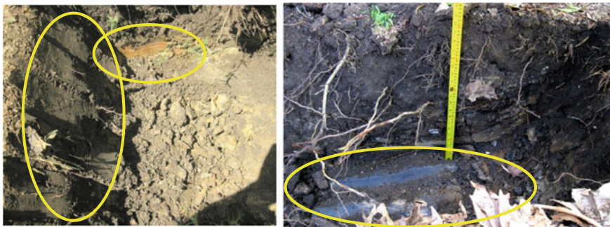
Fig. 9 Visual inspection of the opened trenches shows that except for the initial few centimetres of dry top soil the dominant material was clay. Shearing and dragging a full bucket of this material was enough to generate more than 1.5 tonne of reactions at the cylinders
