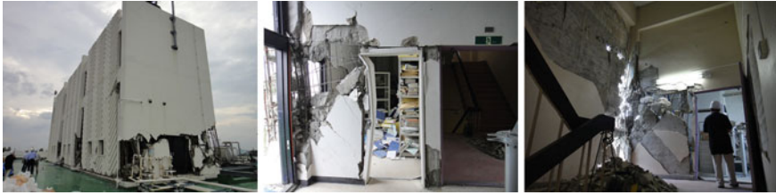
Fig. 2 The building suffered significant structural damage due to the earthquake
