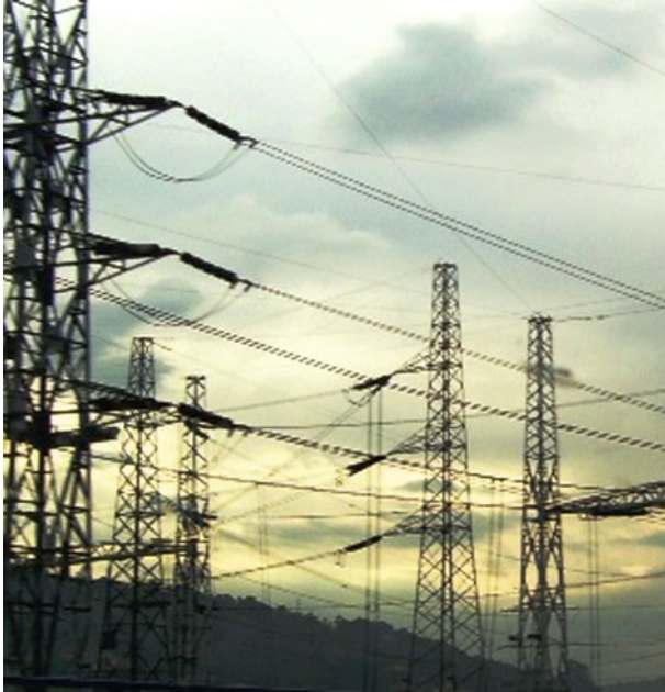
Fig. 16.3 Image of electricity transmission infrastructure
