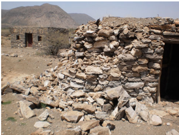
Fig. 9 Most houses in Sireru village were built on sedimentary infill on the caldera floor. Poorly built houses like the one shown collapsed. Behind, a better built one sustained only minor cracking
