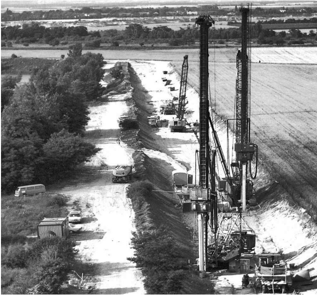
Fig. 11-11 Construction of the chambers of the Wiener Dichtwand Kammersystem (Vienna chamber system) using cut-off walls for the containment of the Rautenweg landfill, Vienna (Source: Archive of Bilfinger Berger Bauges. mbH (Building Company), Vienna)
