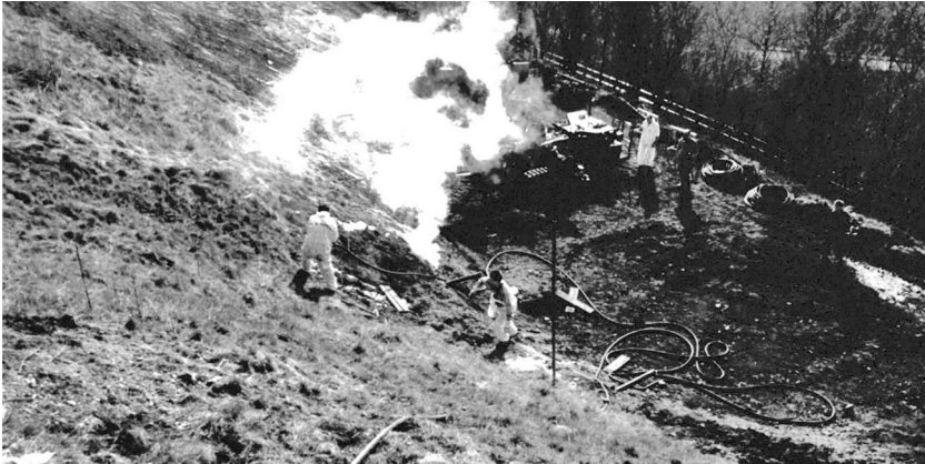
Fig. 11-25 Horizontal drillings injecting insulating material into the smouldering toe of the landfill embankment
