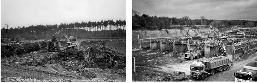
Fig. 11-28 Terraced excavation, sieving the plastics by a backhoe with a special fork-shovel (left). Computer and video controlled temporary storage of single batches in boxes until classification of the contamination by chemical analyses, followed by controlled transport to the specified facility (right) (Source: Archive of Bilfinger Berger Bauges. mbH (Building Company), Vienna)
