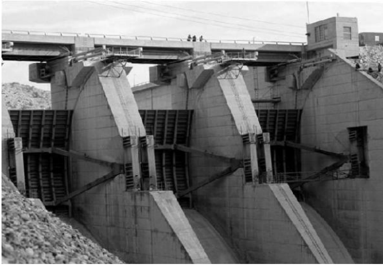
FIGURE 13.9 Top of a gravity spillway. The vertical piers divide the spillway into three bays and also incorporate the pivots for the radial gates and the machinery for raising/lowering the gates (cp Figure 13.11). (Courtesy of Black & Veatch, Overland Park, KS.)
