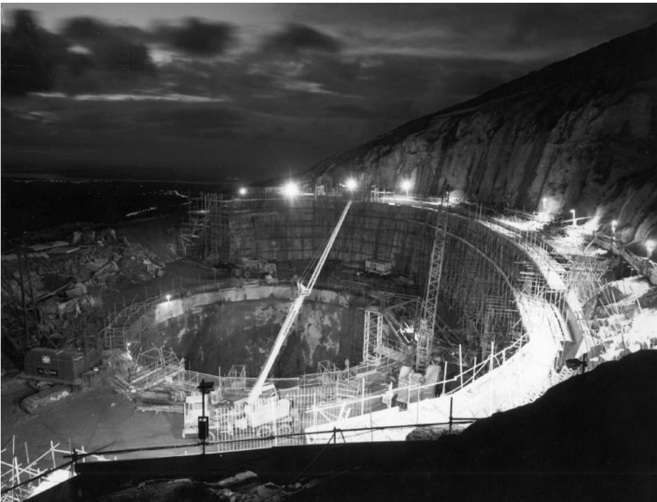
FIGURE 12.11 Construction of the surge tower for Dinorwig pumped storage scheme, Wales. (Photograph courtesy of CEGB/John Mills.)
