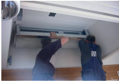
Fig. 9.30. Cooling and ventilation system integrated into the ventilation channel, developed by the company Climator (picture: Climator)
