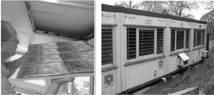
Fig. 9.18. Left: Installation of Dörkens DELTA ® -COOL 24 on top of a suspended ceiling. Right: Containers equipped with DELTA ® -COOL 24 for a field study performed in 2003 (pictures: Dörken)
