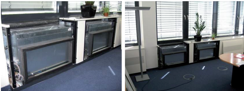
Fig. 9.28. Installed units with open and closed front plate (pictures: Imtech).
