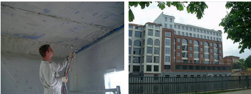
Fig. 9.32. Installation of 1100 m 2 plaster maxit clima ® on capillary sheets (picture: FhG-ISE) in a building in Berlin (picture: M. Schmidt).
