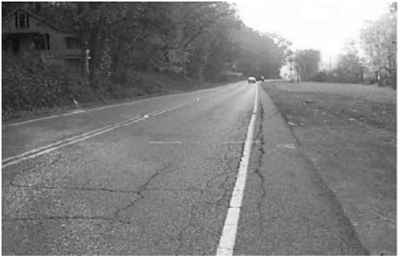
FIGURE 3.58 Localized edge cracking.
