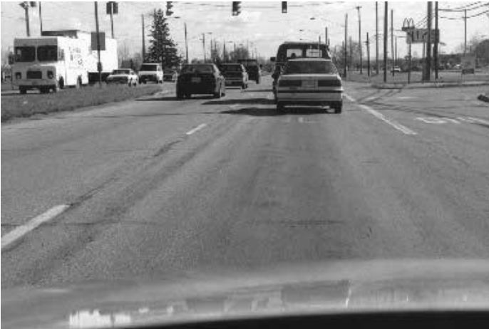
FIGURE 3.34 Example of rutting in flexible pavement.
