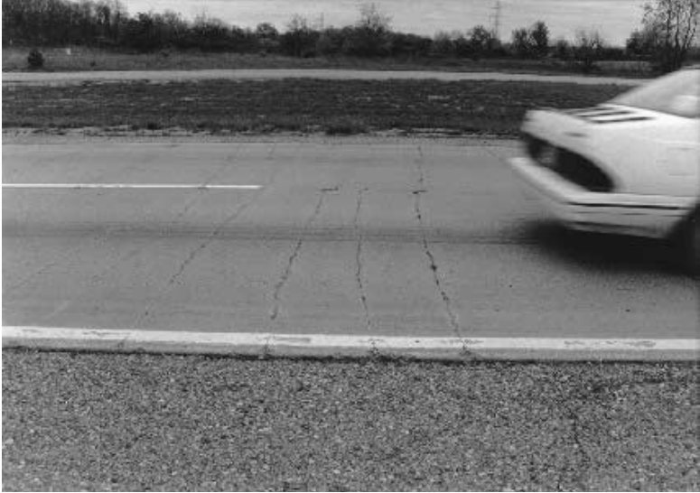
FIGURE 3.29 Example of transverse cracks spaced too closely in continuously reinforced rigid pavement.
