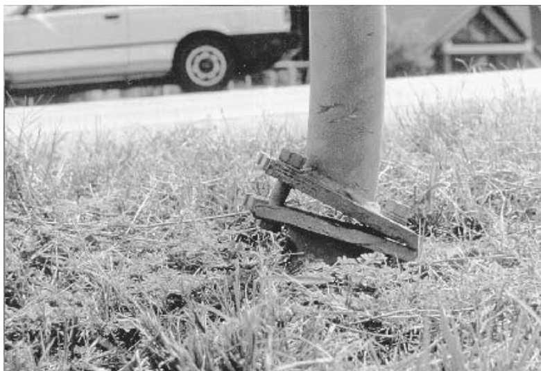
FIGURE 7.26 Loose slip base caused by vibration.
