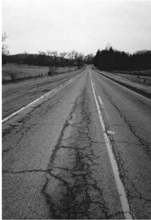
FIGURE 3.39 Example of wheel track cracking in flexible pavement.
