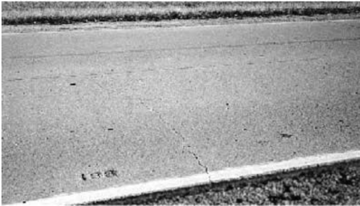
FIGURE 3.55 Hairline crack in rigid pavement.
