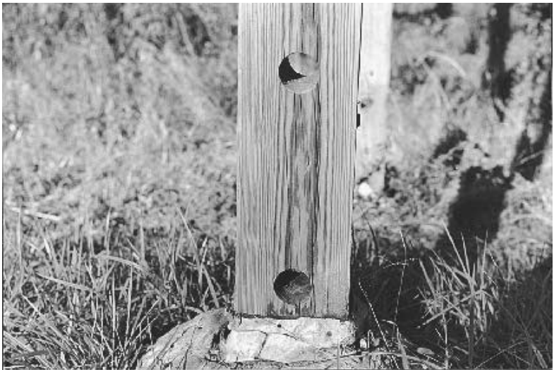
FIGURE 7.62 Weakened wooden post for multiple supports.
