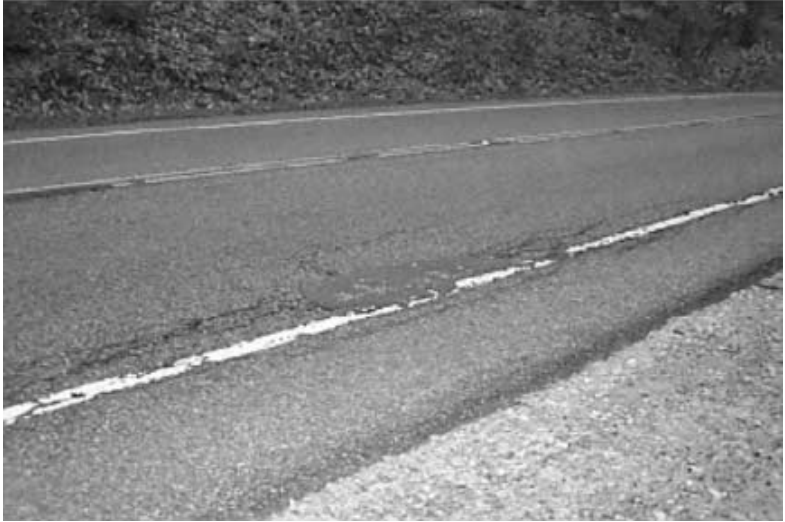
FIGURE 3.57 Localized wheel track and edge cracking.
