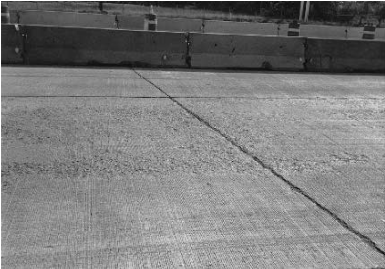
FIGURE 3.22 Example of surface deterioration in jointed rigid pavement.
