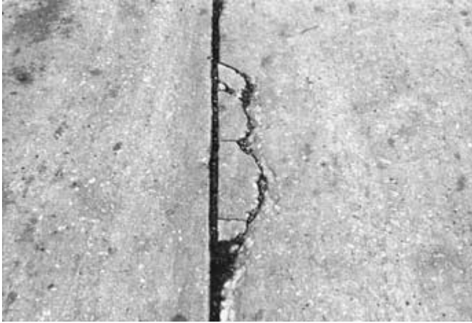
FIGURE 3.25 Example of joint spalling in rigid pavement.
