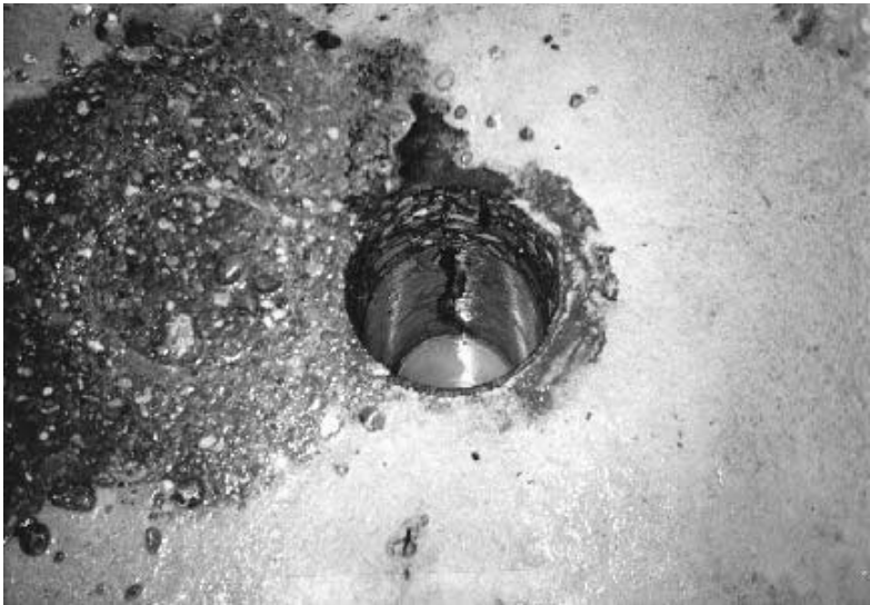
FIGURE 3.42 Hole in pavement after core was drilled at transverse crack in composite pavement.
