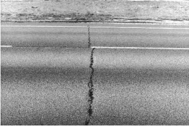
FIGURE 3.37 Example of transverse cracking in flexible pavement.
