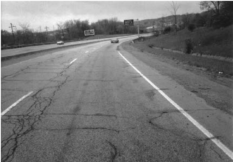
FIGURE 3.38 Example of block cracking in flexible pavement.
