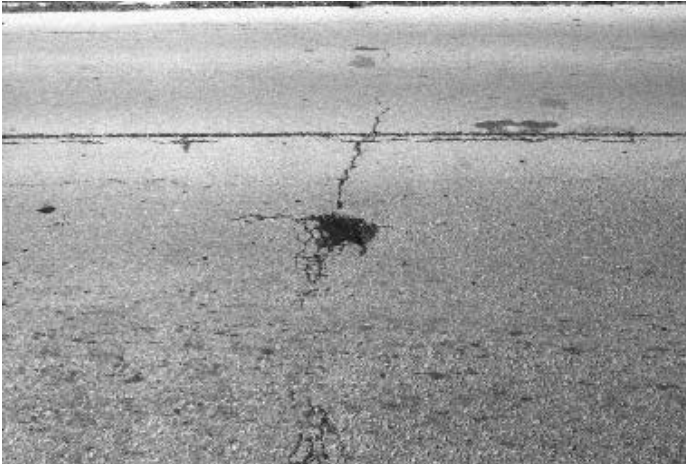
FIGURE 3.33 Example of small pothole in flexible pavement.
