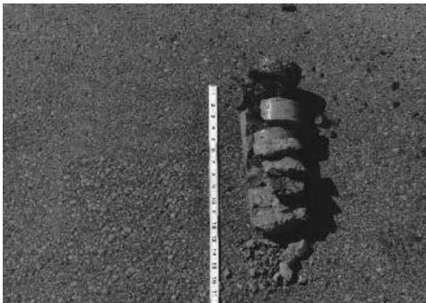
FIGURE 3.44 Crumbled core taken from transverse joint in composite pavement.
