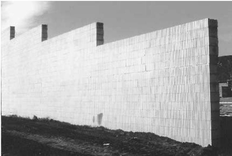
FIGURE 9.2 Concrete-block noise wall with vertical groove treatment, stepped in height.
