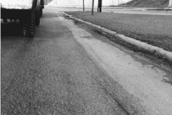
FIGURE 3.35 Example of corrugations in flexible pavement.
