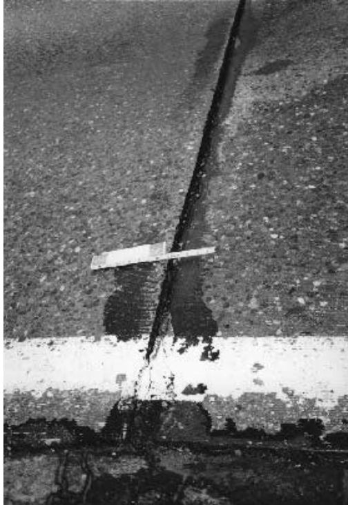
FIGURE 3.24 Example of faulting at joint in rigid pavement; pavement on right is about \frac{1}{2} in lower than that on left.
