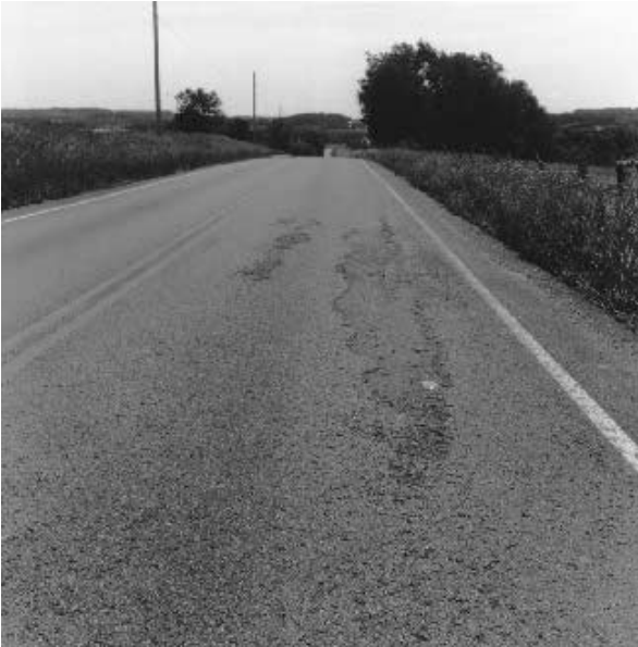
FIGURE 3.31 Example of raveling in flexible pavement.
