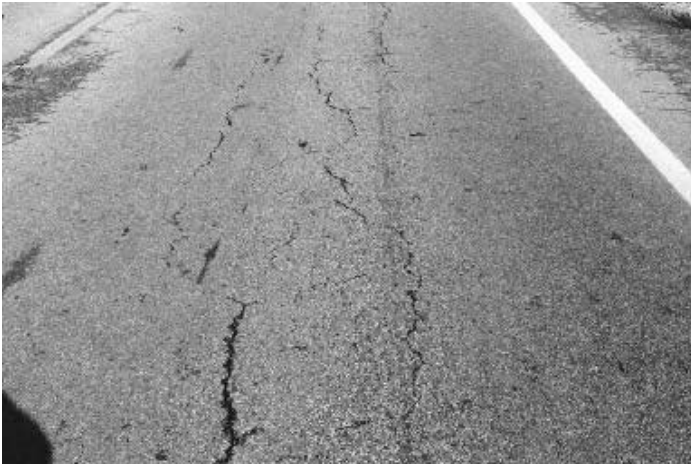
FIGURE 3.36 Example of longitudinal cracking in flexible pavement.
