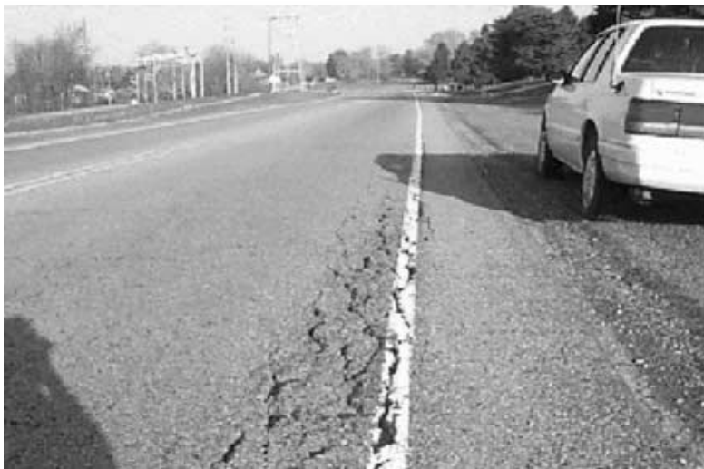
FIGURE 3.56 Localized edge cracking must be repaired full depth before chip sealing.
