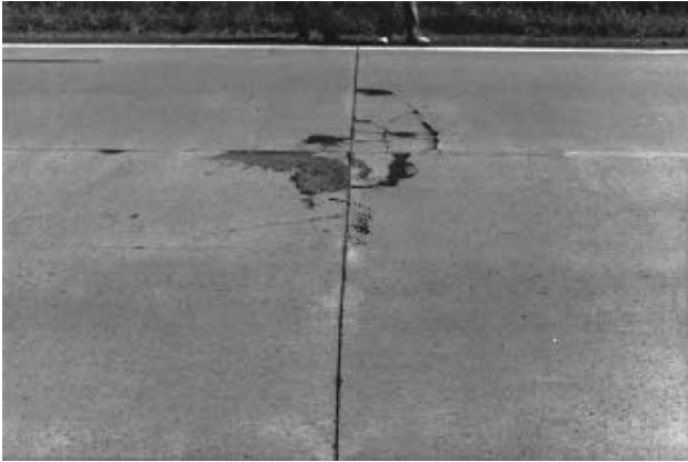
FIGURE 3.28 Example of corner break in jointed rigid pavement.
