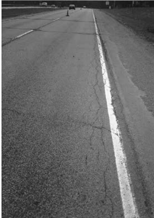
FIGURE 3.40 Example of edge cracking in flexible pavement.
