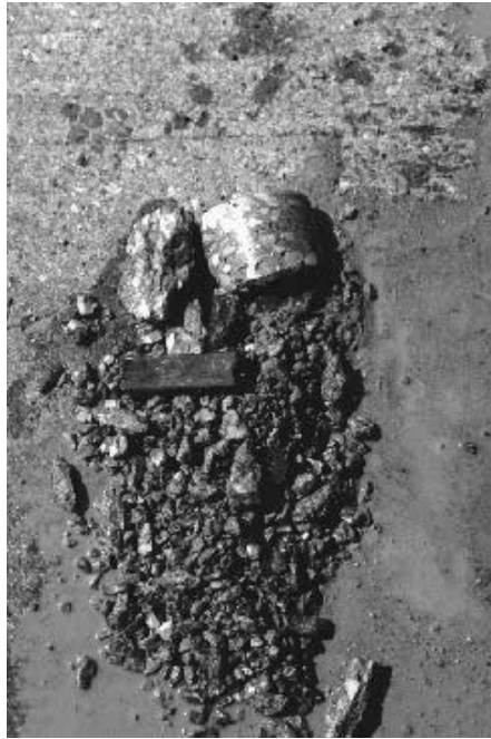
FIGURE 3.43 Crumbled core taken from transverse joint in rigid pavement.
