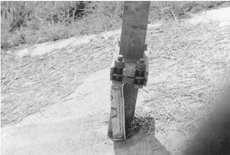
FIGURE 7.52 Improper installation of slip base anchor piece.
