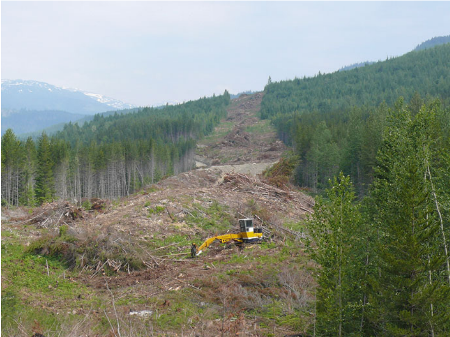
Fig. 2.2 The 287 kV Northwest Transmission Line, under construction in this image, will stretch 344 km across an undeveloped but mineral-rich region of northwestern BC (Photo by C. Johnson). The transmission line will provide electricity to planned and future mines as well as an interconnection point for run-of-river hydroelectric development. The right-of-way and associated infrastructure (effects) will have direct impacts on biodiversity and other values. More complex, however, are the indirect economic growth-inducing effects resulting from the provision of inexpensive electricity to large industrial projects. The positive and negative impacts of future resource development will greatly exceed the impacts of the transmission line; however, those impacts are difficult to predict and consider during project assessment and approval
