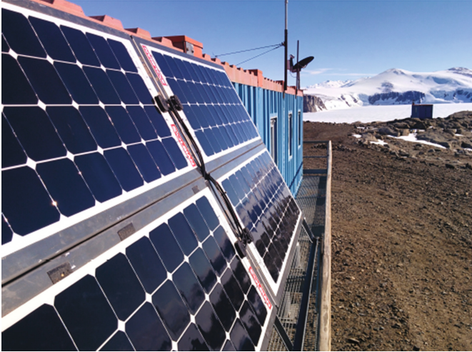
Fig. 4. Solar panels used by the system as primary source of energy.
