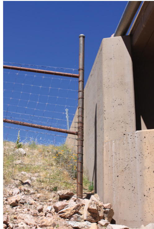
Figure 20.1 Depending on the species, the join between this bridge abutment and fauna fence may be too large, allowing animals to breach the fence and access the roadway. Source: Photograph by R. van der Ree.
