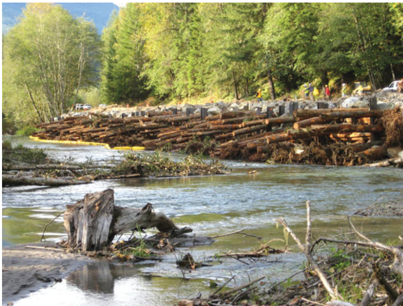
Figure 44.4 A change in approach is needed to address the habitat loss by continued use of rip-rap. The Sauk River wood cribwall is an example of a more natural approach, Washington, USA. Source: Photograph by Paul J. Wagner.
