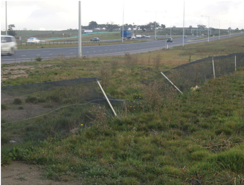
Figure 31.4 Amphibian fencing that has fallen over and is no longer functional. Frogs are able to cross onto the busy freeway, risking death or injury. The crossing structure accompanying the fence is shown in Figure 31.5. Source: Photograph by R. van der Ree.
