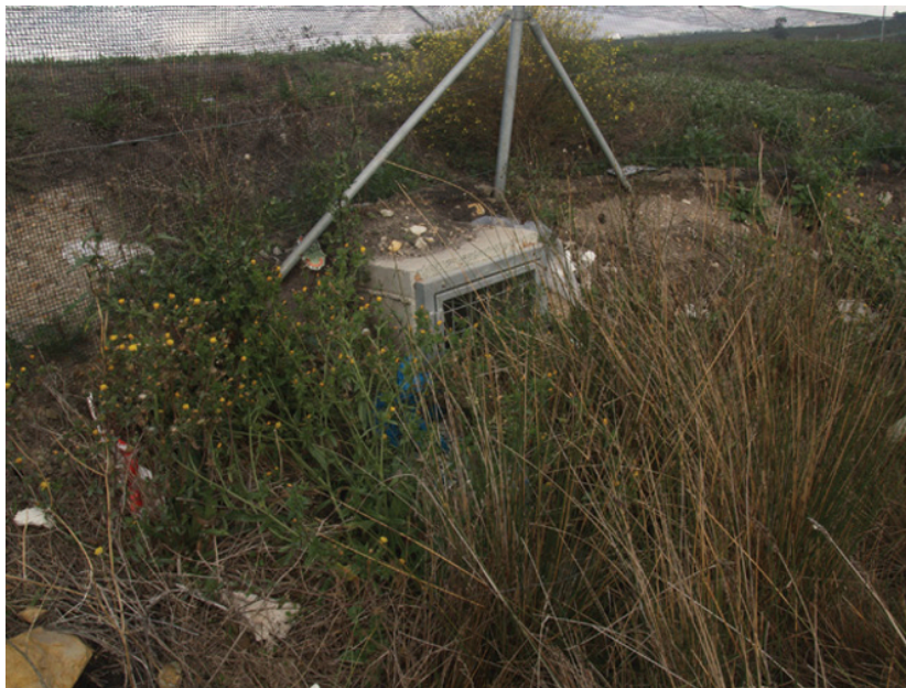
Figure 31.5 Poorly designed and maintained underpasses for the growling grass frog, an endangered species in south-east Australia. The fence is not flush with the tunnel entrance and does not direct frogs into the tunnel. The culvert also has no ventilation slits and is probably dry. The entrance is overgrown with vegetation. There is no evidence that frogs move through this structure. Photograph by R. van der Ree.
