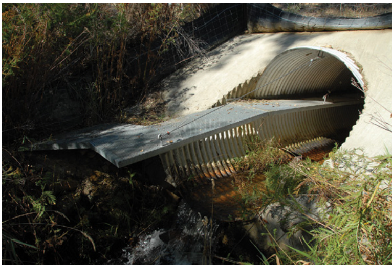
Figure 35.7 Bolt-on wildlife shelf retrofitted to an existing drainage culvert for use by weasels. Source: Photograph by and reproduced with permission of Kerry Foresman, Critter-Crossing Technology L.L.C.
