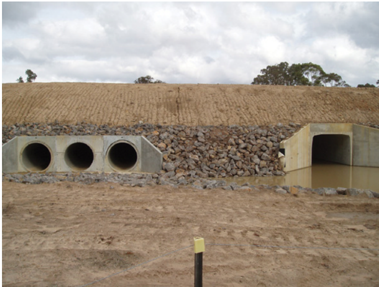
Figure 9.2 Due to relatively minor modifications, mistakes or misunderstandings during design and construction, the three drainage culverts remain dry during rainfall events and the wildlife underpass is flooded. Source: Photograph by and reproduced with permission of Scott Watson.
