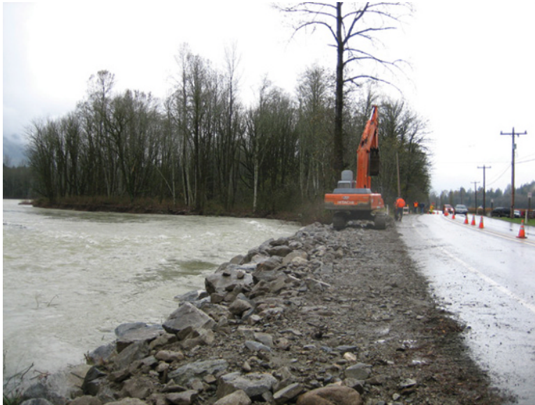
Figure 44.3 The use of large rock (or rip rap) is a common approach to protecting road infrastructure from damaging flows, here used as an emergency response along Highway 20 on the Skagit River, Washington, USA. Source: Photograph by Paul J. Wagner.
