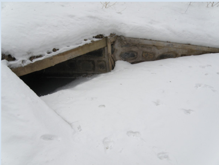
Figure 57.2 Tracks of Siberian weasel through a culvert under the Ring Changbai Mountain Scenic Highway. Source: Photograph by Yun Wang.
