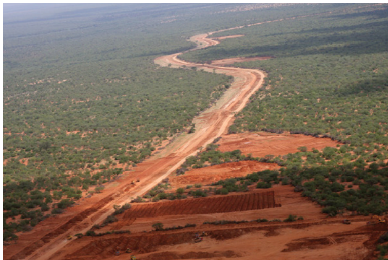
Figure 56.4 Footprint of construction crews building the road north of Isiolo in Kenya. Source: Photograph by M.E. Gadd.
