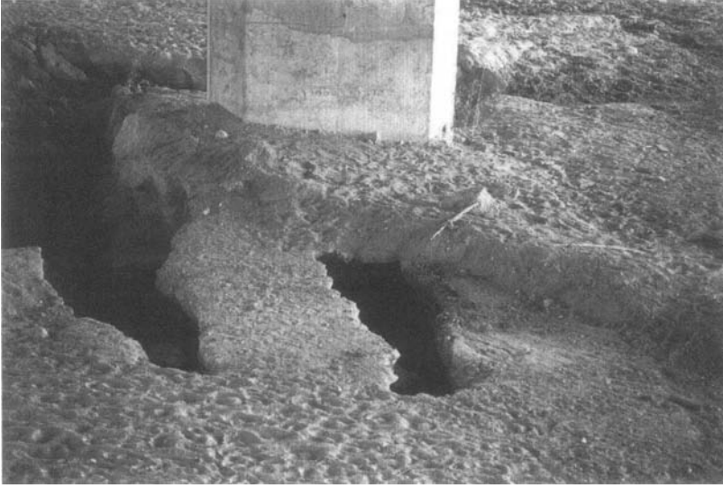
Figure 10-9. Scour of a bridge foundation caused by soil running water
