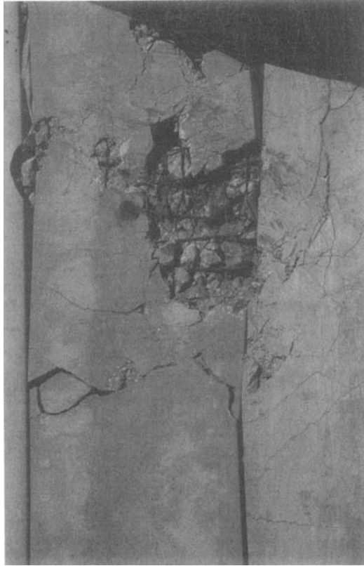
Figure 10-21. Broken concrete element due to a lorry collision (cause C-D2)
