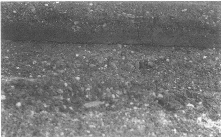
Figure 10-22. Severe scaling of concrete surface due to freeze/thaw cycles (cause C-E5)
