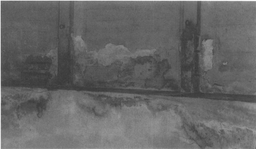
Figure 4-7. Lack of waterproofing
