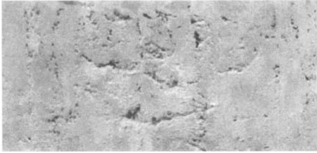
Figure 5-15. Plastic settlement cracking
