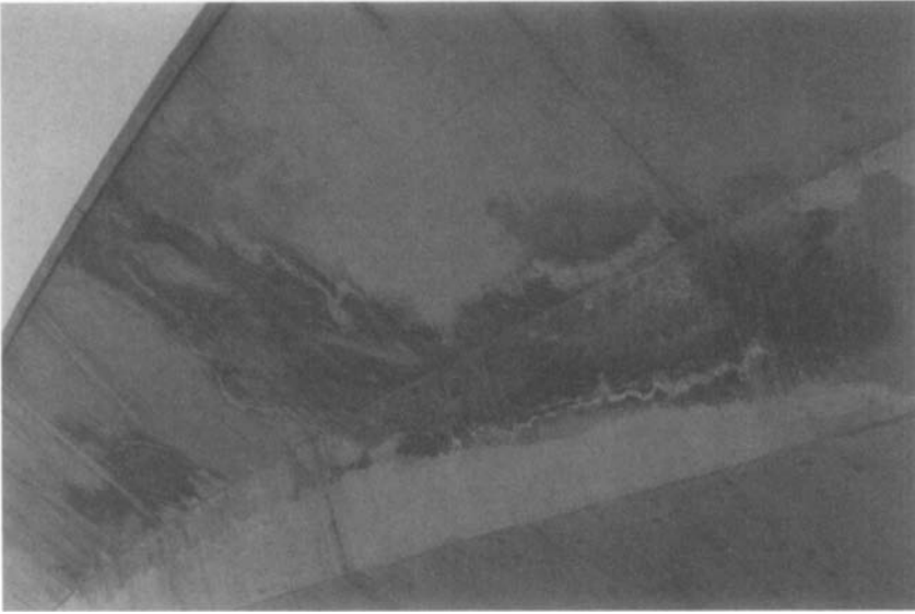
Figure 10-19. Drainage directly over concrete due to a design error in the drainage system (cause C-A24)
