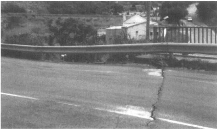
Figure 5-17. Settlement of the approach fill
