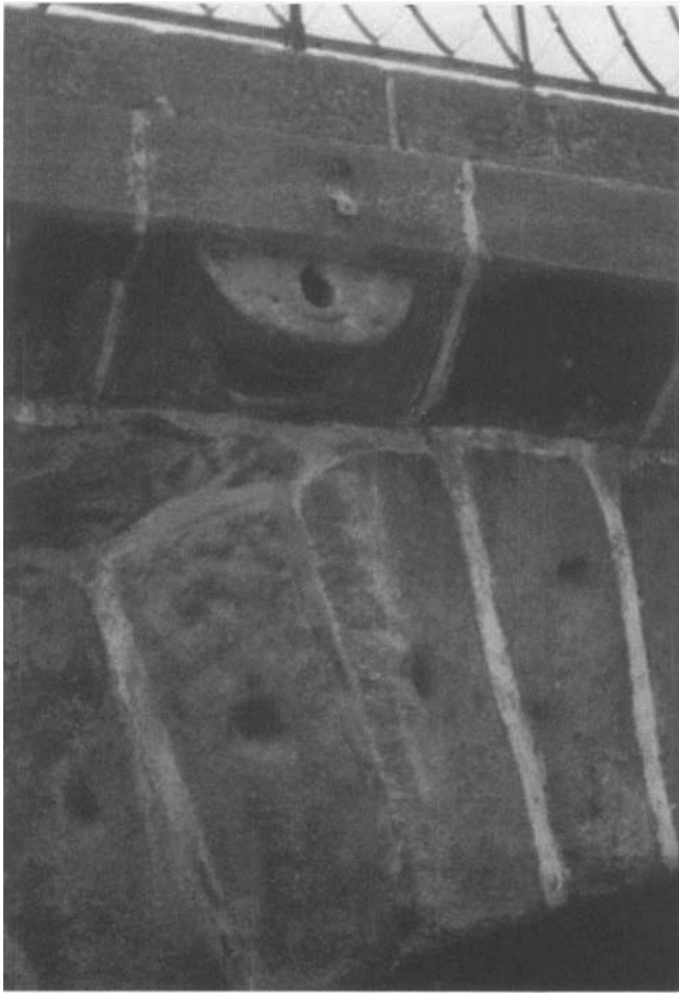
Figure 1-2. Detail of the drainage system of a Roman bridge in Chaves, Portugal
