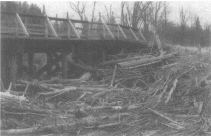
Figure 10-20. Stream obstructed by debris and siltation after a flood (cause C-C4)
