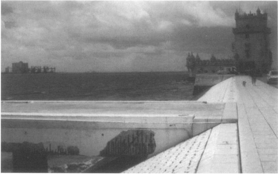
Figure 1-6. 50-year-old deteriorated quay (in foreground) and the 500-year-old well-preserved Belém Tower (in background) in Lisbon, Portugal
