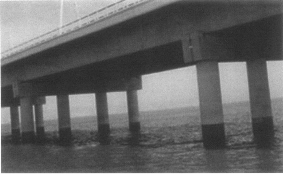
Figure 4-5. Steel elements in a marine environment, South viaduct, Alcochete, Portugal
