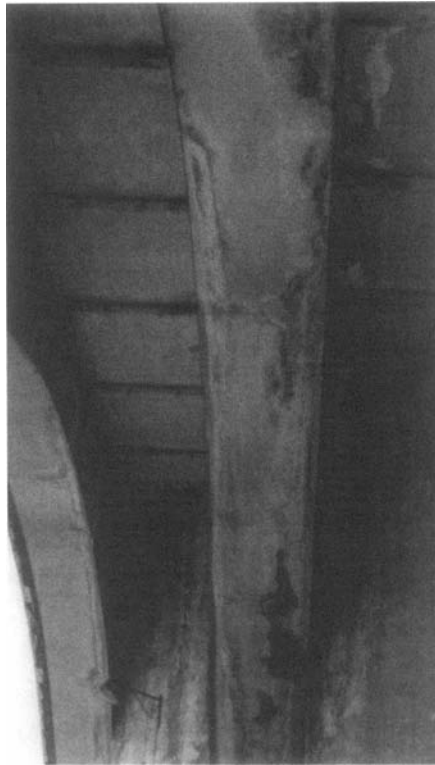
Figure 4-2. Degradation in a 60-year-old bridge
