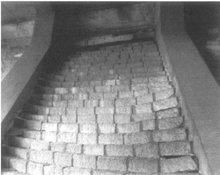
Figure 5-19. Deterioration of earth fill slopes
