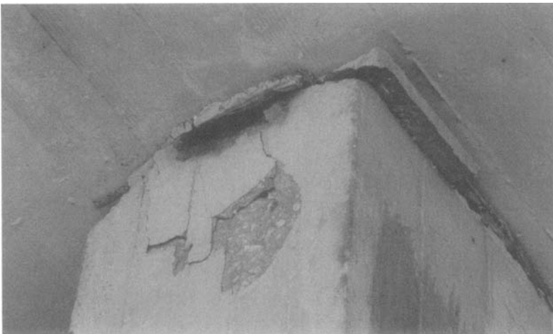
Figure 2-6. Deterioration of a bearing
