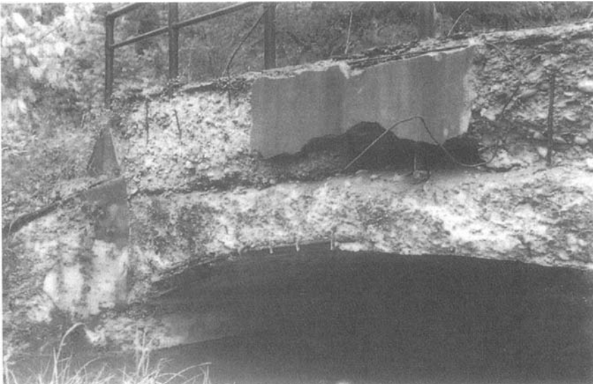
Figure 6-3. Exterior surface of a concrete deck suffering from highly advanced disintegration
