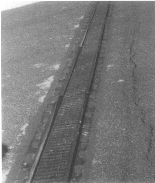
Figure 10-26. Settlement of the approach slab due to an increase in the maximum allowed load (cause C-I3)
