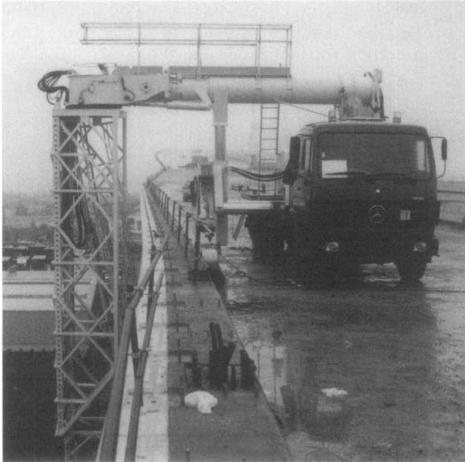
Figure 4-12. Mobile scaffold truck
