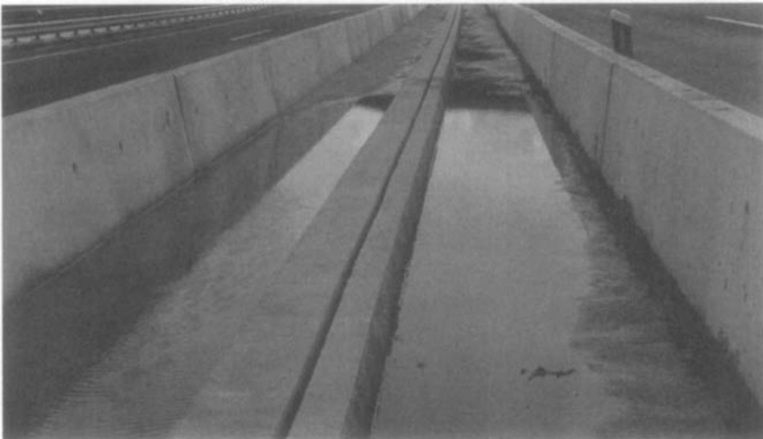
Figure 10-17. Defect A-H1: Deposit of water
