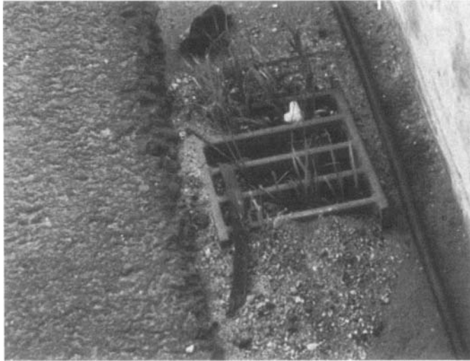
Figure 5-22. Deficient placement of deck drain
