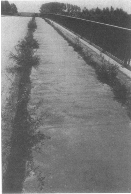
Figure 10-25. Noxious vegetation in the sidewalks borders due to lack of maintenance (cause C-H8)
