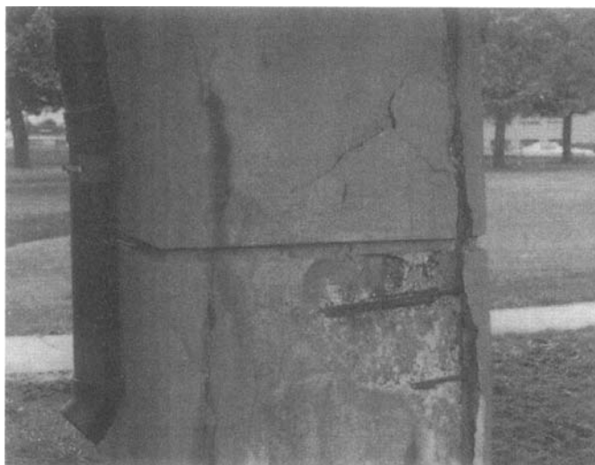
Figure 6-5. Defect in column rated as MCR 2 (serious delamination and spalling in more than 15% of the surface, with reinforcement in full view) and PCR 4 (the deterioration results in a 5% loss in the load-bearing capacity)
