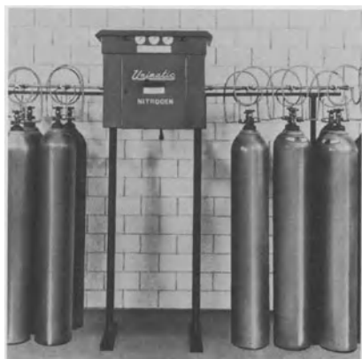
A stand-mounted nitrogen manifold with “in use” and reserve cylinder banks.
