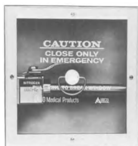
Recessed valve box with single nitrogen valve.
