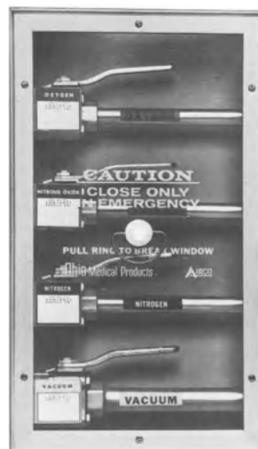
Recessed valve box with four valves.
