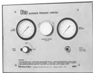
Nitrogen pressure control cabinet.
