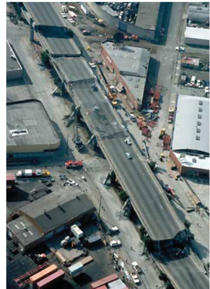
A double-deck freeway in Oakland, California, collapsed during the Loma Prieta earthquake on October 17, 1989, crushing the cars on the lower deck and killing 42 people.
