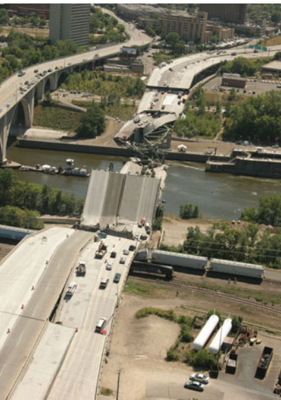
The I-35W Bridge in Minneapolis, Minnesota, collapsed into the Mississippi River and riverbanks on August 1, 2007, killing 13 people and injuring 145.
