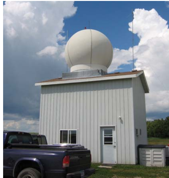
FIGURE 4-9 Weather radar installation. Shown is a 5-cm (2-in.) wavelength facility located in Stanley, North Dakota. The antenna and pedestal are housed within a fiberglass radome that allows operation to continue even in strong winds. The building is air-conditioned to provide comfort to the electronics and project staff. An auxiliary power unit provides power when commercial service fails
