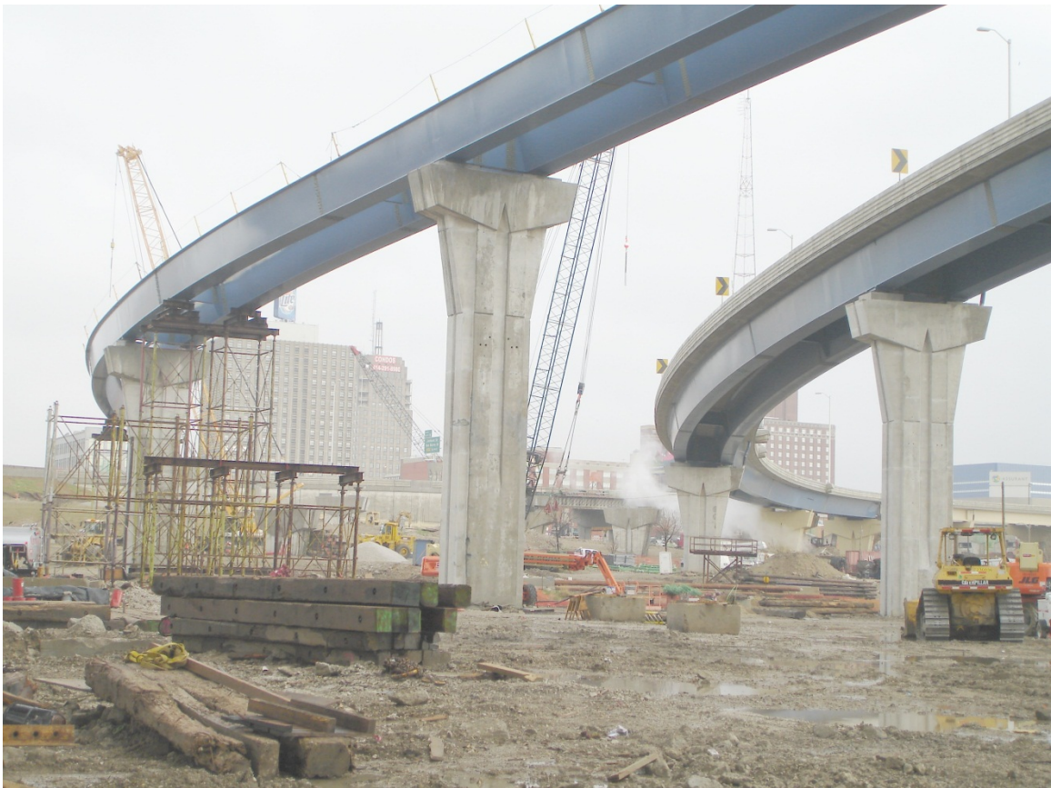
Figure 4.37. ETCCR 15, Unit B-40-1122 of the Marquette Interchange, Milwaukee, WI (courtesy of Tony Shkurti, HNTB Corporation).
