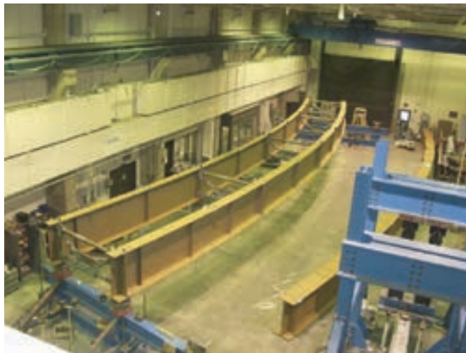
Figure 3-4. FHWA Test Bridge (EISCR1) during the steel erection, with cross-frames attached between girders G2 and G3 (Jung, 2006; Jung and White, 2008).
