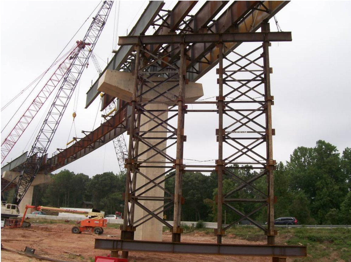
Figure 4.35. EICCR4, Ramp GG John F. Kennedy Memorial Highway, I-95 Express Toll Lanes and I-695 Interchange, Baltimore Co., MD (courtesy of R. Cisneros, High Steel Structures, Inc.).
