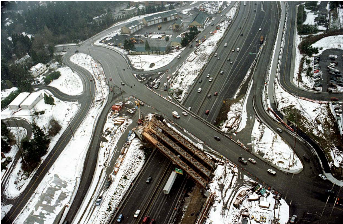
Figure 4.22. ETSSS 2, Sylvan Bridge over Sunset Highway, Multnomah Co., OR (courtesy of Homoz Seradj, Oregon DOT).
