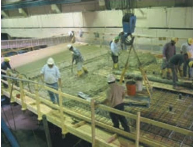
Figure 3-6. FHWA Test Bridge placement of the slab concrete (Jung, 2006; Jung and White, 2008).
