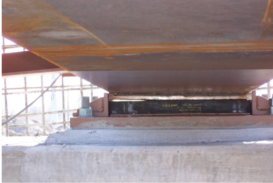
Figure 4.24. EICSS1, Steel Overpass Sunnyside Road I.C. (I-15B) over I-15, Bonneville Co. ID, gap at sole plate under steel dead load; the girders rotated during the deck placement such that full contact was established with the elastomeric pads (courtesy of Matt Farrar, ITD).
