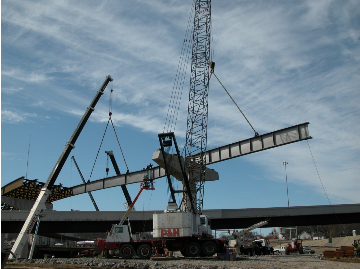
Figure 4.31. EICCR22a, Bridge No. 12 Ramp B over I-40, Robertson Avenue Project, Davidson Co., TN.
