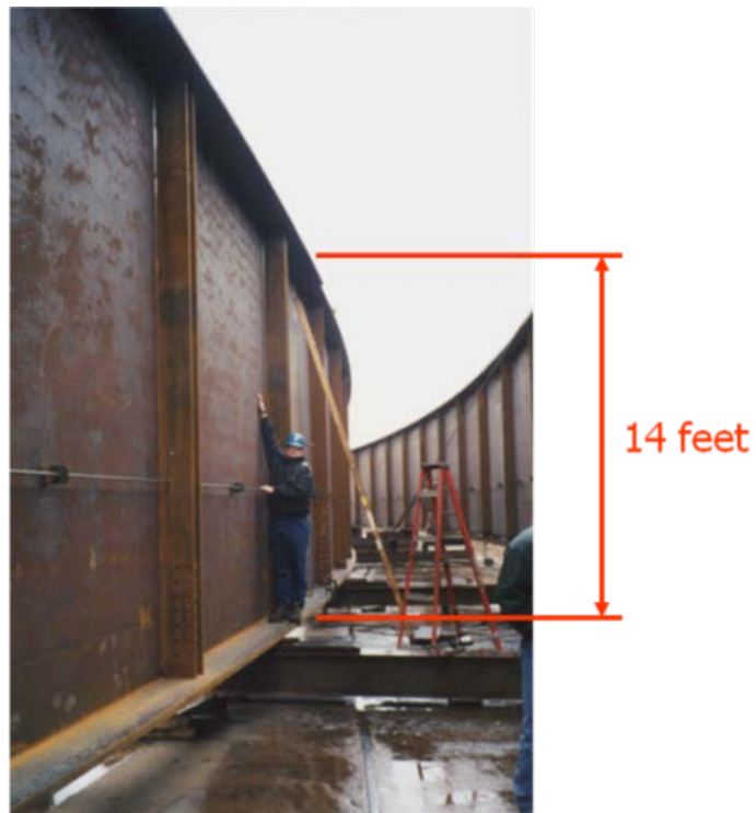
Figure 4.33. EICCR11, Ford City Bridge, Ford City, PA, girder depth and spacing (Chavel, 2008).
