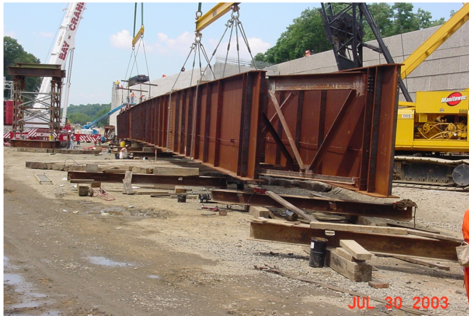
Figure 4.20. EISS6, Bridge on Westchester Co., NY (courtesy of R. Cisneros, High Steel Structures, Inc.).
