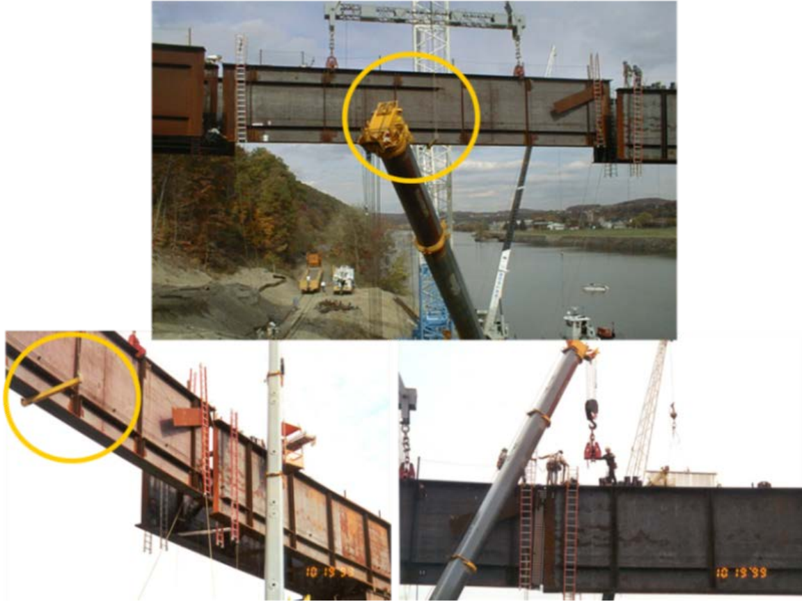
Figure 4.34. EICCR11, Ford City Bridge, Ford City, PA, installation of drop-in segment (Chavel, 2008).
