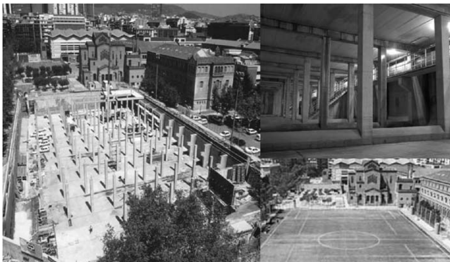
Fig. 4.9. Retention tank located at Escola Industrial de Barcelona
