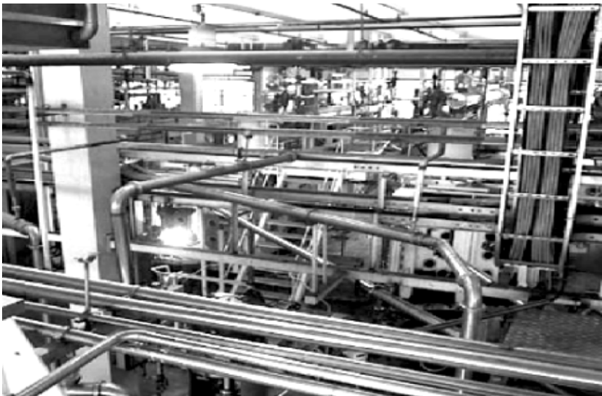
FIGURE 8. Example of inappropriate piping.
