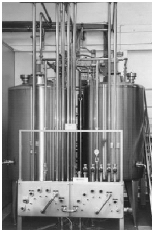
FIGURE 2. CIP system with two tanks. (by courtesy of Norda spa Parma).
